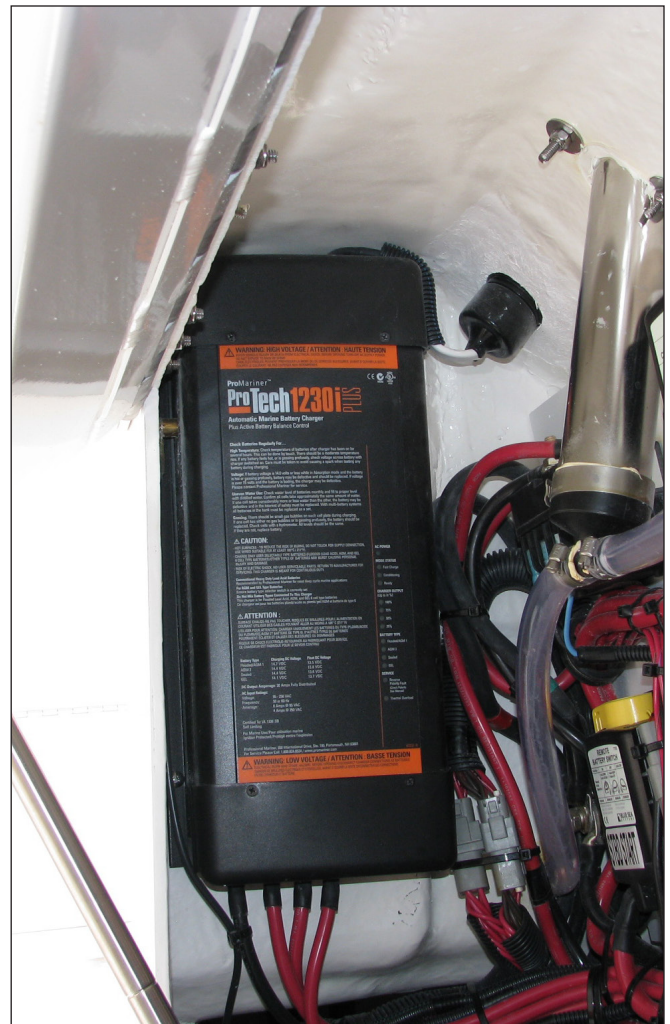
Typical Battery Charger
