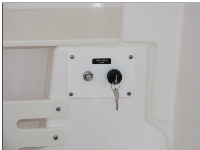
Waste System Pump Out Switch Panel
