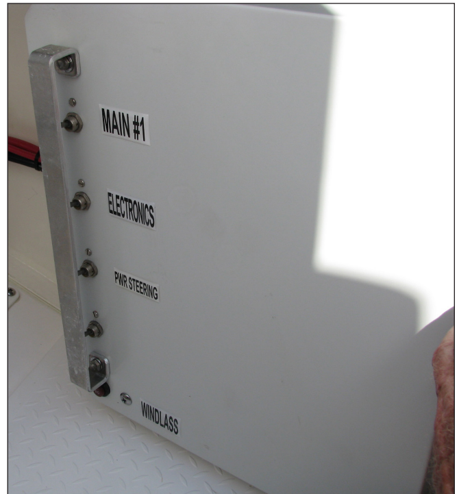
325 Center Console Main Circuit Breakers
