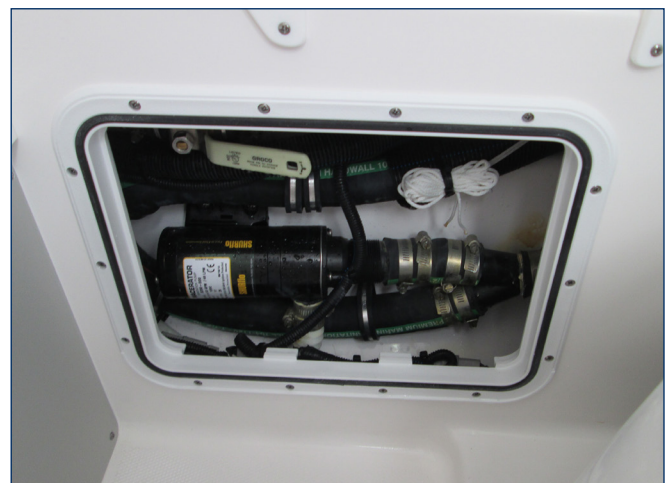
Macerator Access Hatch
