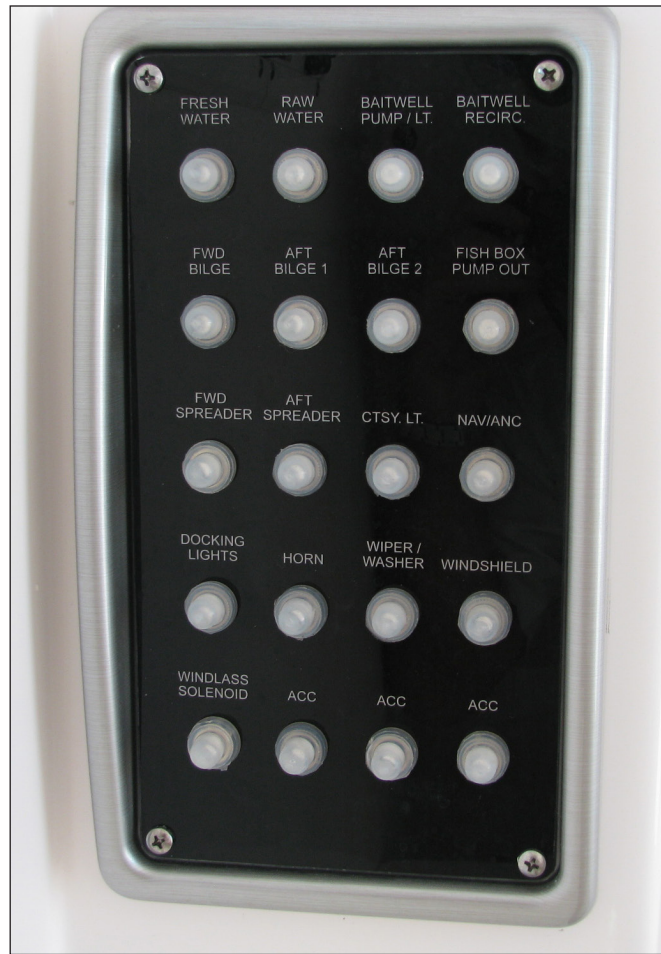
Head Compartment DC Circuit Breaker Panel
