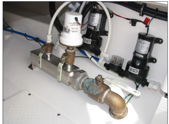
325 Center Console Seawater Supply Manifold and Seacocks Baitwell Supply Pump and Raw Water Pressure Pump
