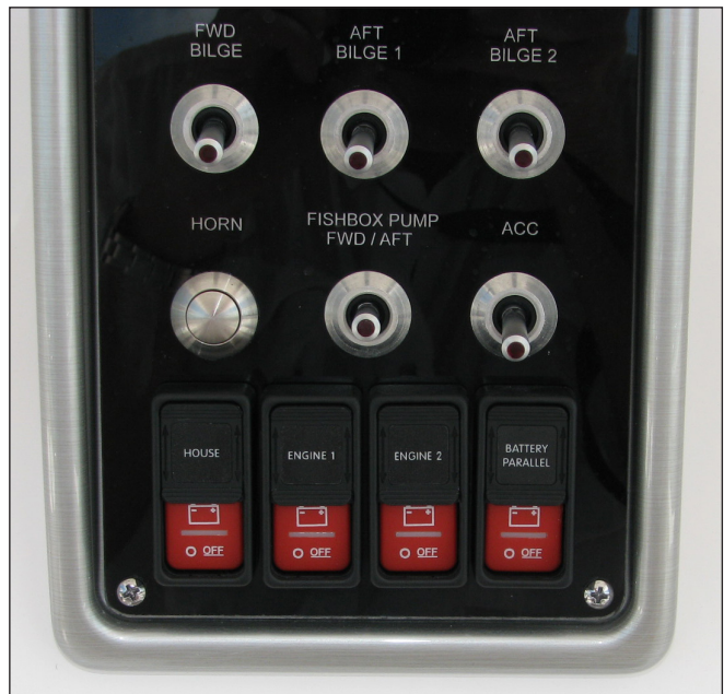
Remote Battery Switches in OFF Position
