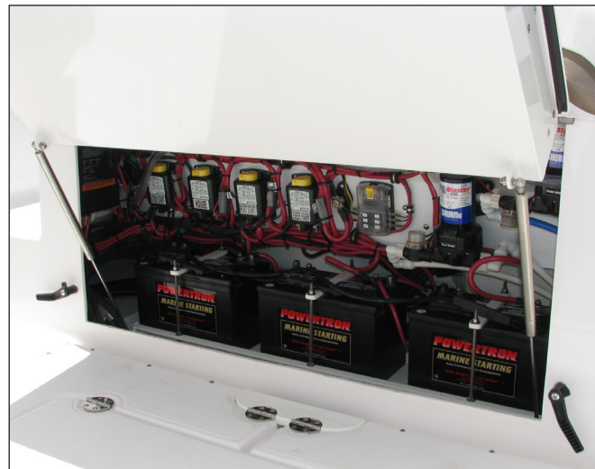
255/275/295 Center Console System Compartment and Batteries
