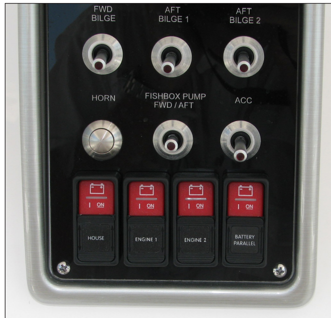
Remote Battery Switches in ON Position
