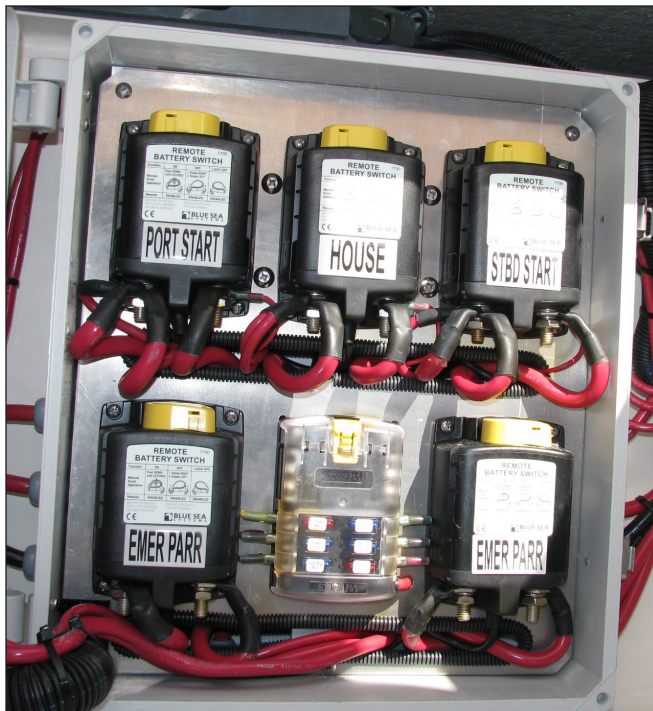
325 Center Console Battery and Emergency Parallel Switches
