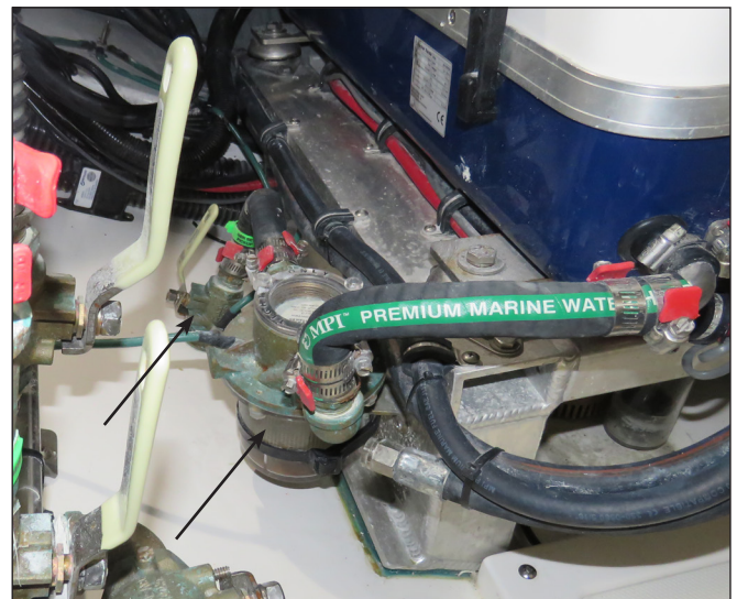
Generator Sea Strainer & Seacock Valve
