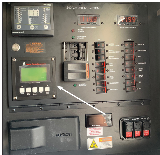
Generator Control Panel
