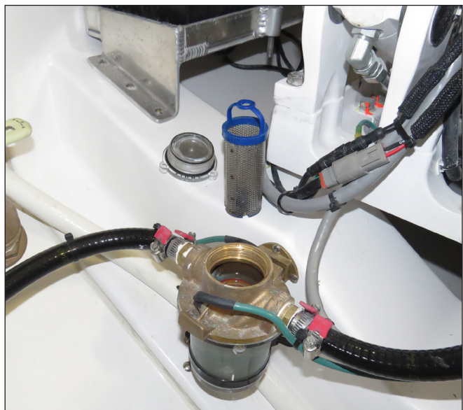
Generator, HVAC, & SeaKeeper Sea Strainer Screen & Cap
