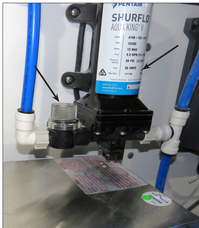
Fresh Water Pump & Strainer
