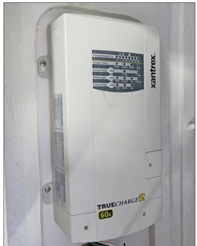
Typical House Battery Charger
