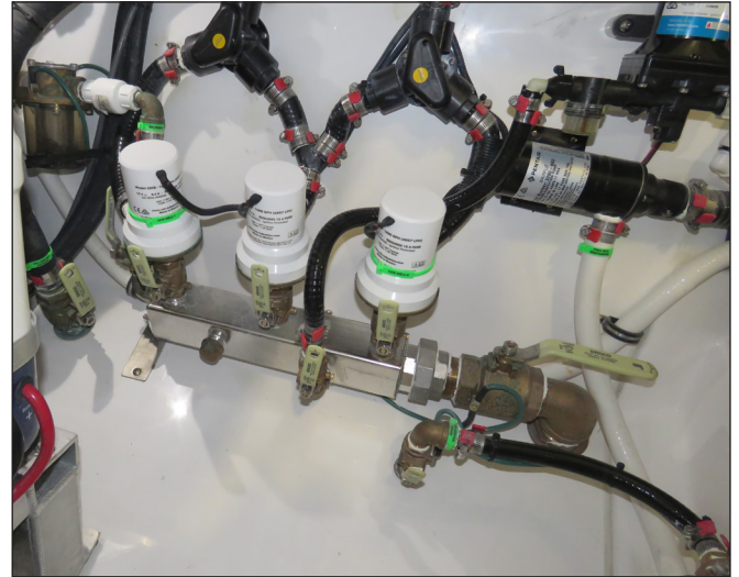
Raw Water Manifold, Baitwell Pumps, Baitwell Y-Valves & Supply Valves
