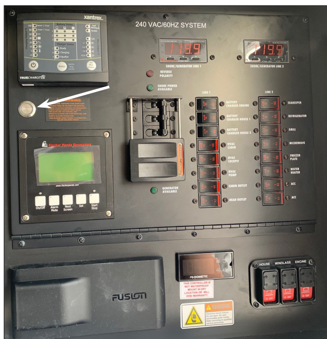
Bilge Blower Switch
