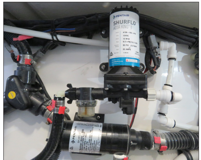
Raw Water Pressure Pump & Sea Strainer
