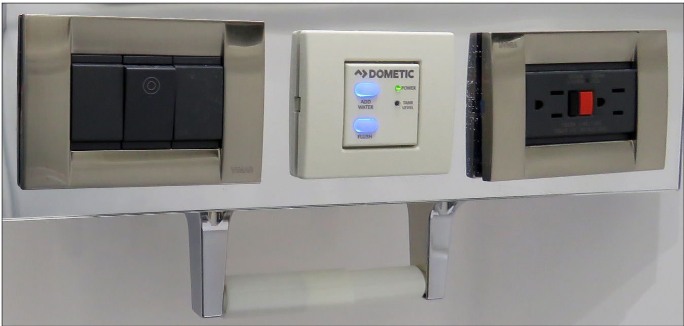
Head Compartment Light Switches, GFI Outlet & Marine Toilet Control Panel
