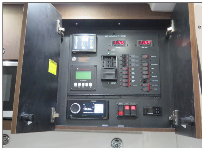
Cabin Electrical Panel
