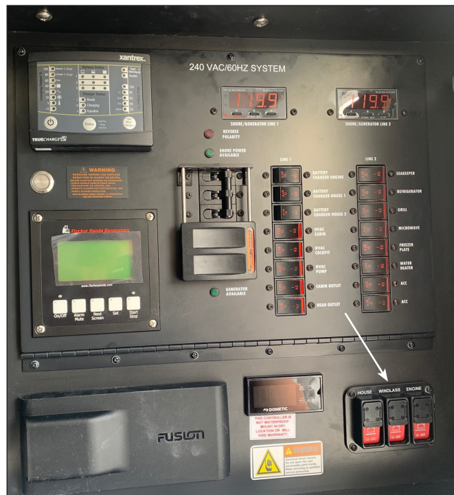
Battery Switch Panel in Cabin AC Panel
