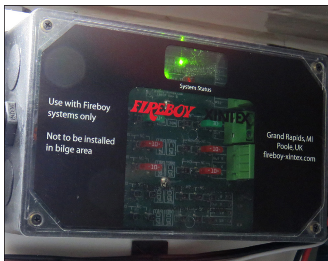
System Status Panel & Fuses
