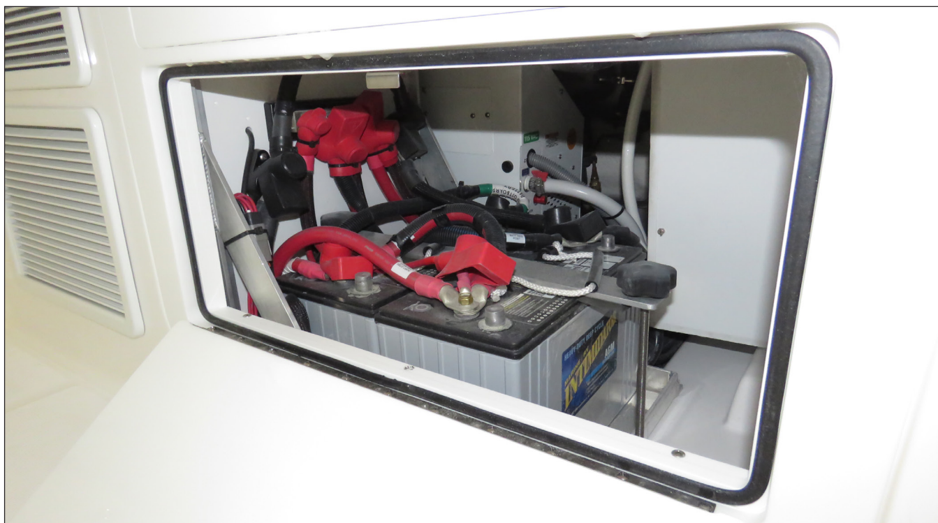
House Batteries in Mezzanine Compartment
