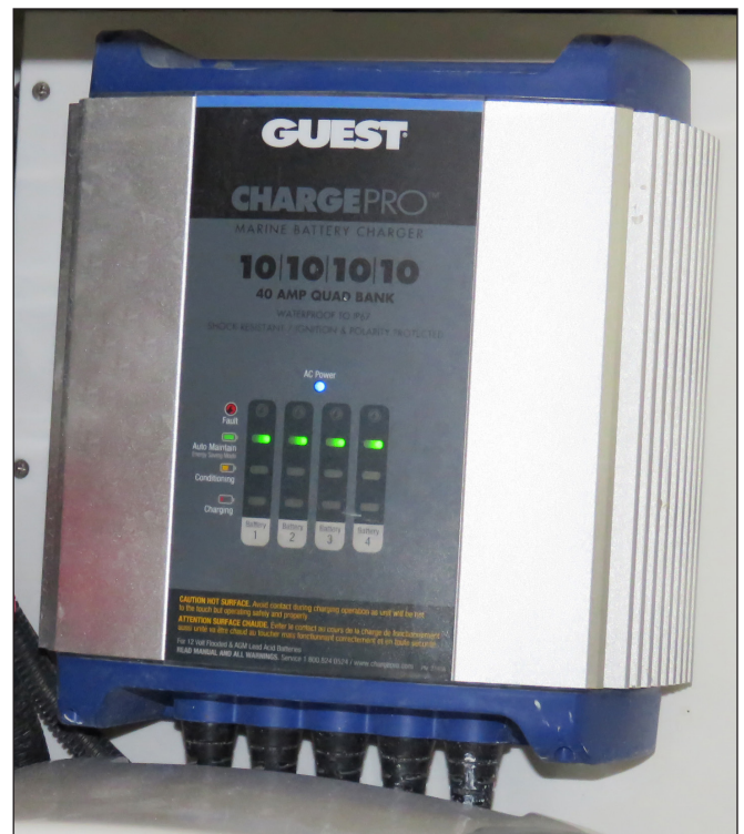
Charger for the Engine Batteries in Aft Systems Compartment
