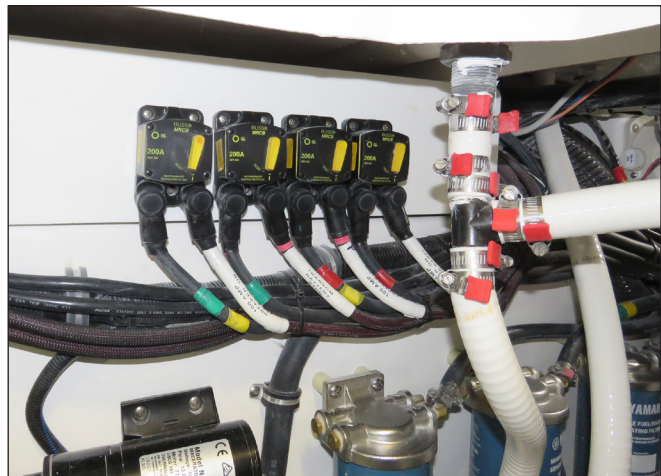
Helm Master Main Circuit Breakers
