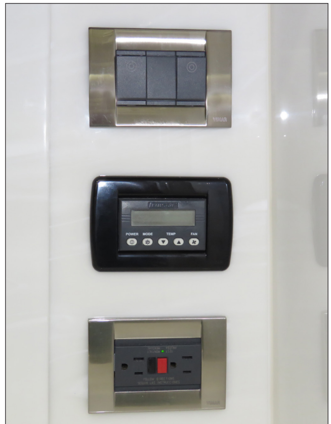
Cabin Switch Panel, HVAC Control Panel & GFI Outlet
