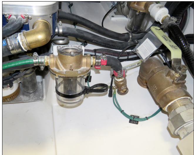
Typical Generator Raw Water Seacock & Strainer
