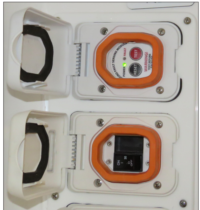
ELCI Panel & Inlet Main Breaker
