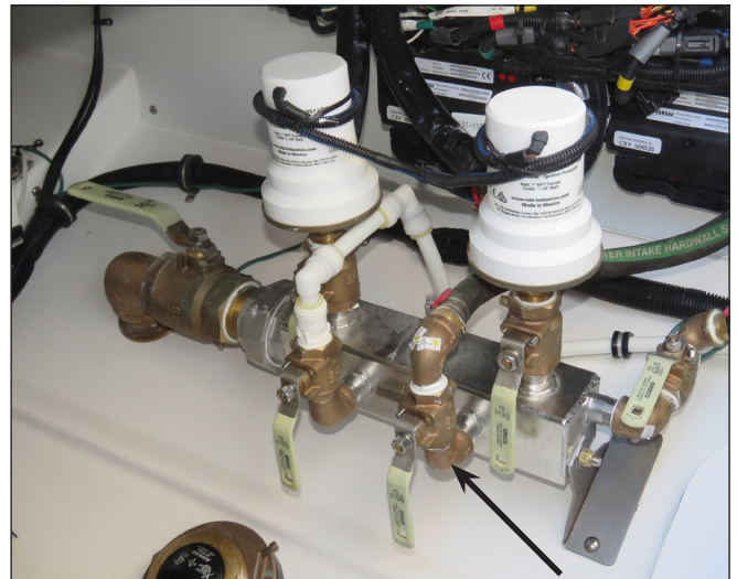
Air Conditioner Pump Supply Valve
