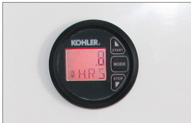
Cabin Generator Control Switch & Monitor
