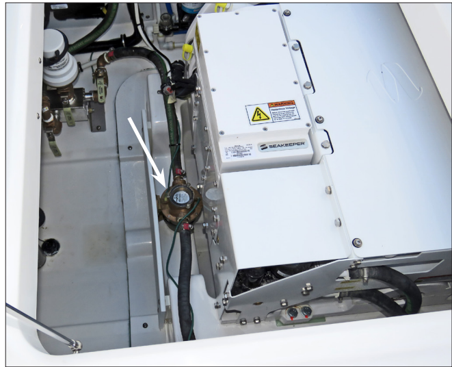
SeaKeeper System Sea Strainer
