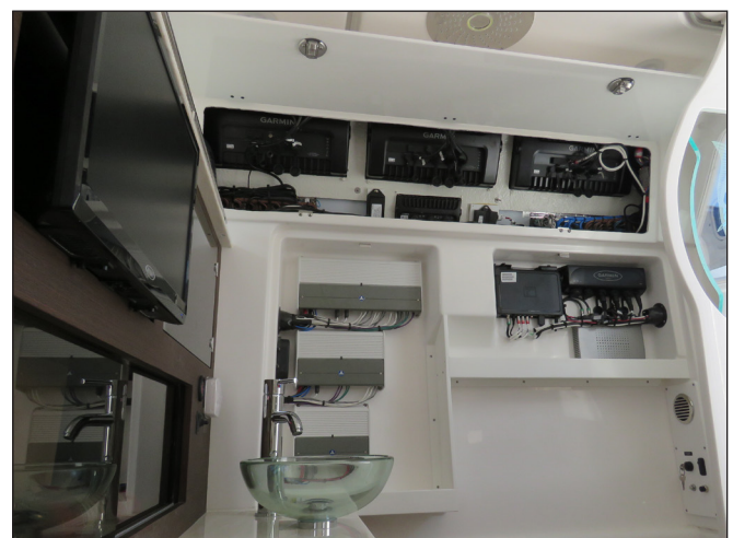
Electronics Access in Rear Cabin Bulkhead
