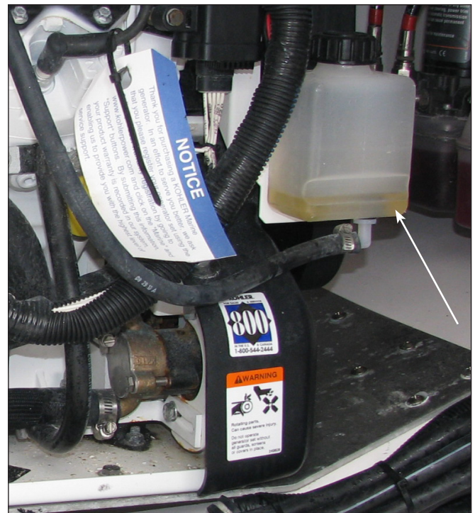
Typical Generator Coolant Recovery Tank
