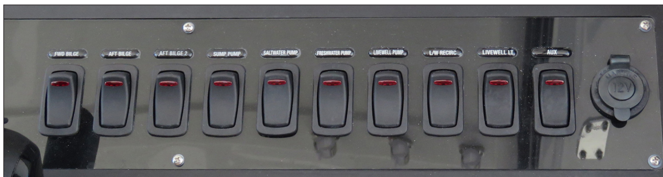
Starboard Helm Accessory Switch Panel
