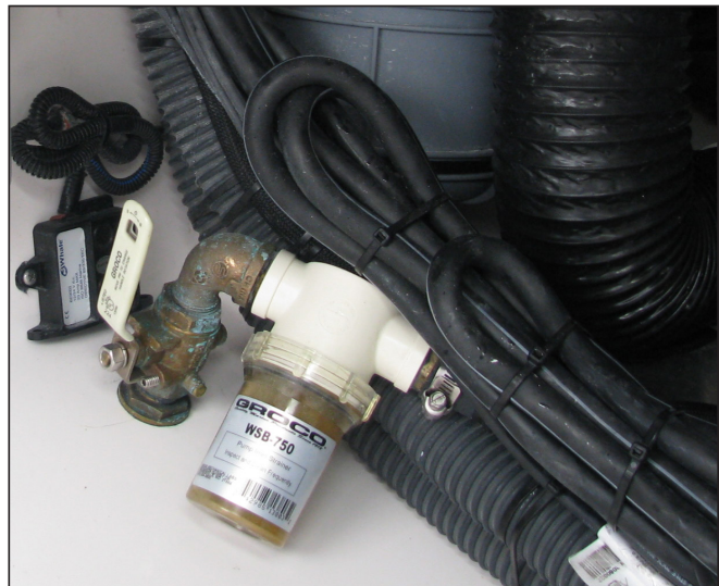
Typical Generator Raw Water Seacock & Strainer
