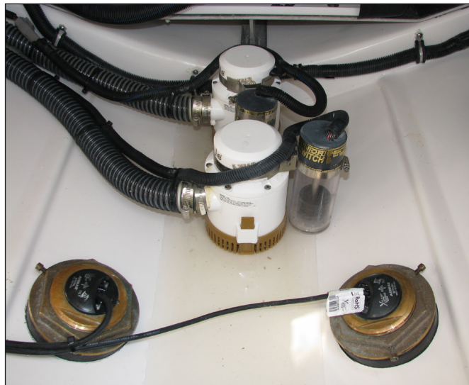
typical Stern Bilge Pumps & Automatic Switches
