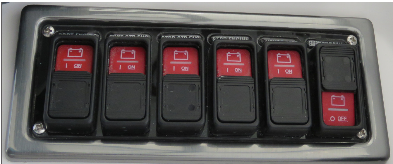
Battery Switch Panel at Helm
