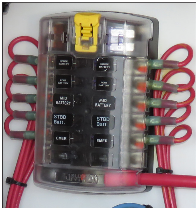
Remote Battery Switch Fuse Panel
