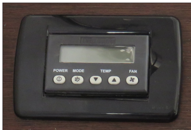
Air Conditioner Control Panel
