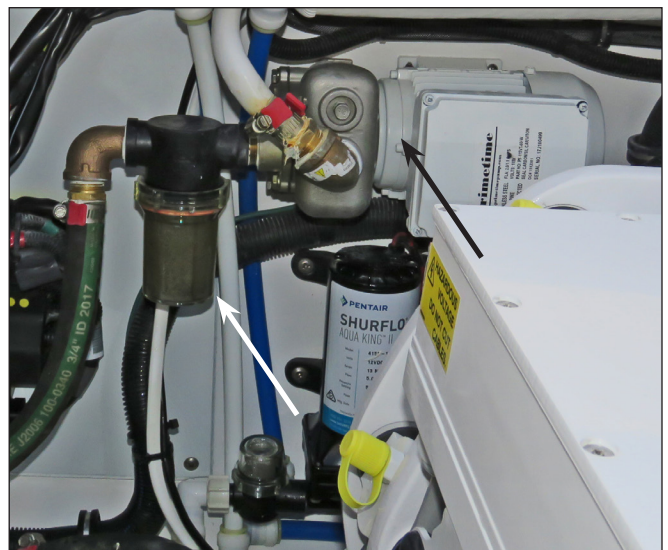
Air Conditioner Seawater Pump & Strainer
