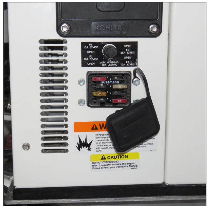
Typical Generator Fuse Panel
