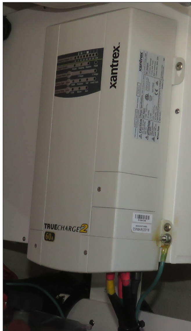
Typical Battery Charger
