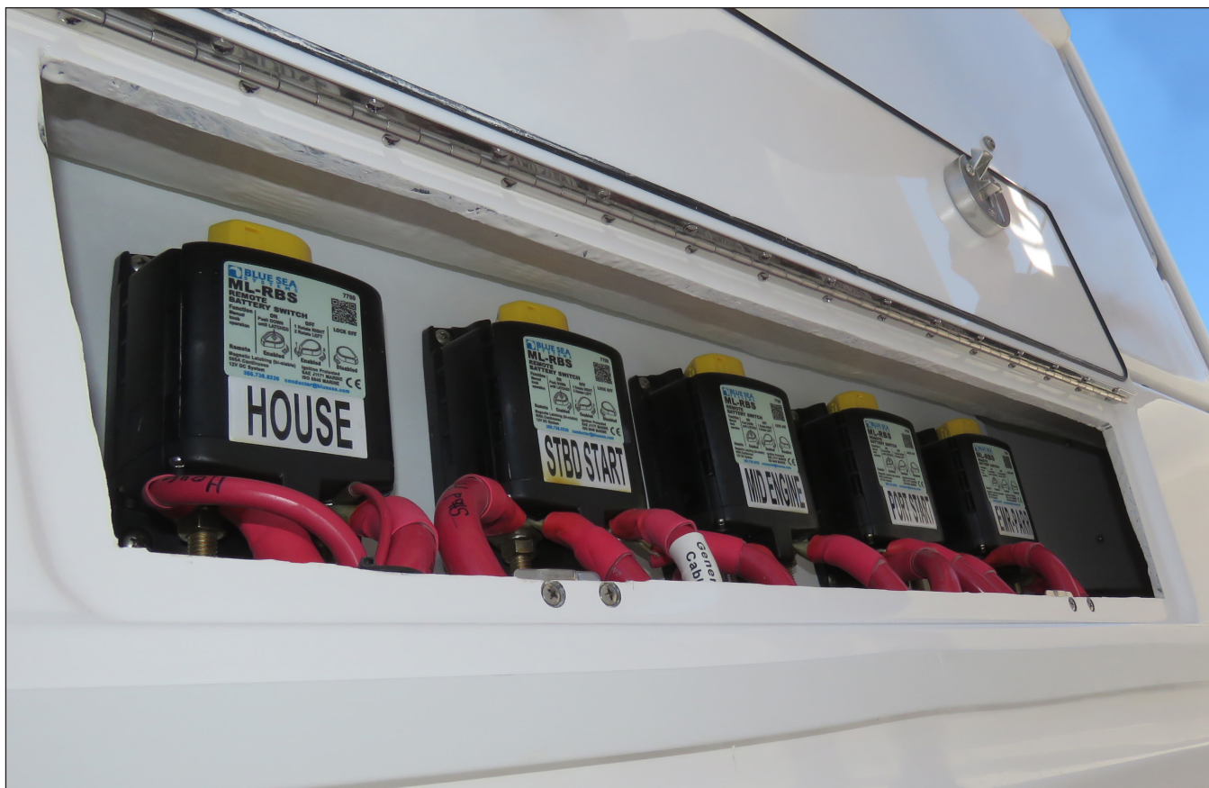
Quad Engine Remote Battery Switches & Emergency Parallel Switch
