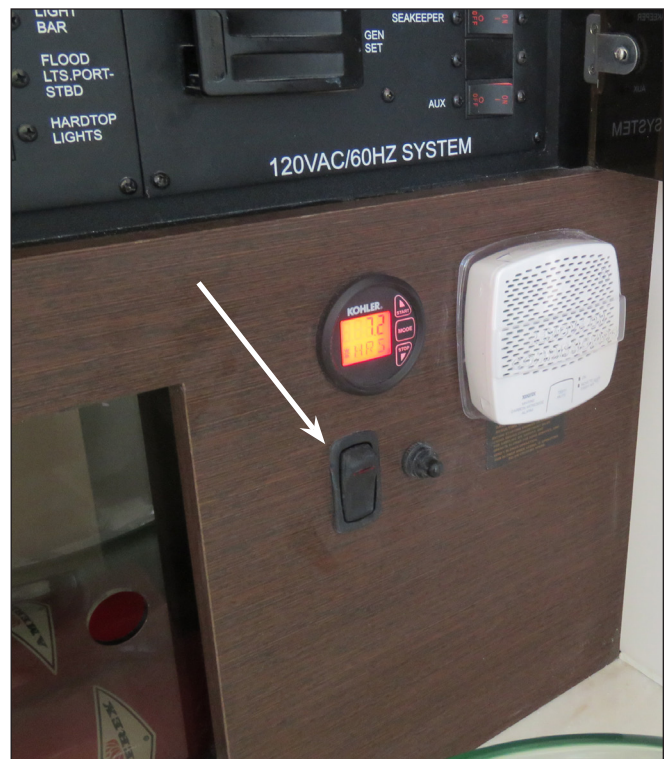
Cabin Bilge Blower Switch
