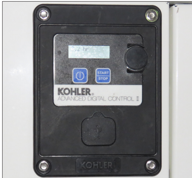
Generator Onboard Control Switch & Engine Monitor,
