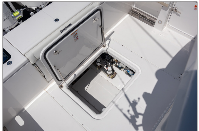
Mechanical Systems Compartment Hatch
