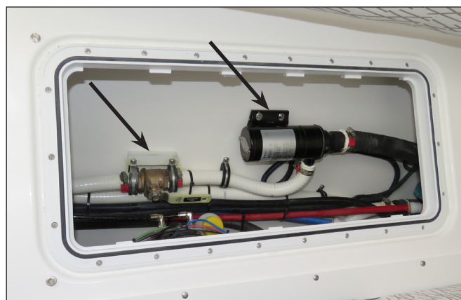
Overboard Macerator Pump & Thru-Hull Valve
