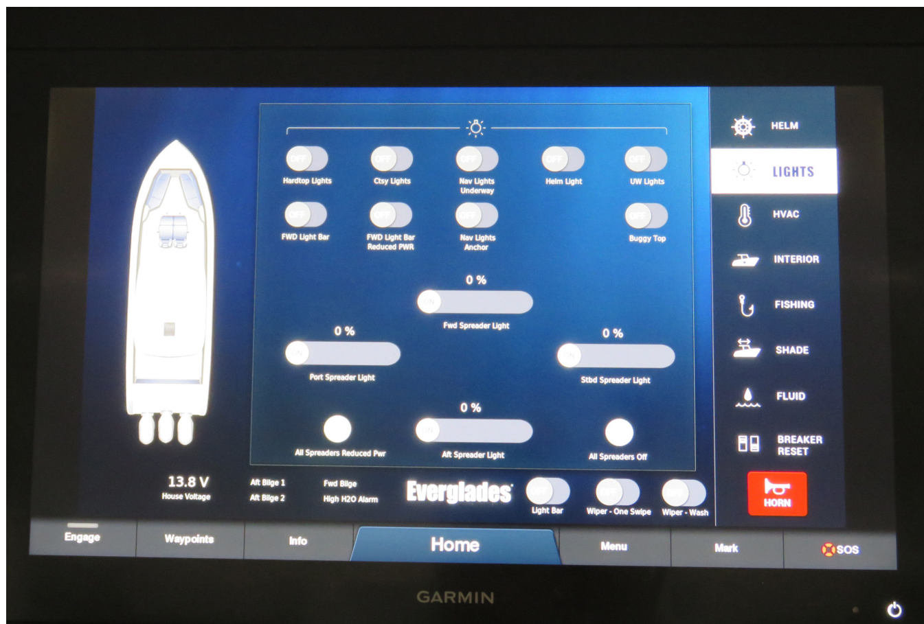
Typical Switches in the Lights Switch Touch Screen Display
