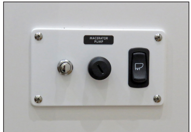
Toilet & Overboard Discharge Control Panel
