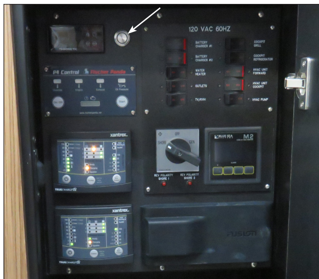
Bilge Blower Switch
