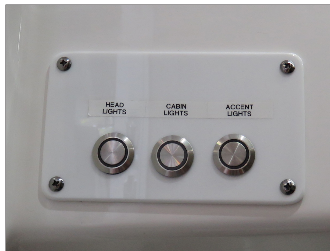
Cabin Switch Panel
