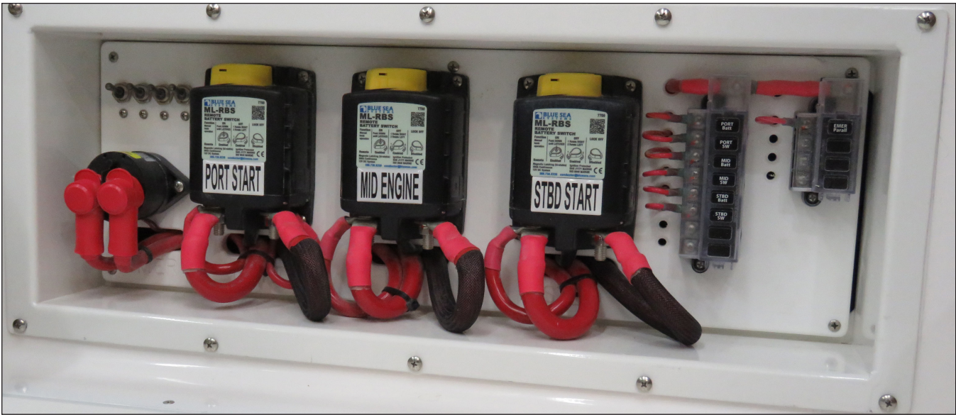
Engine Battery switches & Battery Parallel Switch, Fuse Panels for Remote Battery & Parallel Switches Located Behind the Starboard Cabin V-Berth Backrest Cushion
