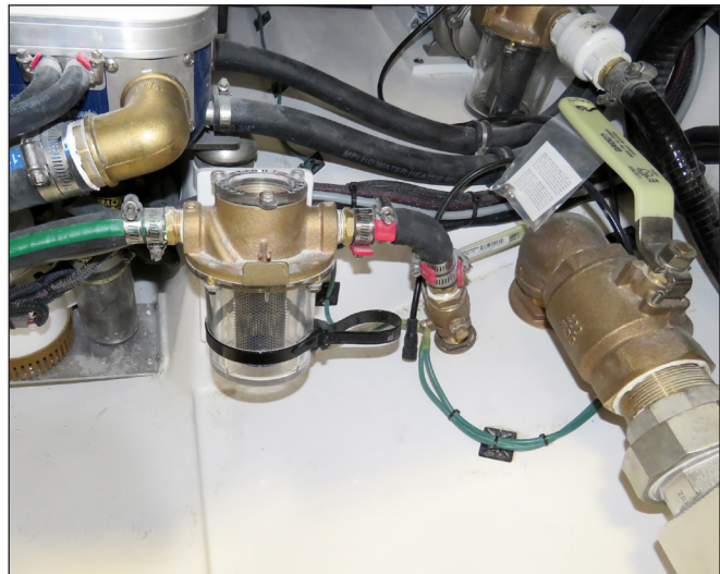
Typical Generator Raw Water Seacock & Strainer
