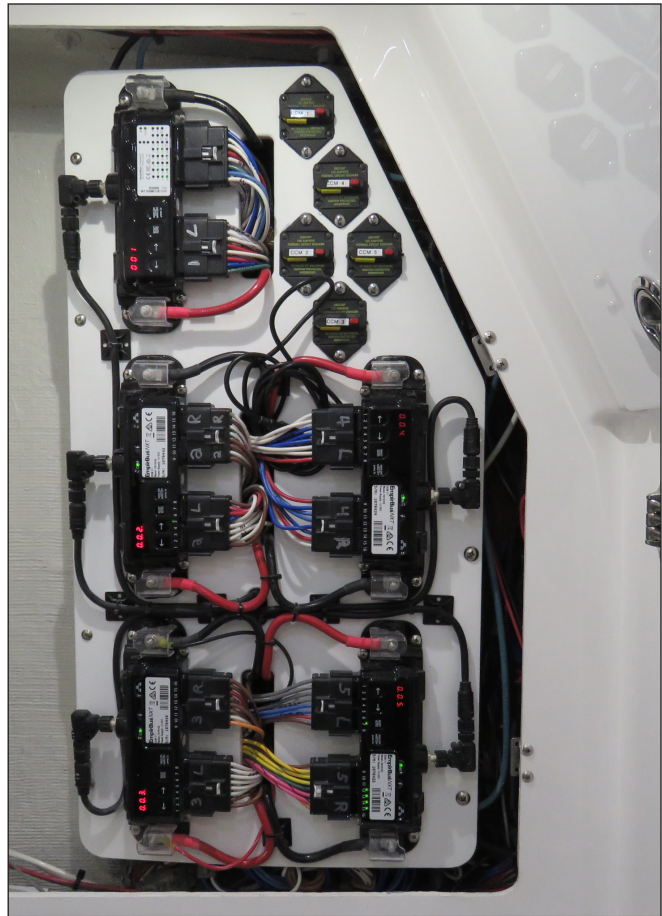
Digital Switch Control Modules & Main Circuit Breakers
