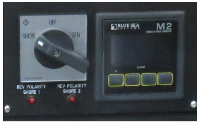
SHORE/OFF/GENERATOR Switch & Multimeter
