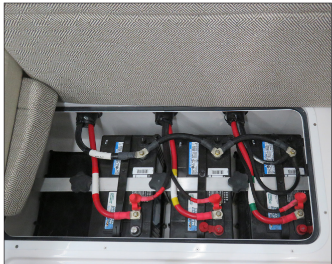
Engine Start Batteries Below Starboard V-Berth Cushion
