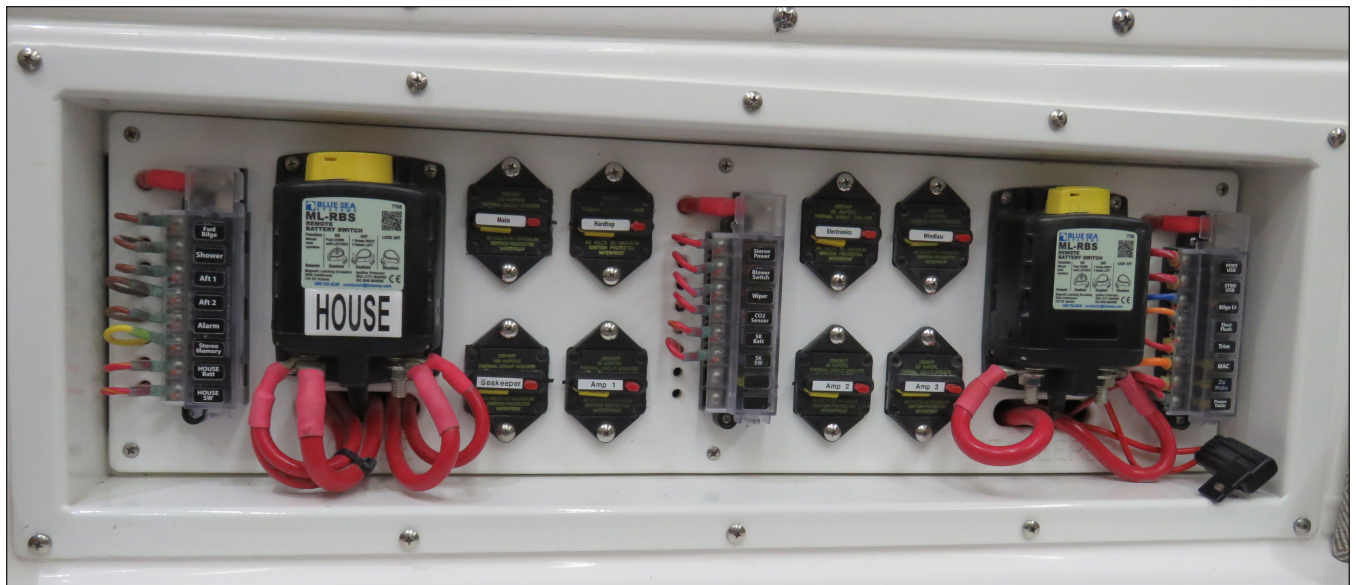
House Battery Switch, SeaKeeper Switch, Continuous Power Fuse Panels & Main Circuit Breakers Located Behind the Port Cabin V-Berth Backrest Cushion
