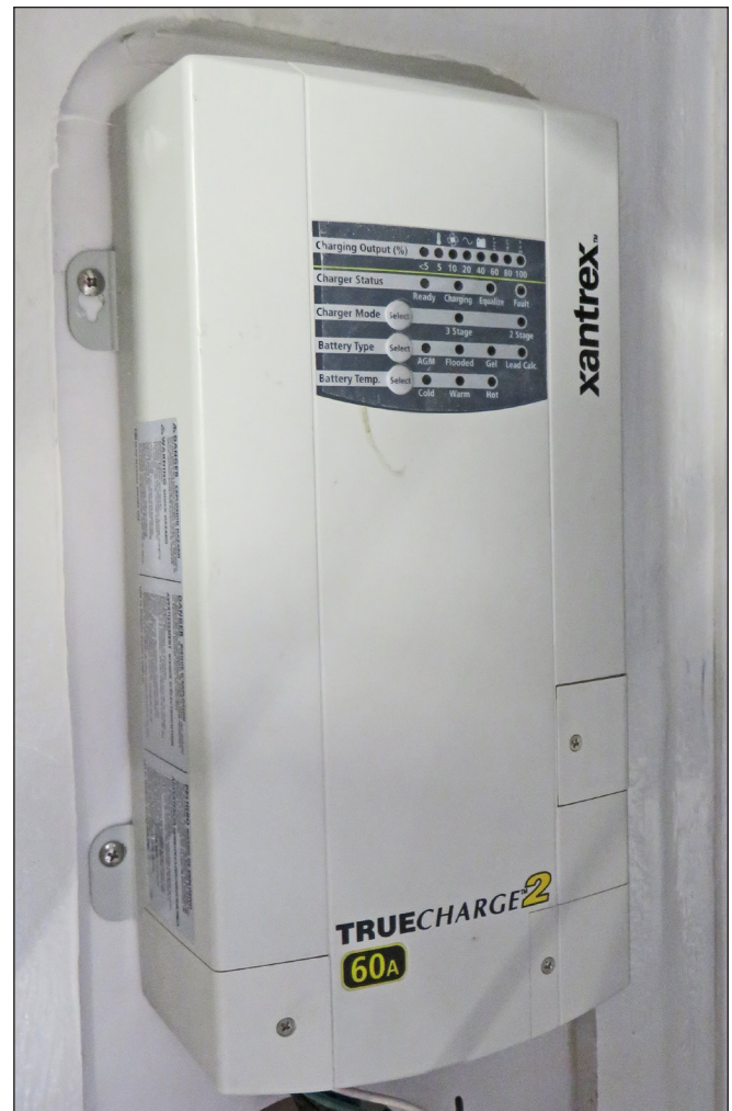
Typical Battery Charger
