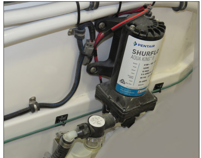
Raw Water Pressure Pump & Sea Strainer
