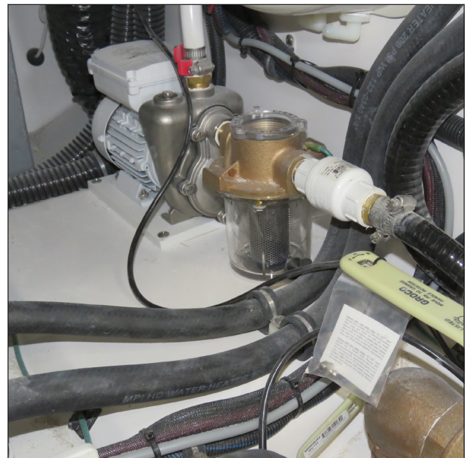
Air Conditioning Pump & Sea Strainer
