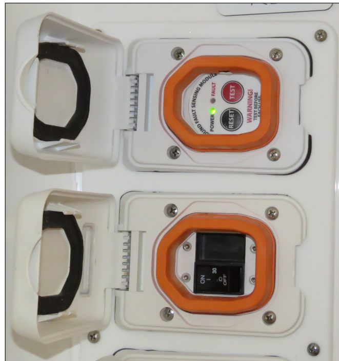
ELCI Panel & Inlet Main Breaker
