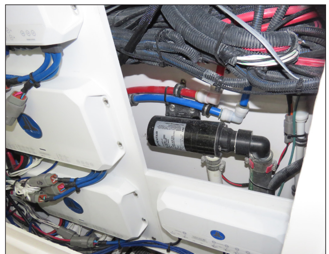
Overboard Macerator Discharge Pump
