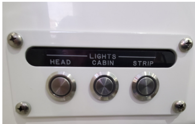
Cabin Light Switch Panel
