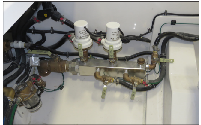
Raw Water Manifold, Port & Starboard Livewell Pumps, Raw Water Pump Connection, HVAC & SeaKeeper Pump Connections & Ball Valves
