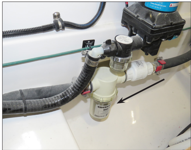
SeaKeeper System Sea Strainer
