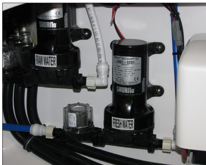
Fresh Water Pump and Strainer
