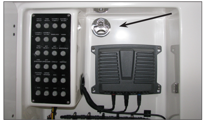
Electronics Modules, Accessory Circuit Breaker Panel and Opening Helm Latch
