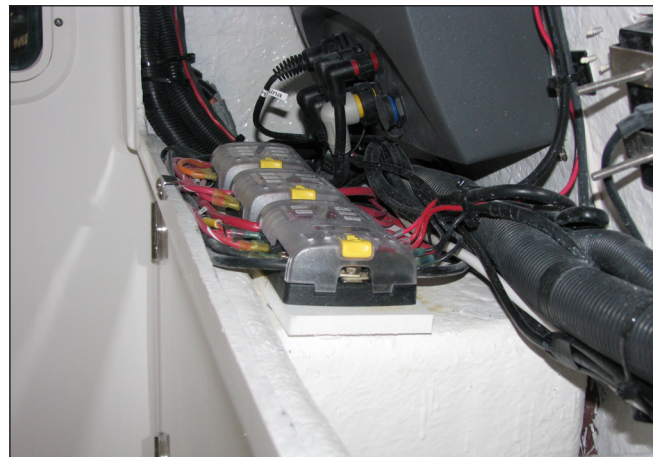
Fuse Panels Behind Helm
