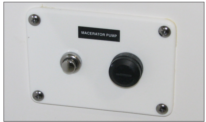
Typical Waste Discharge and Lockout Switches
