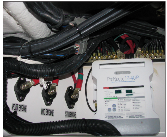
Typical Battery Charger in Systems Compartment
