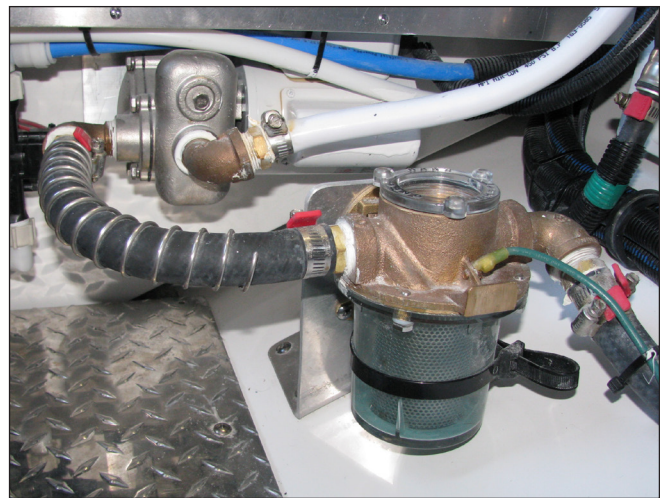
Air Conditioner Seawater Pump & Strainer
