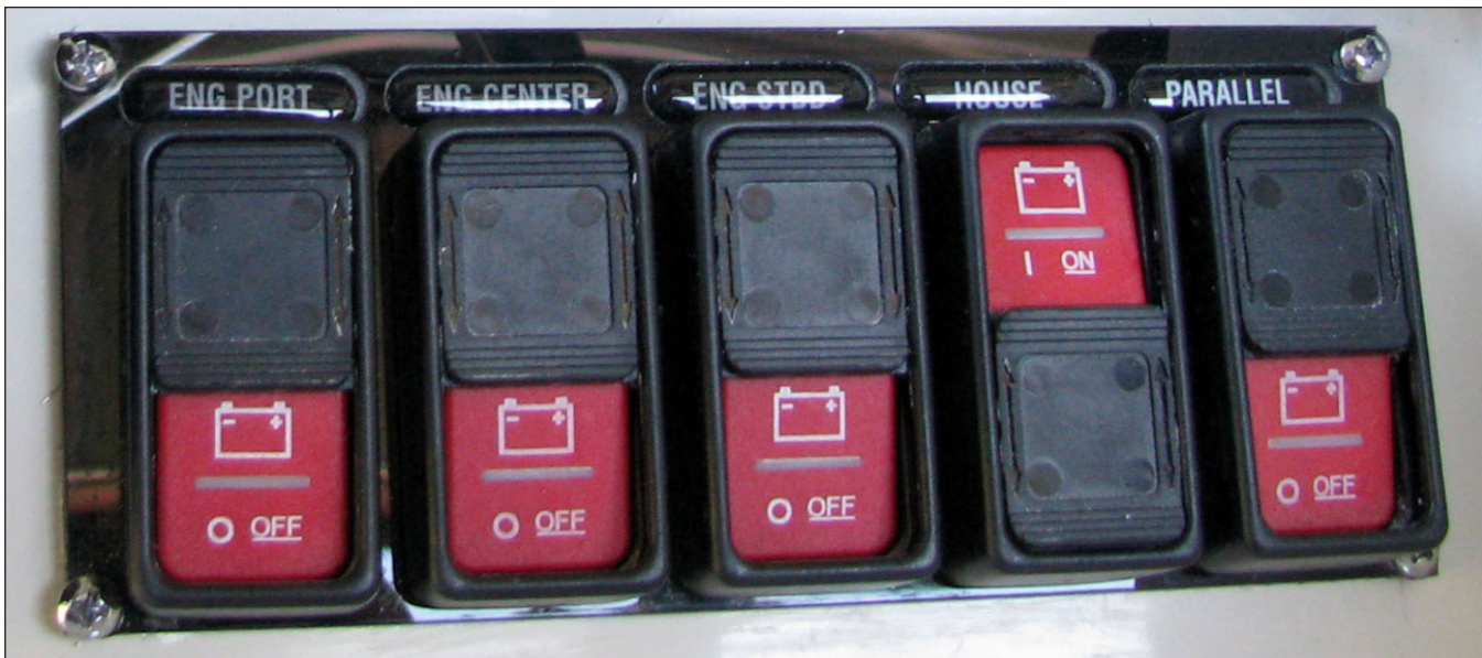
Battery Switch Panel at Helm
