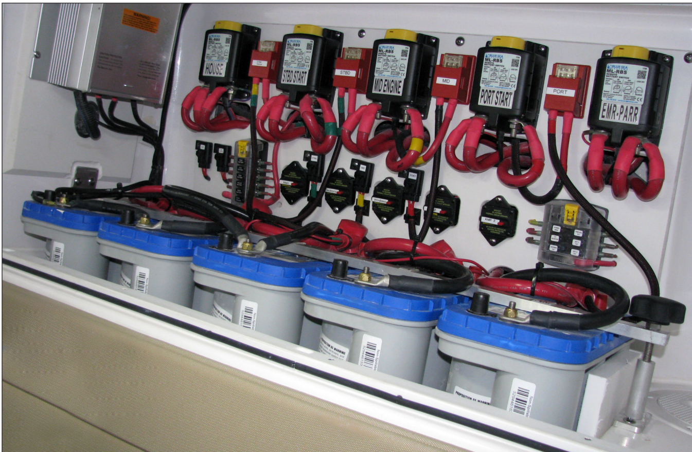
Battery Switches, Emergency Parallel Switch, Main Circuit Breakers & Continuous Power Fuse Panels
