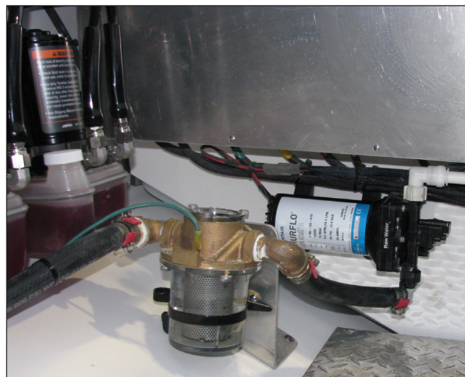
Raw Water Pressure Pump & Sea Strainer
