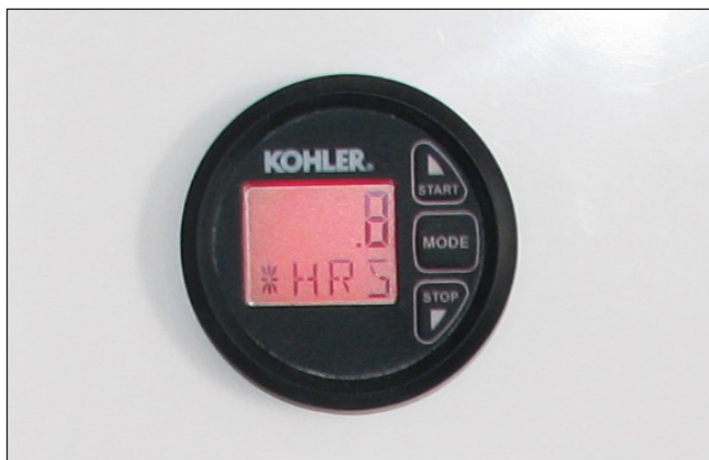
Cabin Generator Control Switch & Monitor
