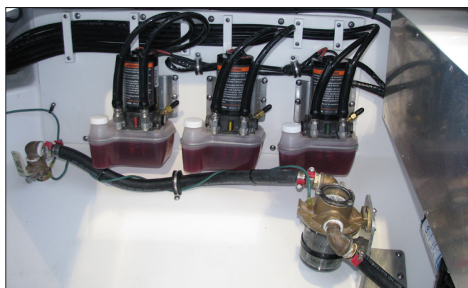
Raw Water Pressure Pump Seacock Valve & Sea Strainer
