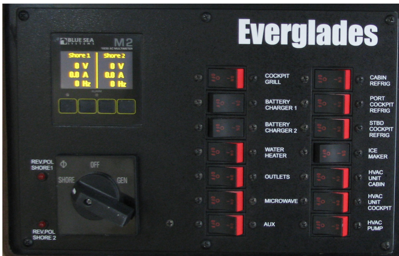
120 Volt AC Panel, SHORE/OFF/GENERATOR Selector Switch, Multimeter & Accessory Circuit Breakers
