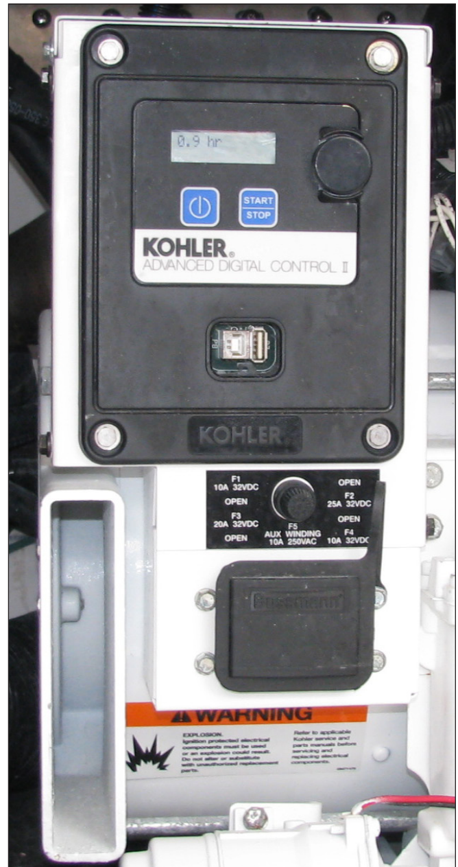
Generator Onboard Control Switch & Engine Monitor, Fuses & Circuit Breaker
