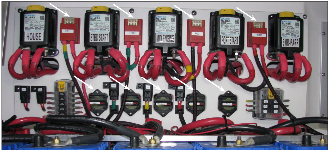
Battery Compartment Main Circuit Breakers & Fuses
