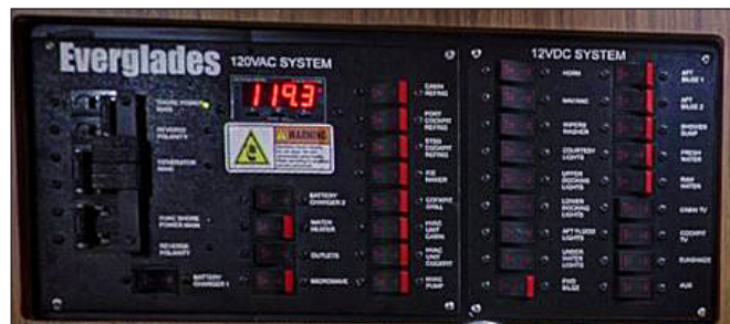
Cabin AC/DC Panels
