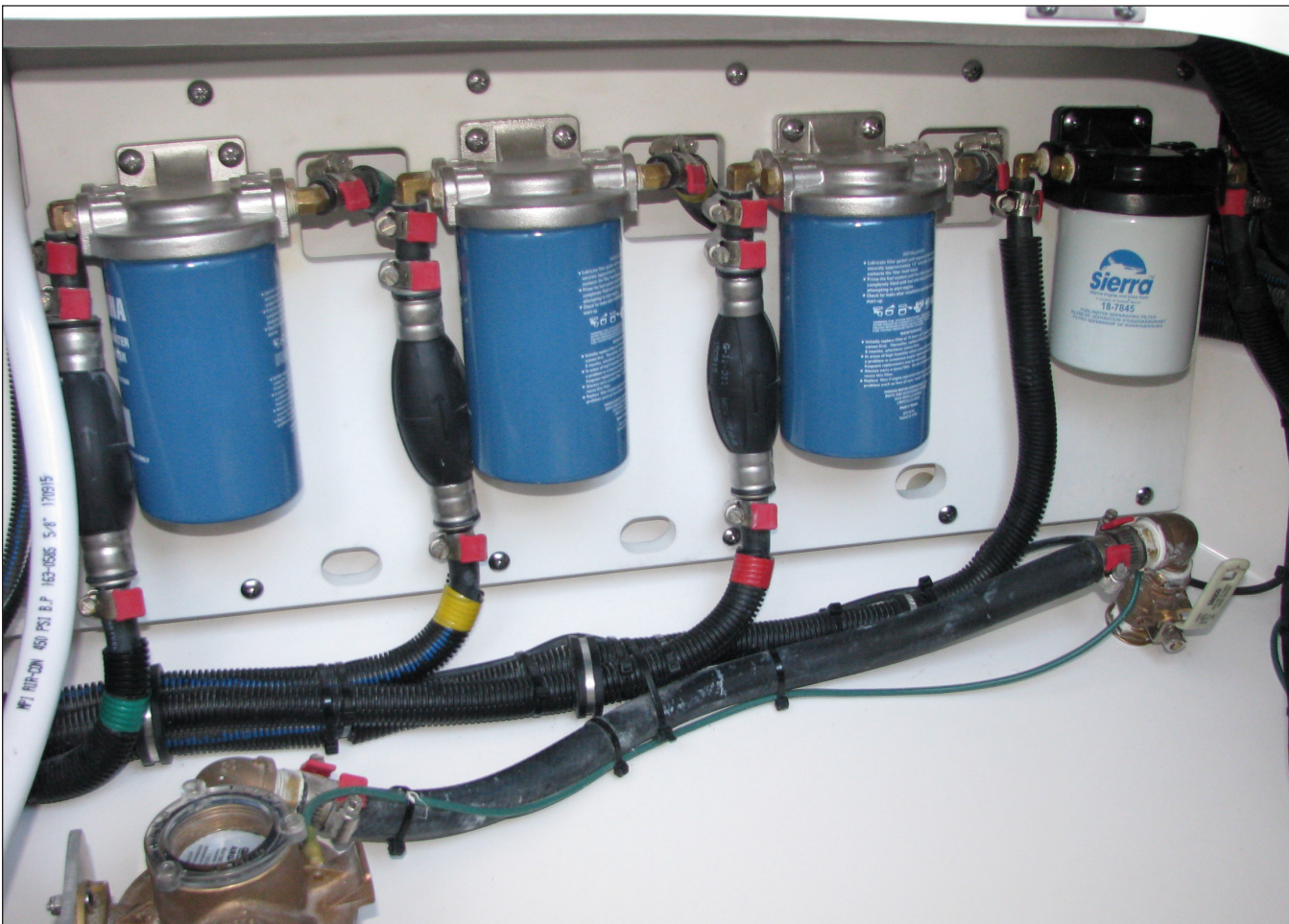
Generator & Engine Fuel filters & Primer Bulbs
