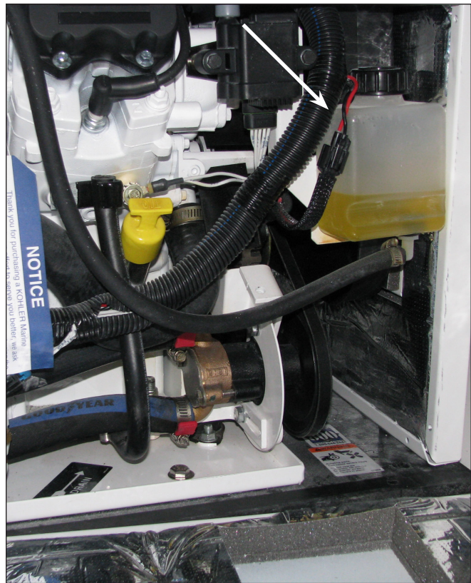
Generator Coolant Recovery Tank
