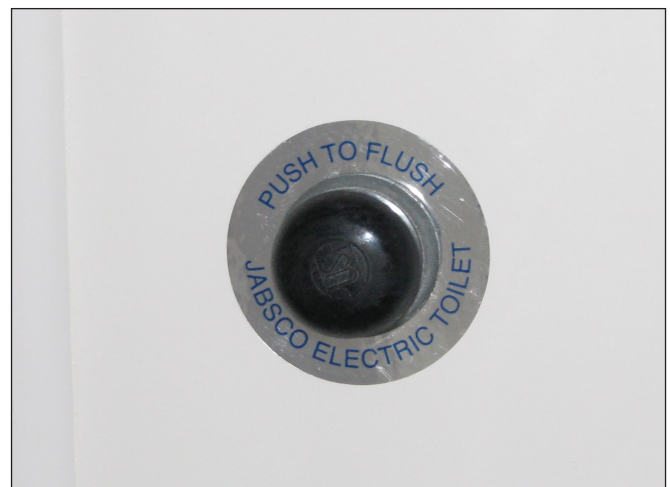
Toilet Flush Switch
