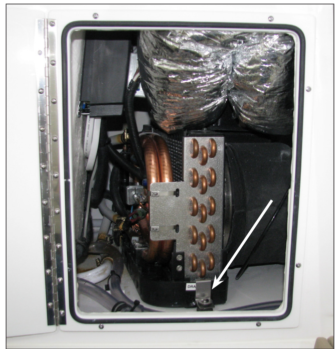
Cockpit Air Conditioner & Drain Pan in Aft Berth
