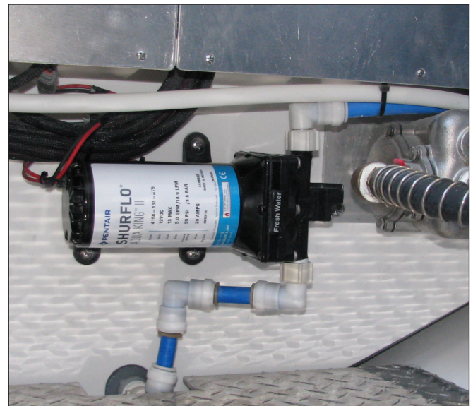
Fresh Water Pump
