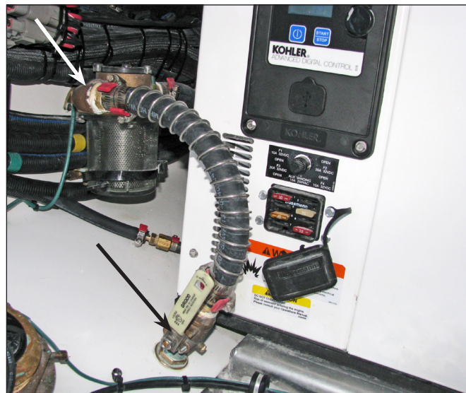
Generator Seacock Valve & Strainer
