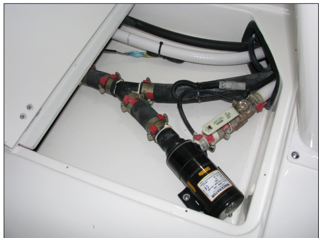
Macerator Pump & Overboard Discharge Thru-Hull Valve
