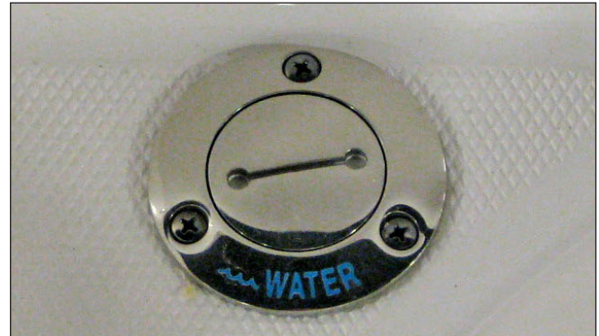
Fresh Water Fill
