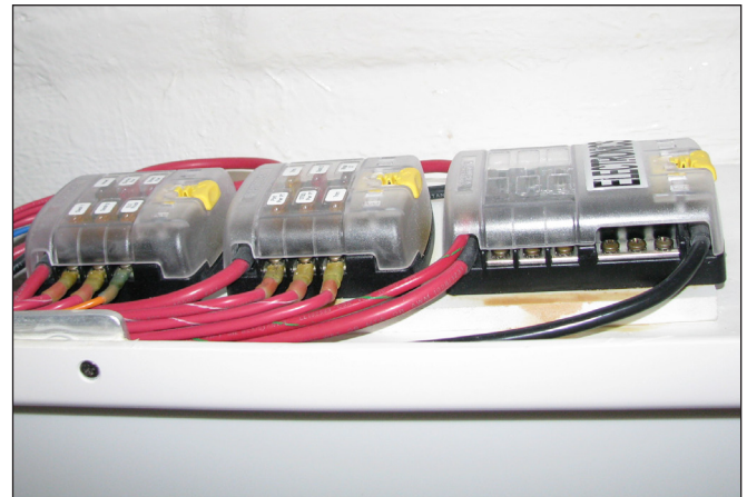
Electronics and Accessory Fuse Panels Behind Helm
