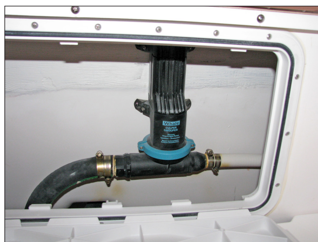
Forward Fishbox Macerator Pump Behind the Removable Hatch in the Forward Storage Compartment
