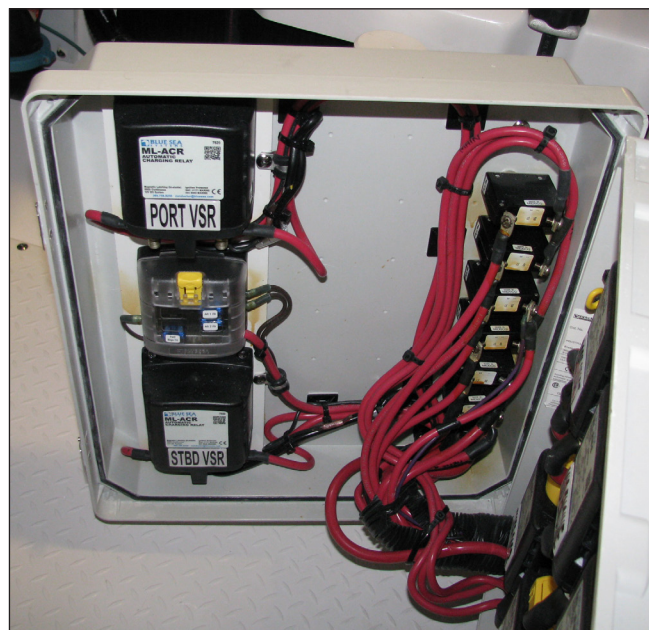
PT & STBD Voltage Sensitive Relays, Main Circuit Breakers and Continuous Power Fuse Panel
