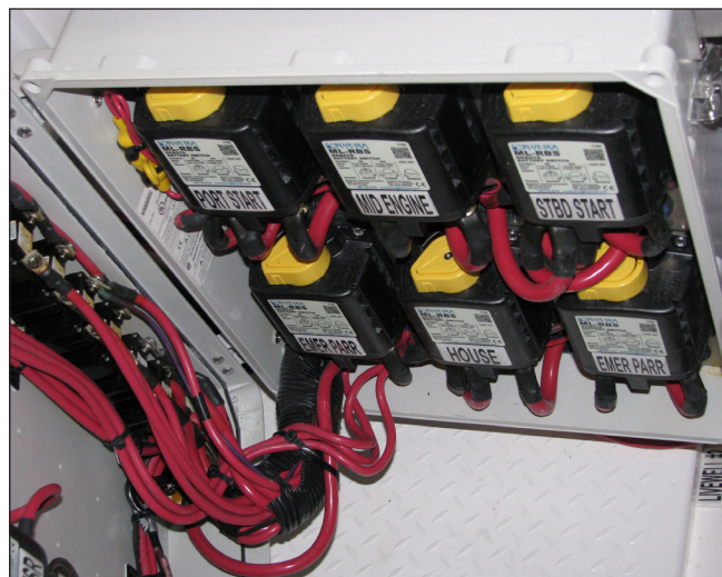
Battery Switches and Emergency Parallel Switches
