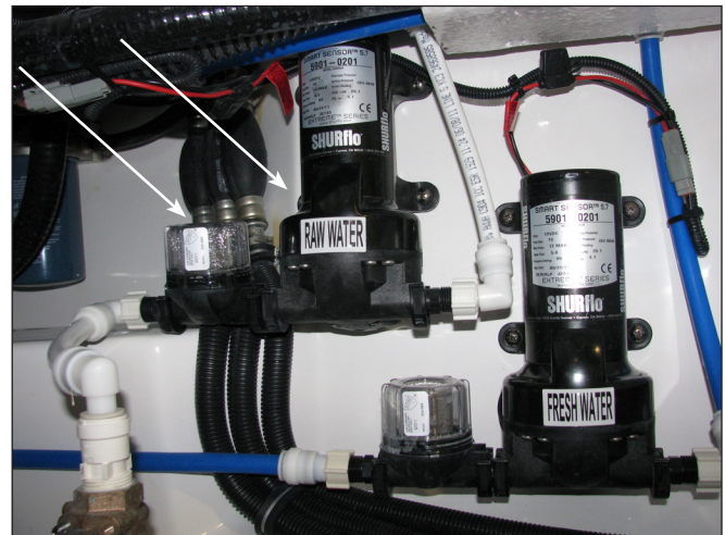
Typical Raw Water and Fresh Water Pressure Pumps and Sea Strainer Located in the Starboard Rear Corner of the Systems Compartment
