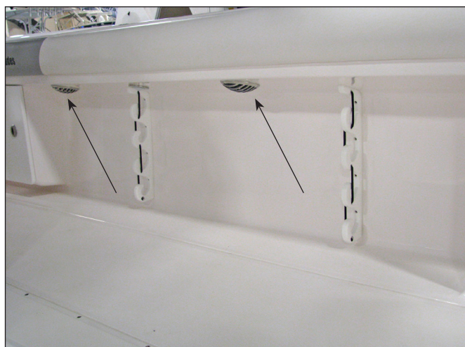
Bilge and Systems Compartment Vents
