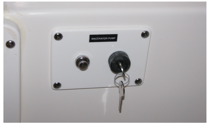
Typical Waste Discharge and Lockout Switches
