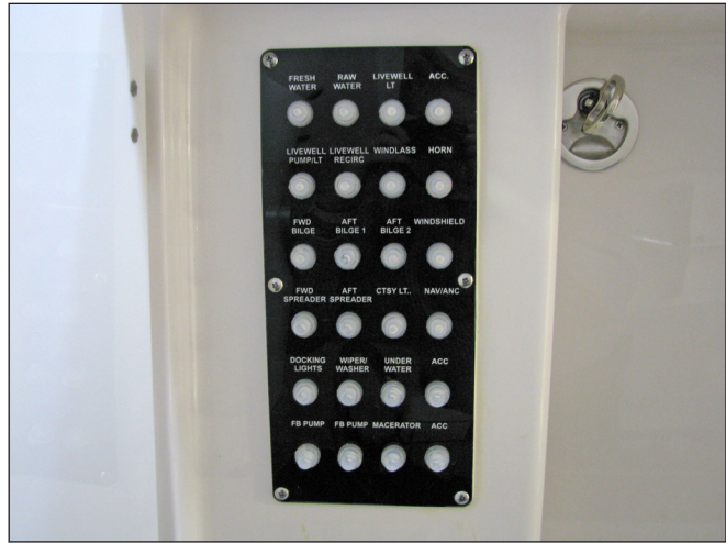
DC Circuit Breaker Panel
