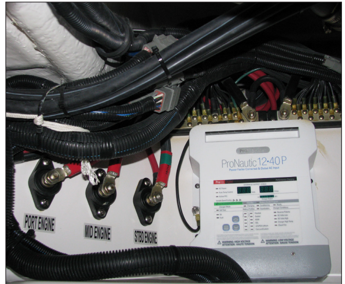
Typical Battery Charger in Systems Compartment
