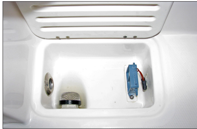
Head and Shower Sump System
