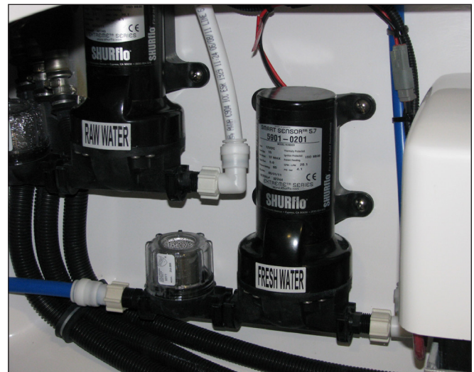
Fresh Water Pump and Strainer
