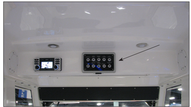
Hard Top Switch Panel
