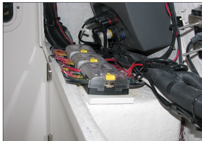
Fuse Panels Behind Helm
