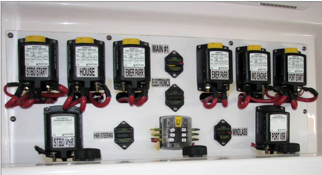
Battery Switches, Emergency Parallel Switches, PT & STBD Voltage Sensitive Relays, Main Circuit Breakers and Continuous Power Fuse Panel
