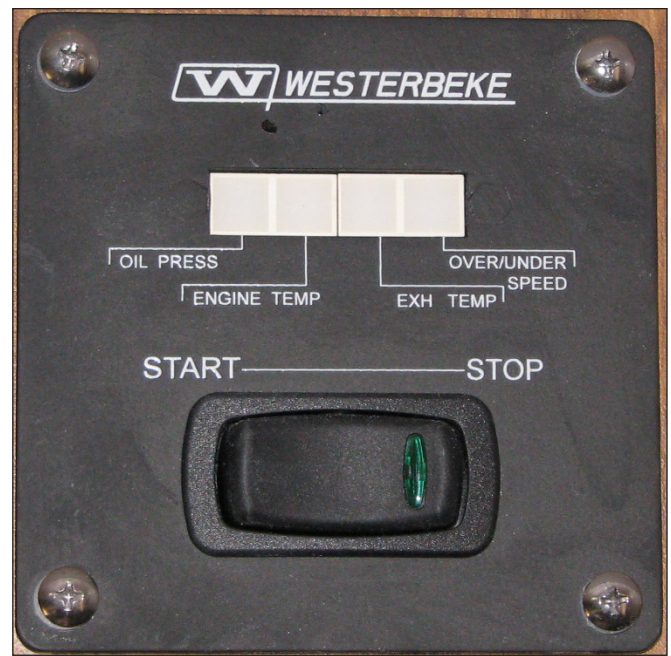
Cabin Generator Control Switch and Monitoring Lights
