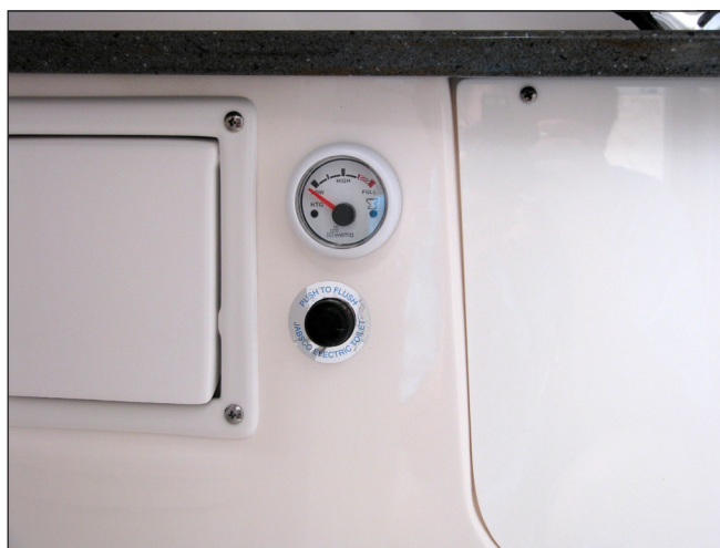
Holding Tank Gauge and Head Flush Switch
