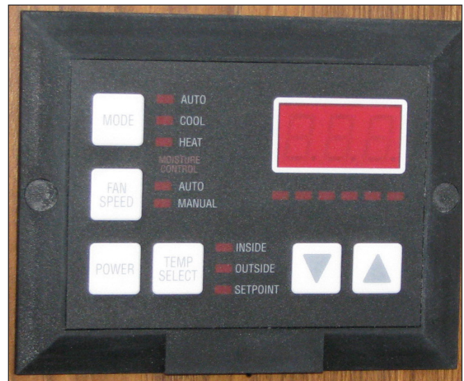
Air Conditioner Control Panel
