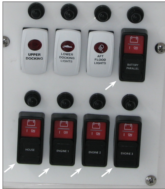
Parallel and Battery Switches
