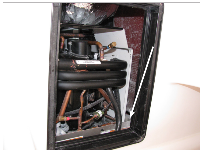
Air Conditioning Condensation Pan
