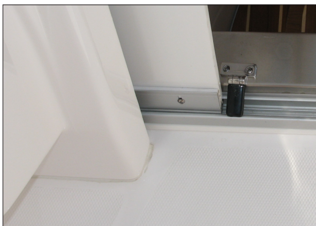
Cabin Door Latched in Open Position
