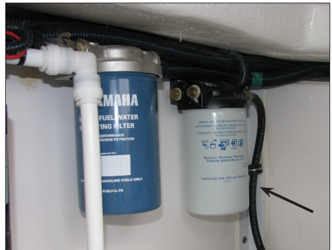
Generator Water Separator Filter
