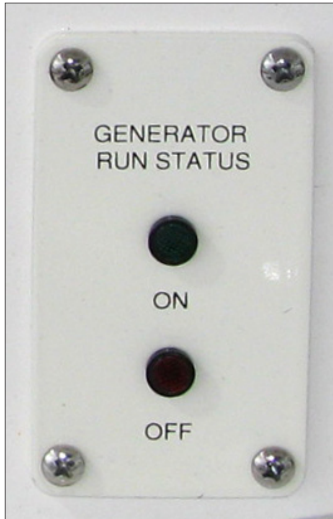
Generator Run Status Panel at the Helm
