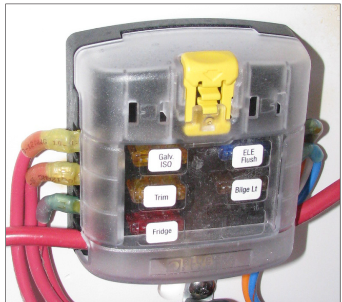
Typical Cabin DC Fuse Panel
