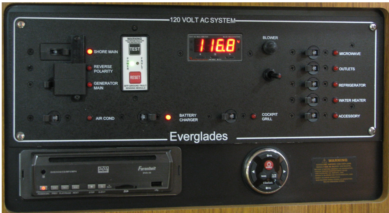
Cabin AC Circuit Breaker Panel
