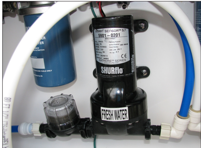
Fresh Water Pump and Strainer
