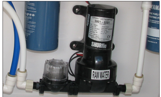
Raw Water Pressure Pump and Sea Strainer
