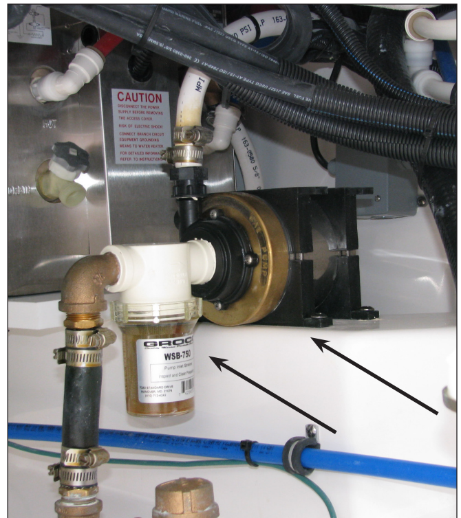
Air Conditioner Seawater Pump and Strainer
