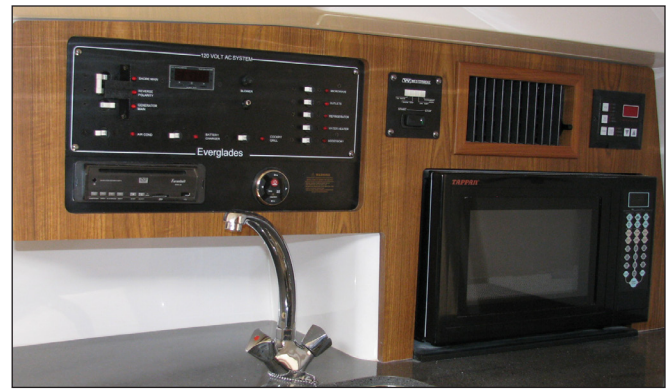
120 Volt AC Breaker Panel, Generator Control Panel and Air Conditioning Control Panel Above Gally
