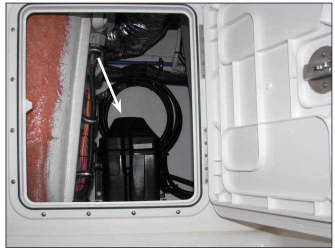
Power Steering Unit in Behind Access Hatch in Aft Berth
