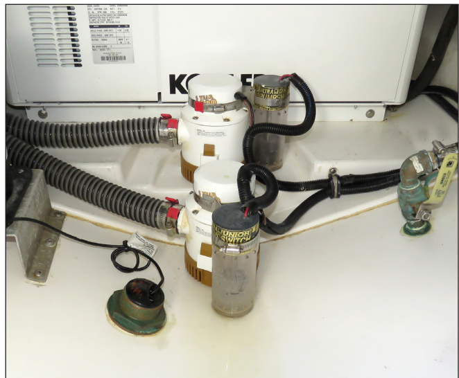
Aft Bilge Pumps & Automatic Switches
