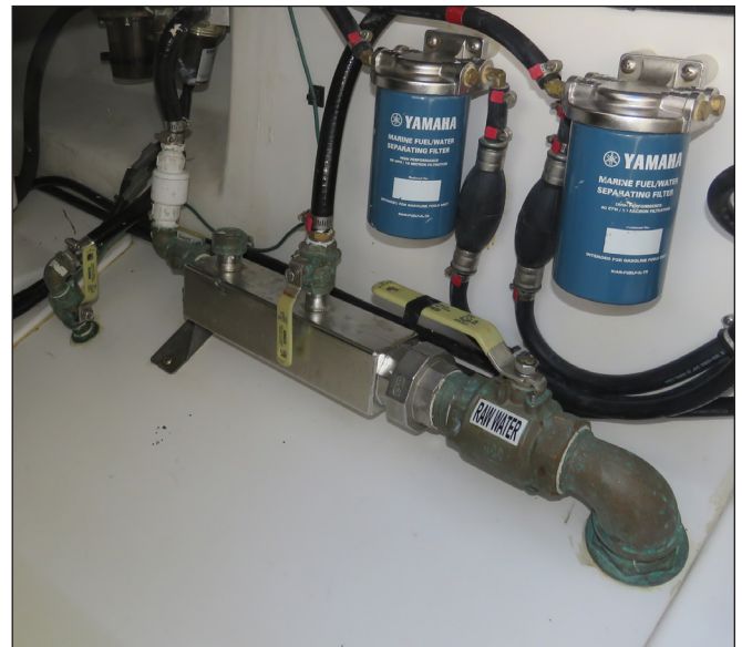
Raw Water System Manifold & Valves
