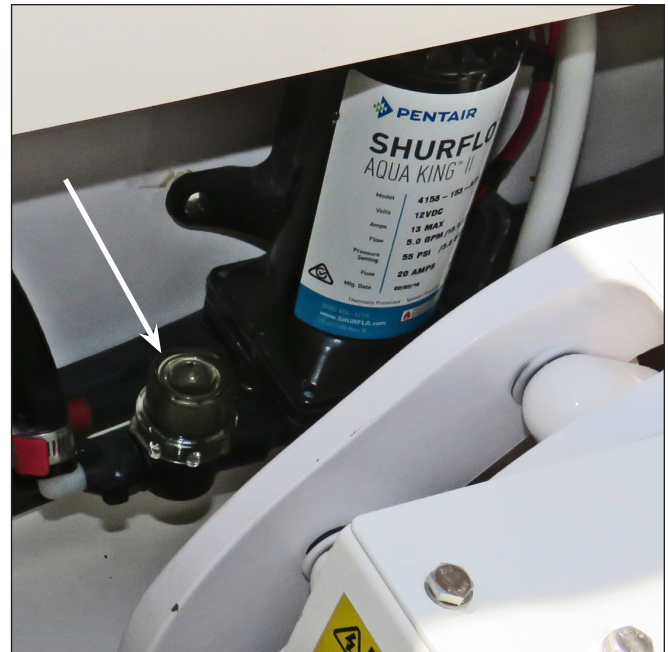
Raw Water Pump Strainer
