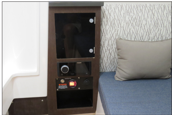
120 Volt AC Panel, Generator Control Panel & Stereo
