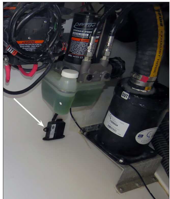
Bilge High Water Alarm Automatic Switch
