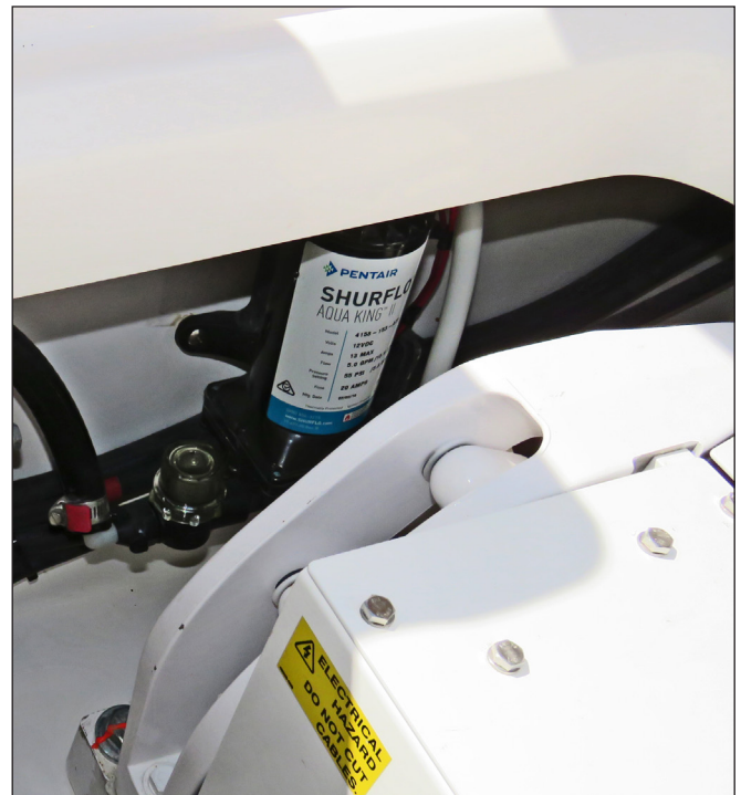
Raw Water Pressure Pump & Sea Strainer
