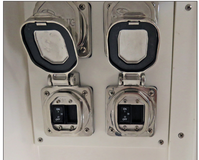
Shore Power Inlet Circuit Breakers
