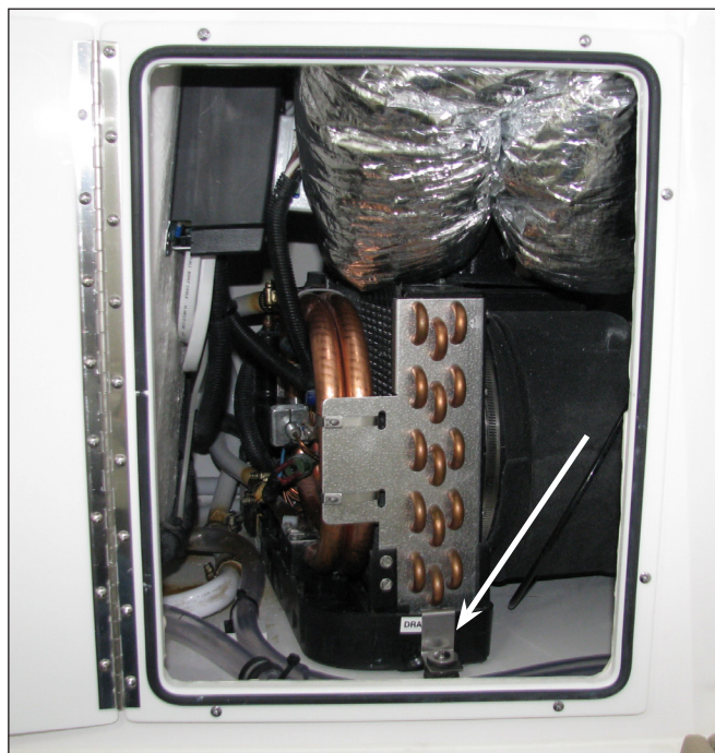
Typical Air Conditioner & Drain
