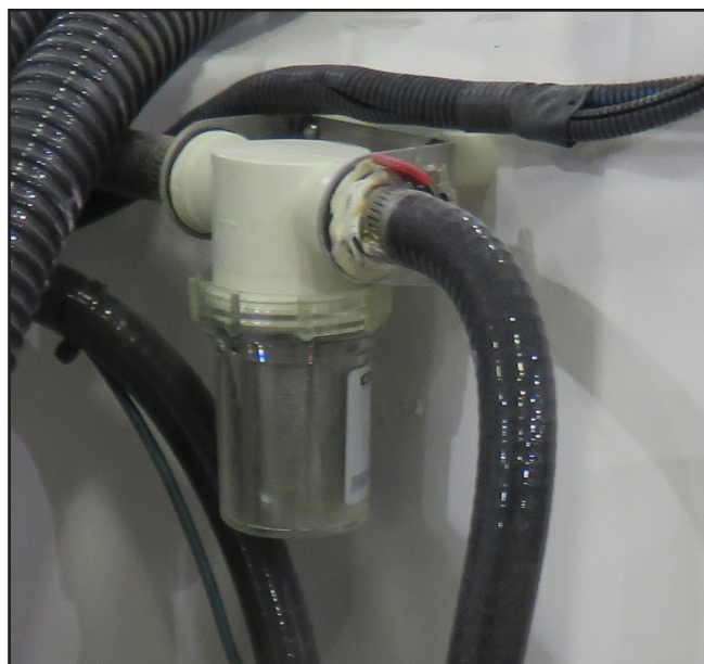
Typical Air Conditioner & SeaKeeper Pump Strainer
