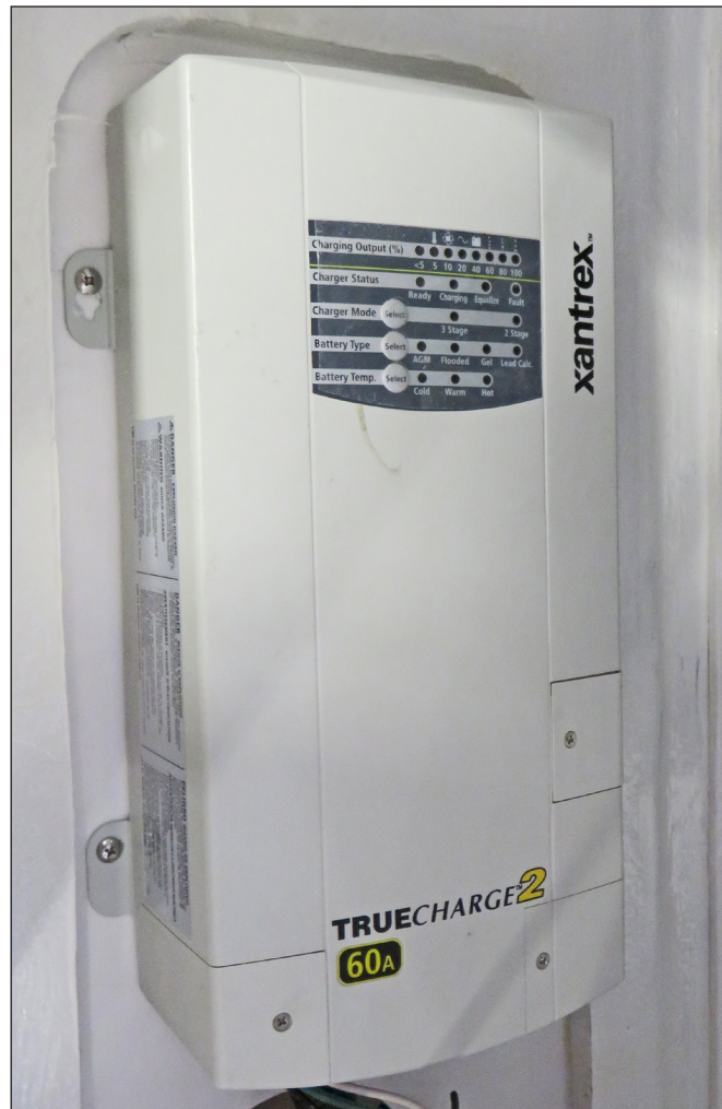
Typical Battery Charger
