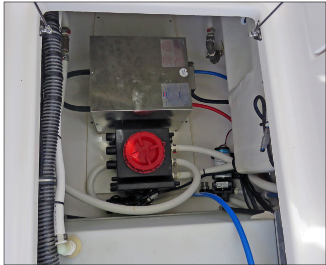
Drain Sump System
