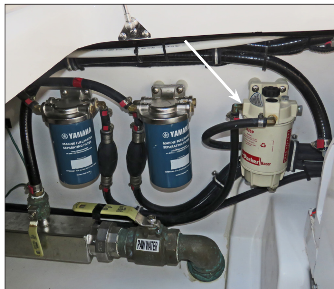
Generator Fuel Filter
