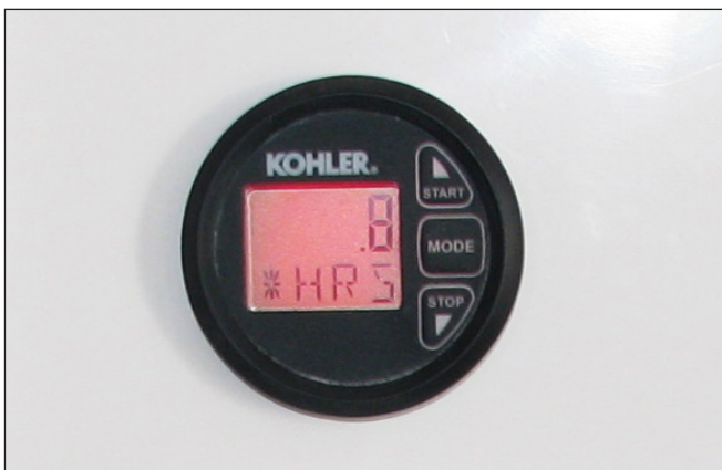
Cabin Generator Control Switch & Monitor
