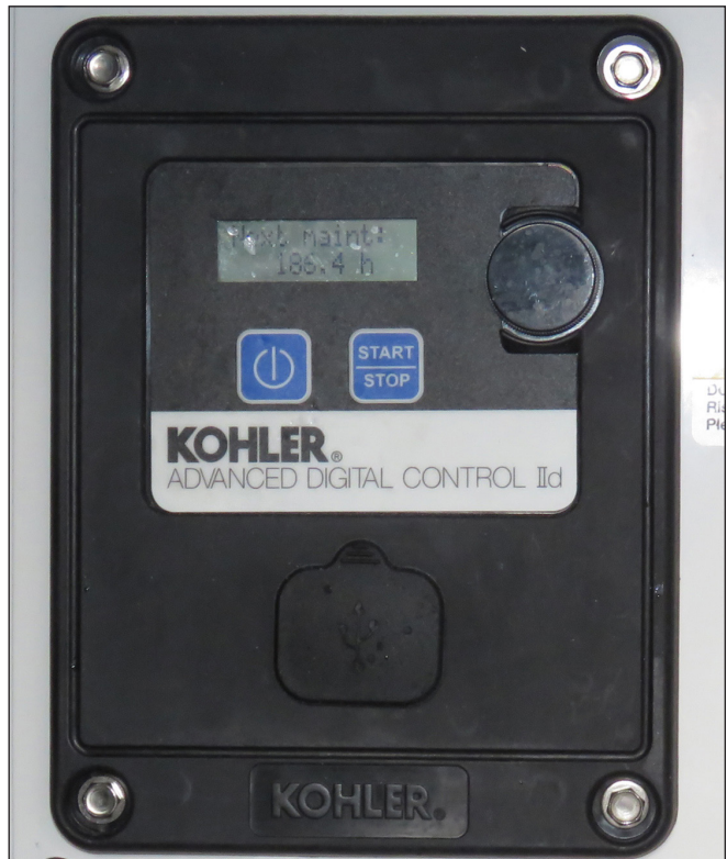
Generator Onboard Control Switch & Engine Monitor, Fuses & Circuit Breaker
