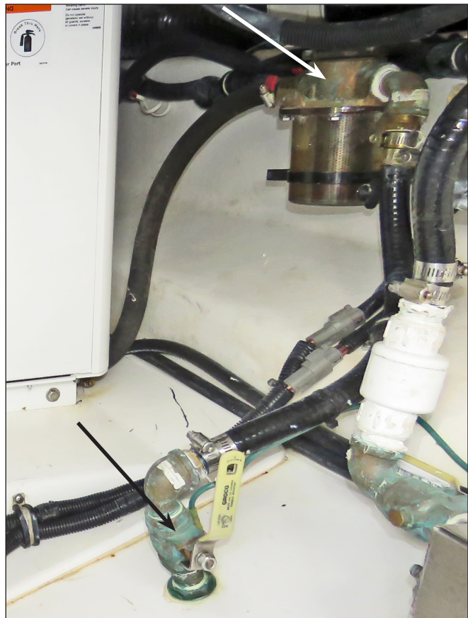
Generator Seacock Valve & Strainer
