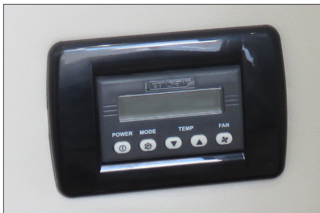
Typical Air Conditioner Control Panel
