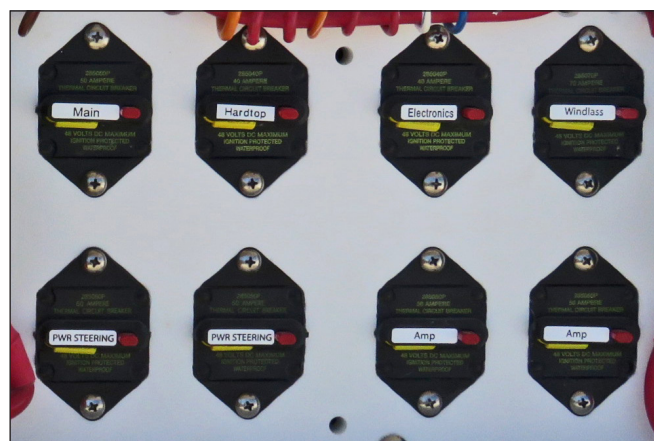
Main Circuit Breakers
