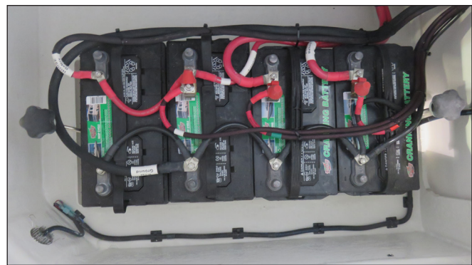
Engine & House Batteries
