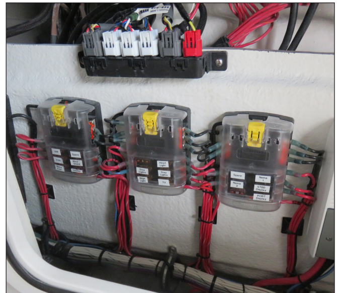
Electronics Fuse Panels Below Helm
