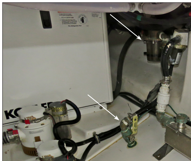
Generator Strainer & Seacock
