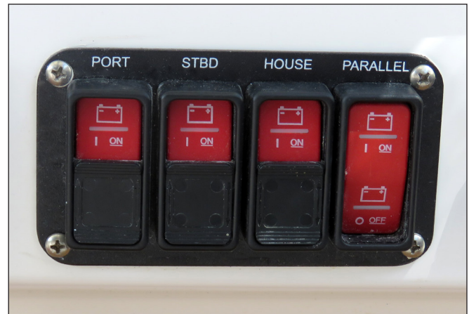
Remote Battery Switches At Helm
