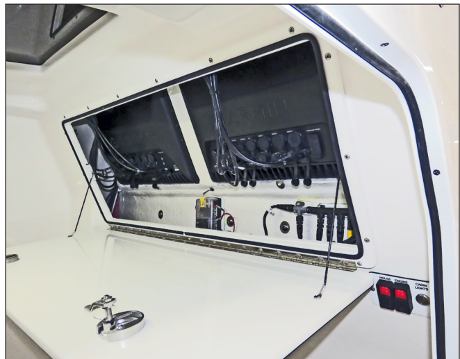
Fuse Panel & Electronics Behind Access Door
