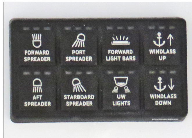
Starboard Hardtop Switch Panel
