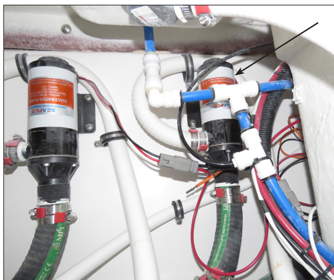
Waste Overboard Discharge Pump
