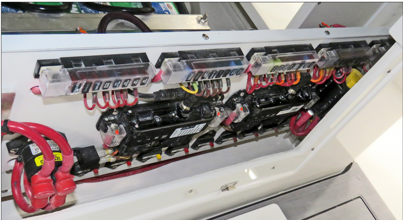
Accessory Fuse Panels On Fuse & Breaker Panel In Battery Compartment
