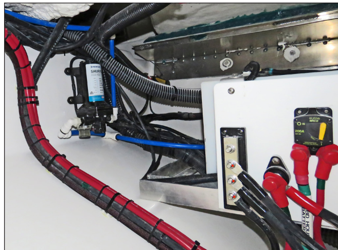
Fresh Water Pump
