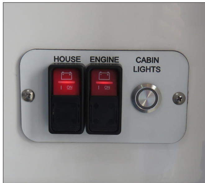
Battery Switches On Panel In Head Compartment
