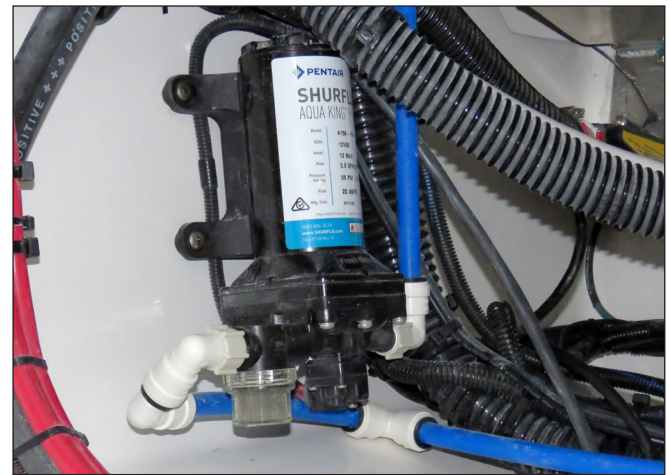
Fresh Water Pump & Strainer
