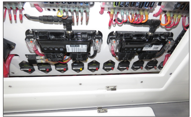
Digital Switching Control Modules
