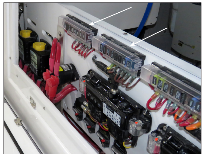
Continuous Power Fuse Panels
