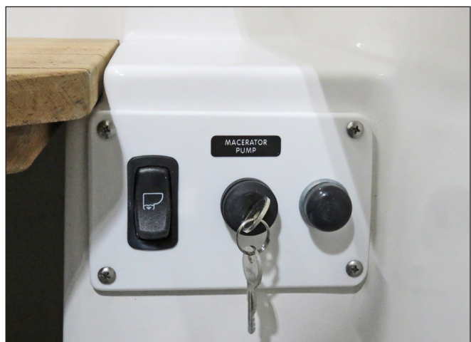
Head & Macerator Switch Panel
