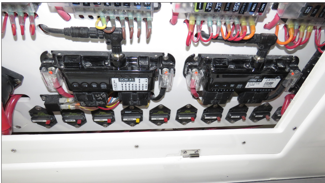
Main Circuit Breakers On Fuse & Breaker Panel In Battery Compartment
