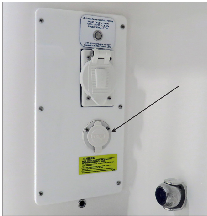
Shore Power Cable Inlet Connection
