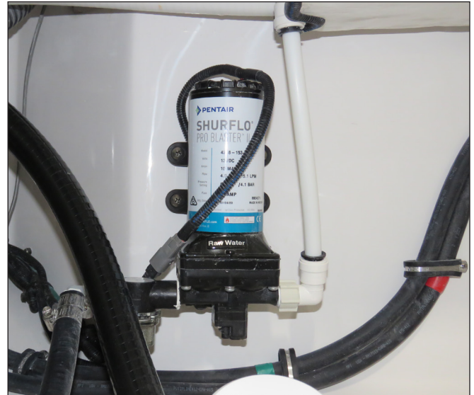
Raw Water Pressure Pump & Sea Strainer
