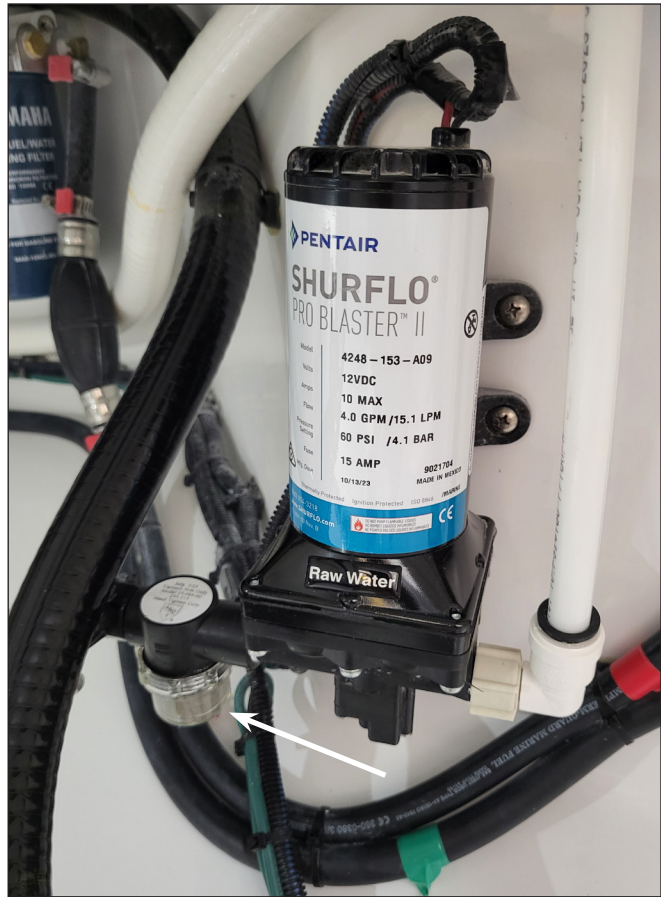
Typical Raw Water Pump Sea Strainer
