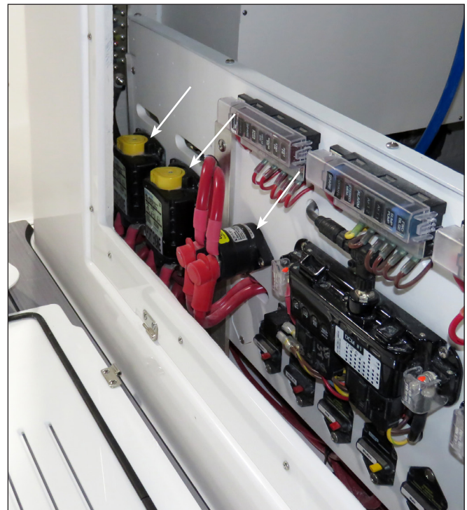
Starboard Engine & House Battery Switches & Parallel Relay On Fuse and Breaker Panel In The Battery Compartment
