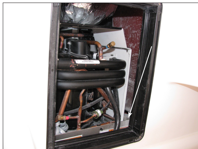
Typical Air Conditioning Condensation Pan
