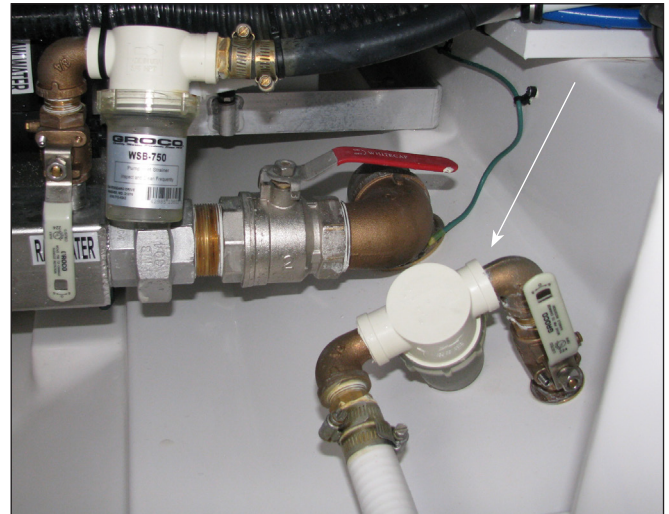
Generator Sea Strainer and Seacock Valve
