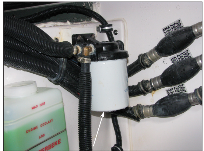
Generator Water Separator Filter
