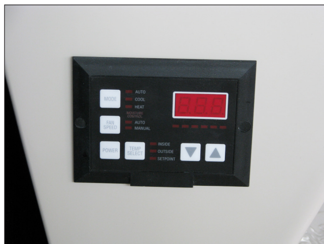
Helm Air Conditioning Control
