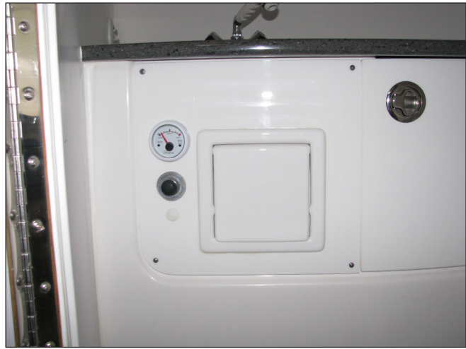
Holding Tank Gauge and Head Flush Switch
