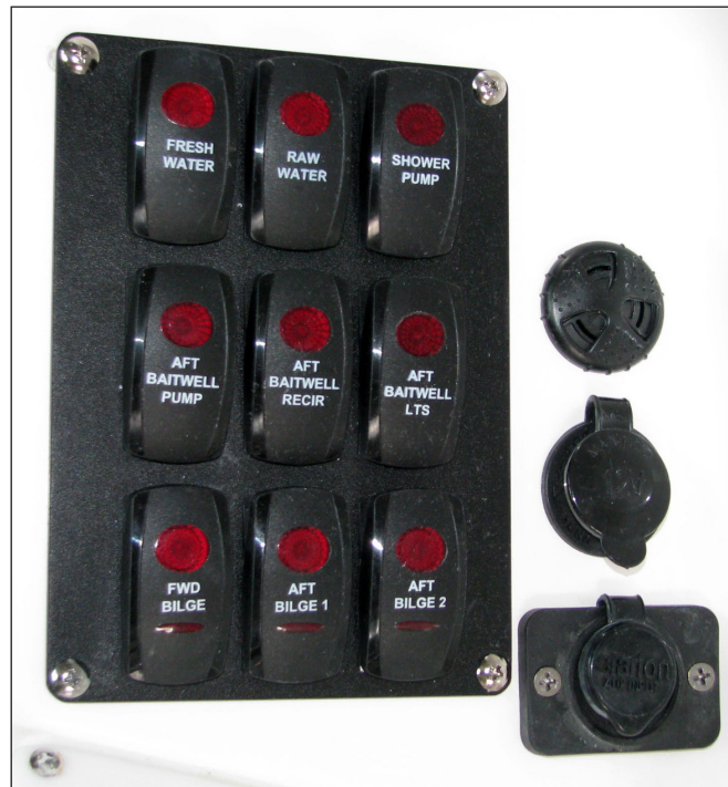
Accessory Switch Panel 2, Engine Alarm, Accessory Plug and MP3 Connection in Storage Compartment on Starboard Side Of Helm
