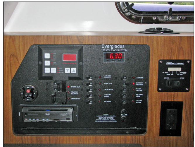
120 Volt AC Breaker Panel, Generator Control Panel and Air Conditioning Control Panel Above Gally
