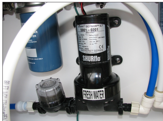
Typical Fresh Water Pump and Strainer
