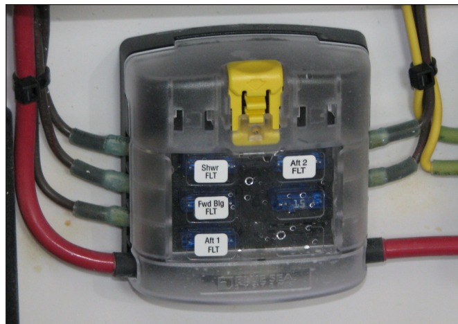
Continuous Power Fuse Panel 1
