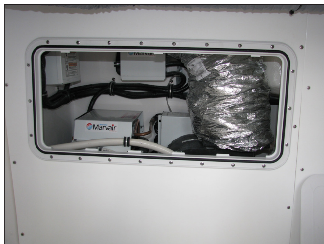
Access to Helm Air Conditioning Unit in Work Station /Tackle Storage Compartment
