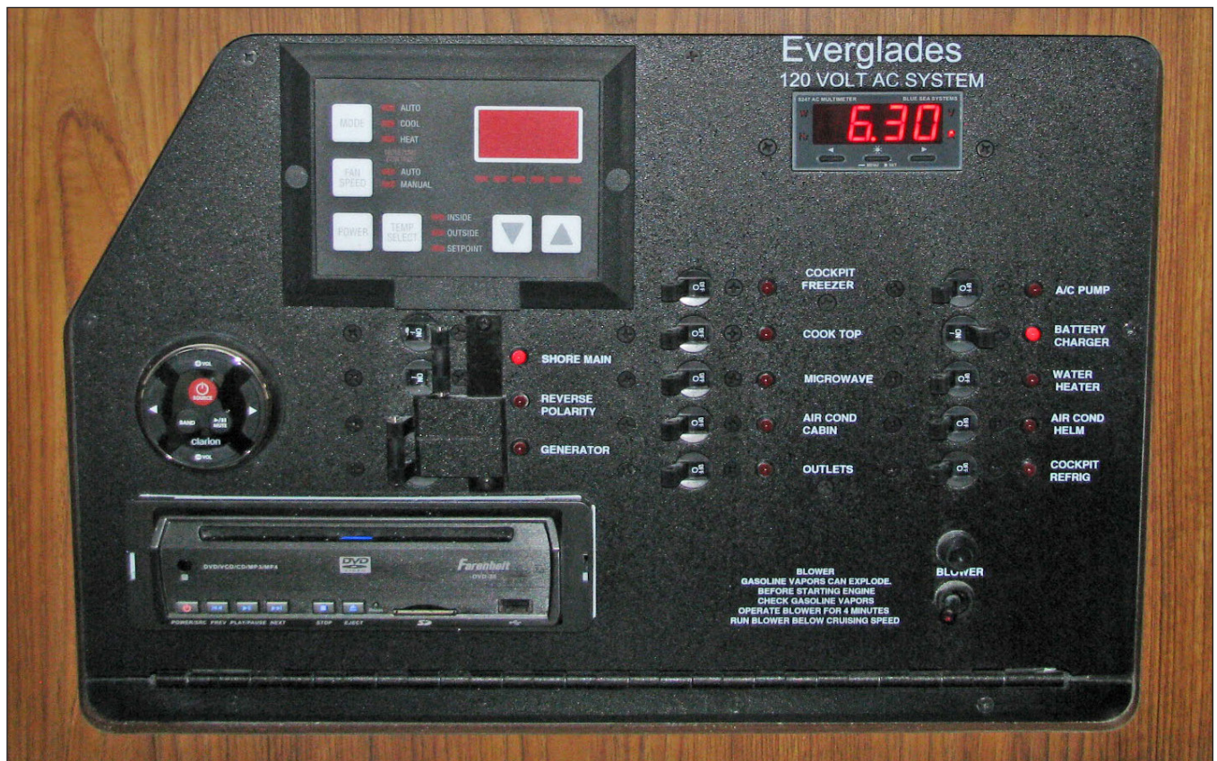
Cabin AC Circuit Breaker Panel
