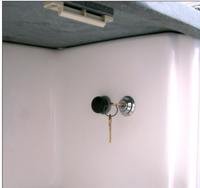
Typical Macerator Discharge and Key Lockout Switches In Compartment Near the Head
