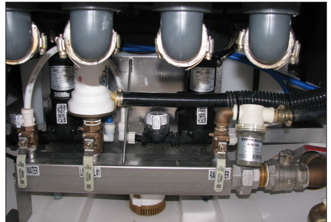
Fresh Water Pump Location in Systems Compartment
