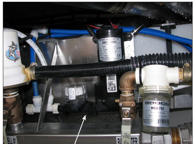
Raw Water Pump and Strainer
