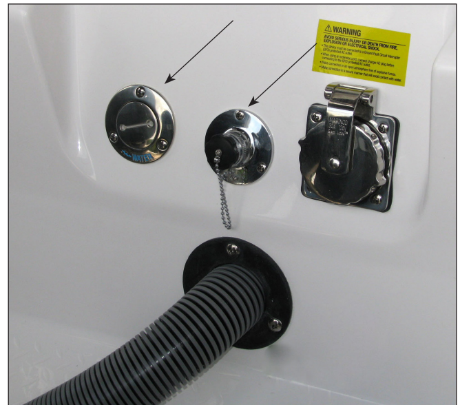
Fresh Water Fill and Shore Water Connection
