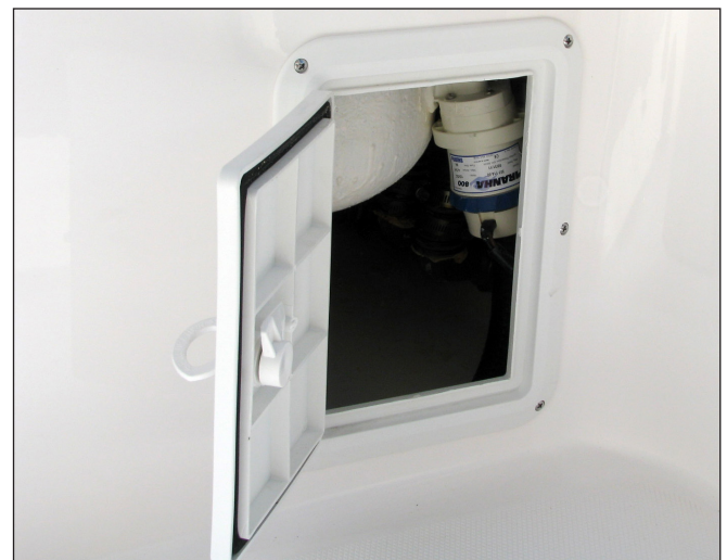
Baitwell Recirculation Pump
