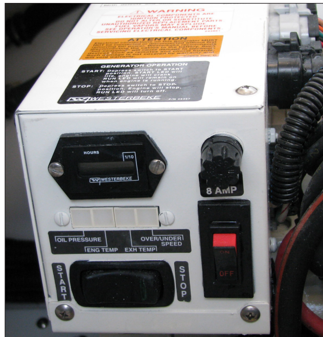
Generator Onboard Control Switch and Engine Monitor, Fuses and Circuit Breaker
