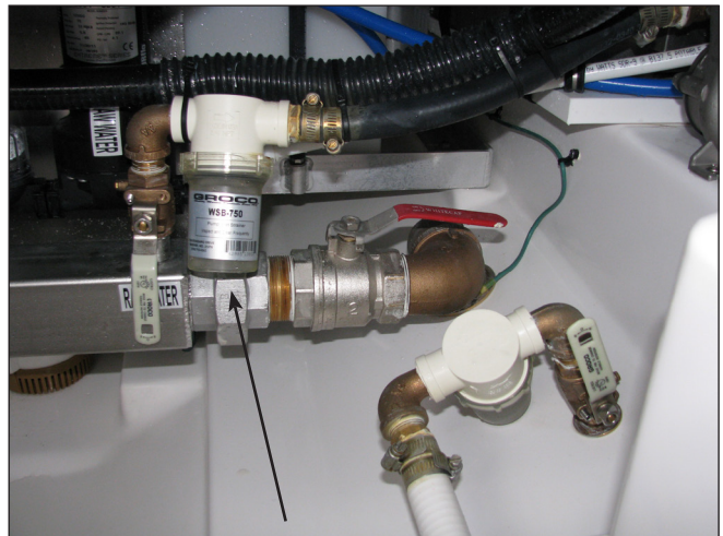
Air Conditioning Pump Sea Strainer and Valve
