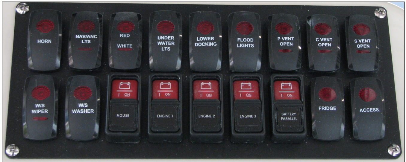
Main Accessory Switch Panel, Battery Switches and Emergency Parallel Switch in Helm
