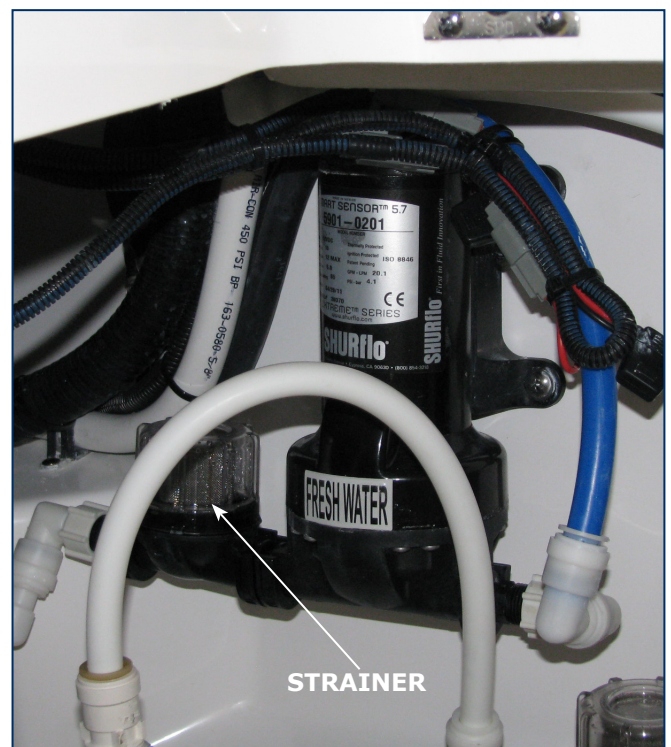
325 Pilot Fresh Water Pump and Strainer
