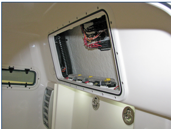
Helm Access Panel in Head Compartment
