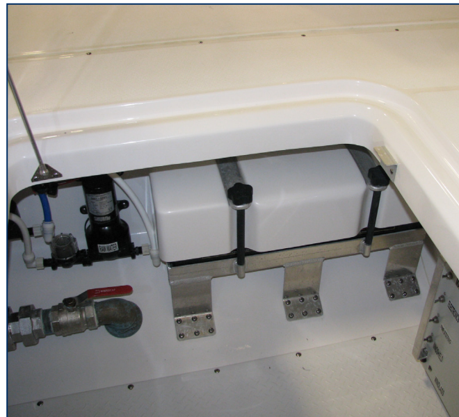
325 Pilot Port Battery Bank and Battery Box
