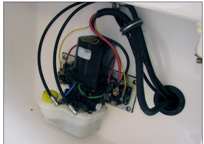
Hydraulic Pump System for Windshield In Head Compartment
