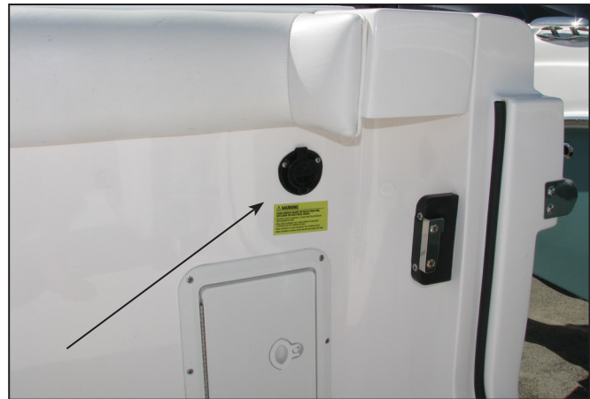
325 Pilot Shore Power Inlet Connection
