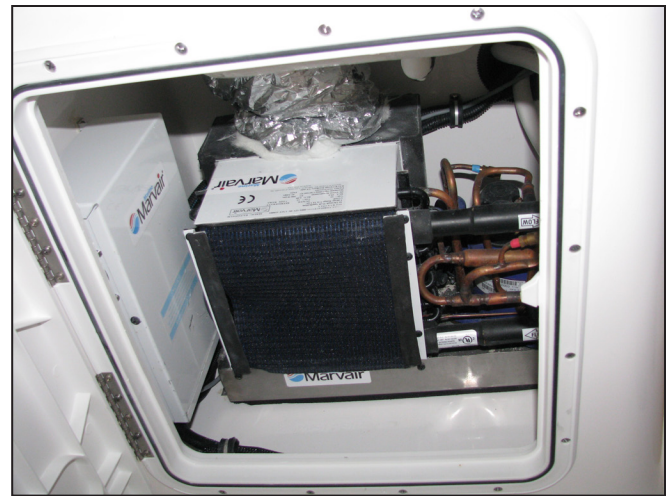
Air Conditioning System Below Head Compartment Sink
