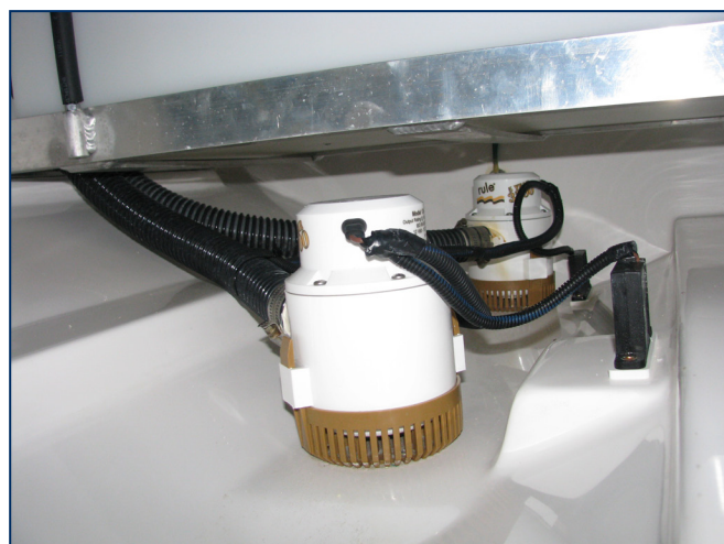
325 Pilot Aft Bilge Pumps and Automatic Switches
