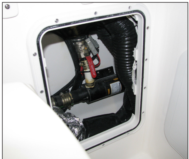
Macerator Overboard Discharge Pump and Valve
