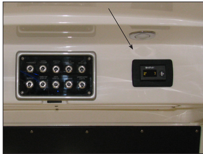
Air Conditioner Control Panel Above Helm in Pilot House
