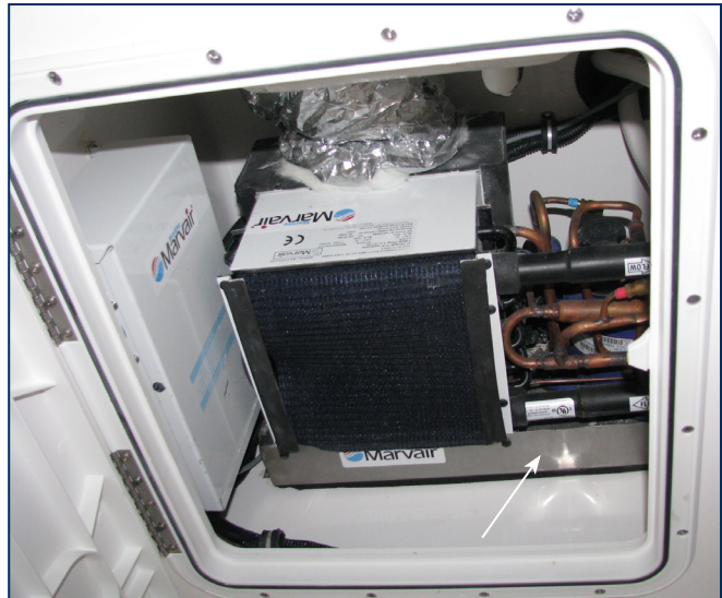
Air Conditioner Condensation Pan
