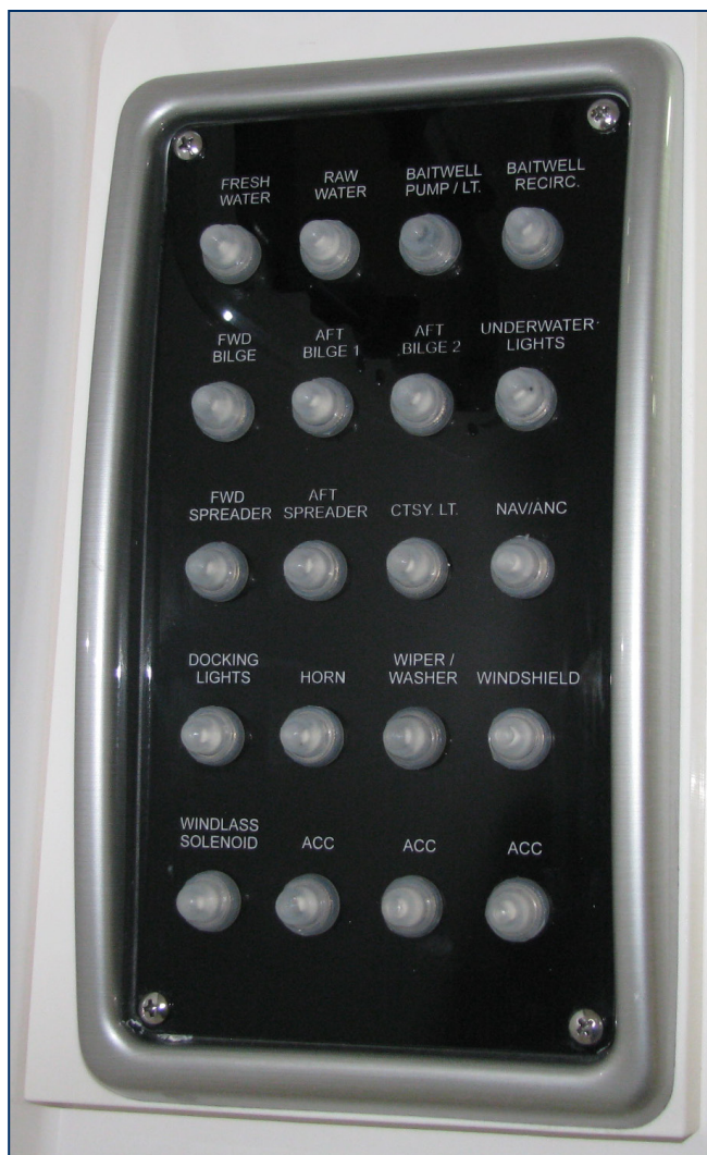
Head Compartment DC Circuit Breaker Panel
