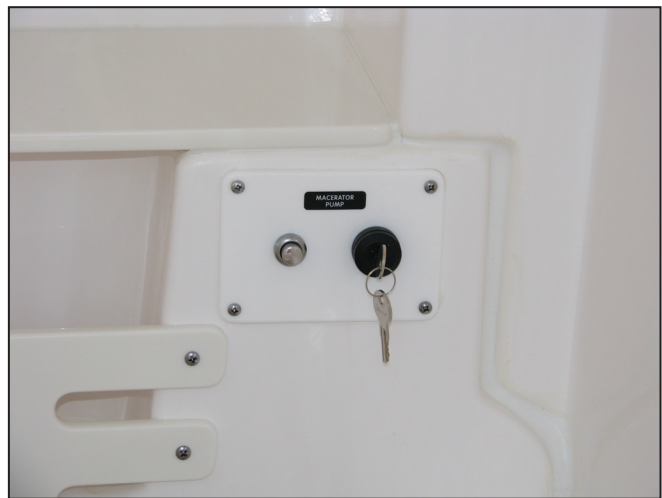
Waste System Pump Out Switch Panel
