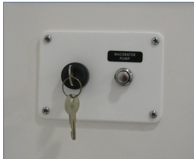
Head Compartment Macerator Pump Key Switch
