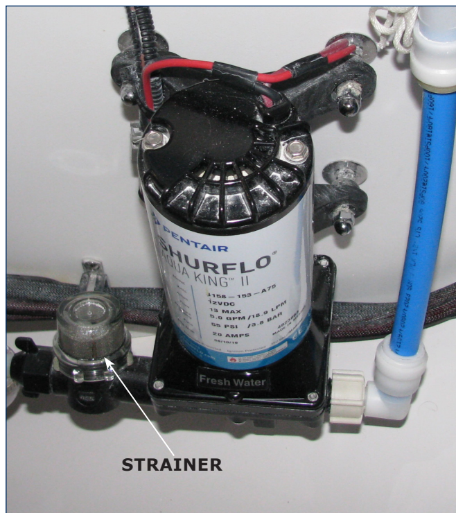
Fresh Water Pump & Strainer
