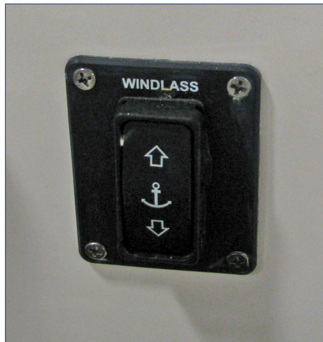
Anchor Locker Windlass Switch
