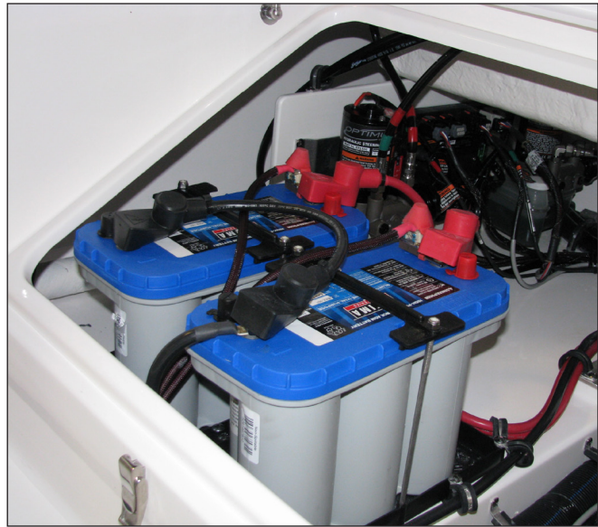
Typical AGM Batteries
