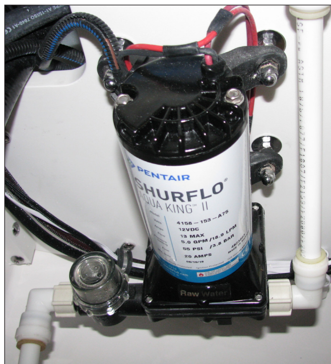
Raw Water Pressure Pump & Sea Strainer
