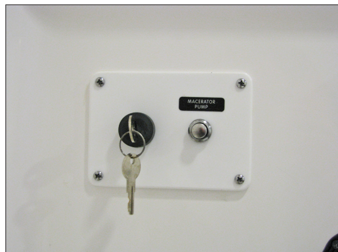
Waste System Pump Out Switch Panel
