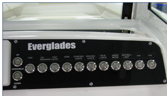
Starboard Side Helm Switches
