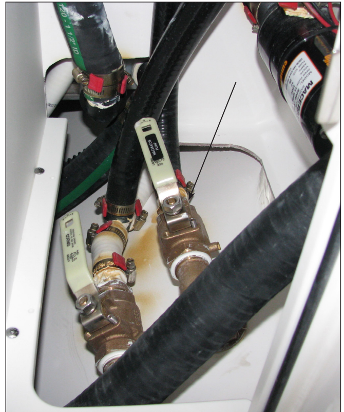
Overboard Discharge Thru-Hull Valve
