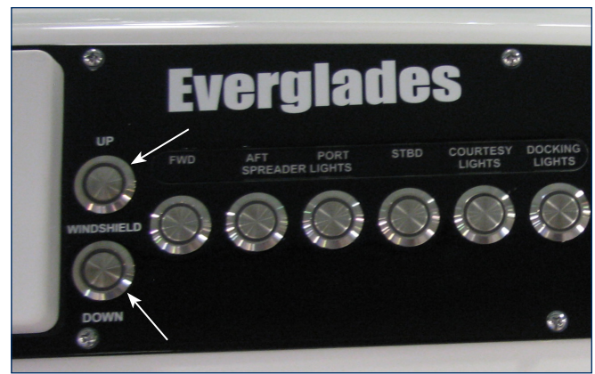
Helm Windlass Switches
