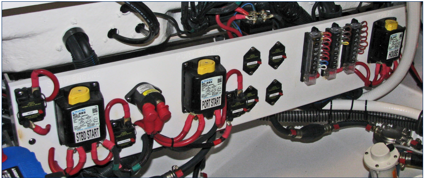
Battery Switch Panel In Aft Systems Compartment
