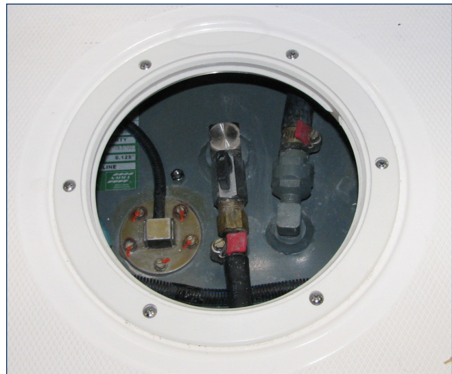
Fuel Withdrawal Valves & Tank Sending Unit
