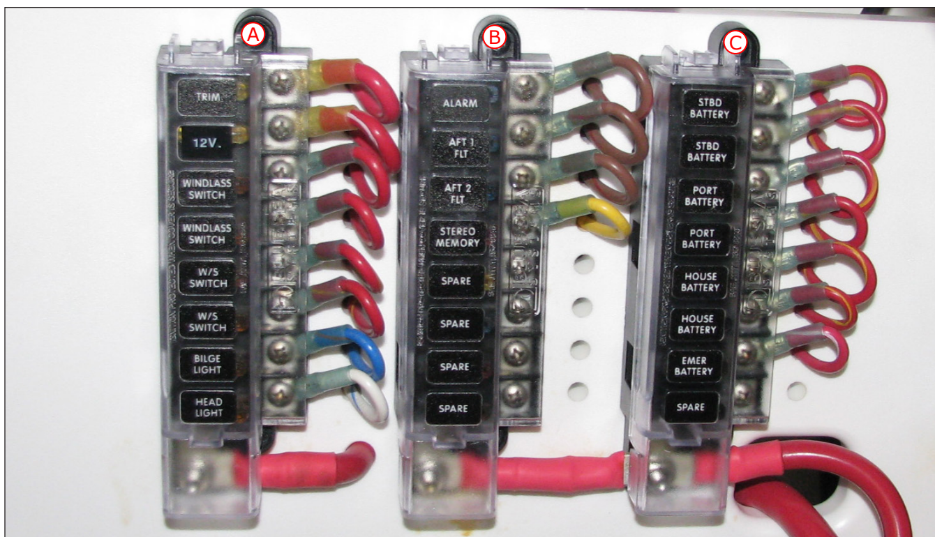
Accessory & Continuous Power Fuse Panels In Aft Systems Compartment A) Accessory Fuse Panel B) Continuous Power Fuse Panel C) Remote Battery Switch Fuse Panel
