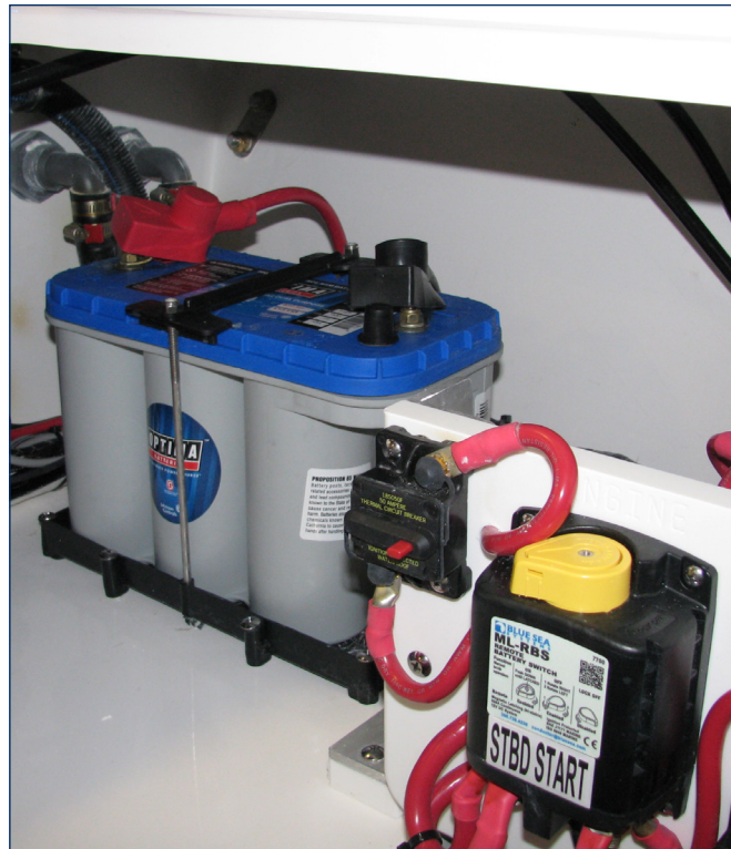
Typical AGM Battery
