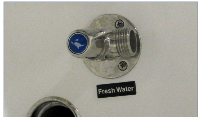
Fresh Water Washdown Hose Connection
