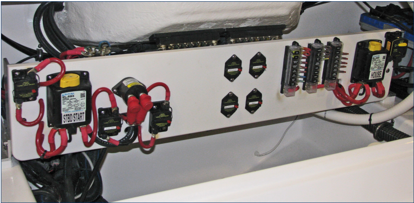
Battery Switches, Fuse Panels & Main Circuit Breakers
