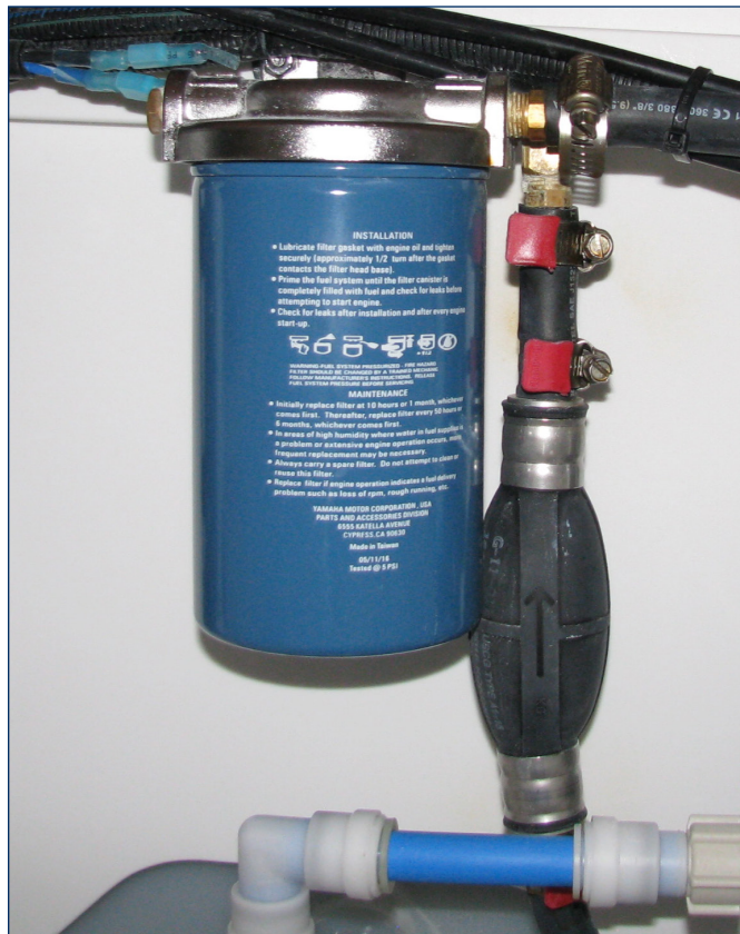
Typical Yamaha Fuel Filter In Aft Systems Compartment
