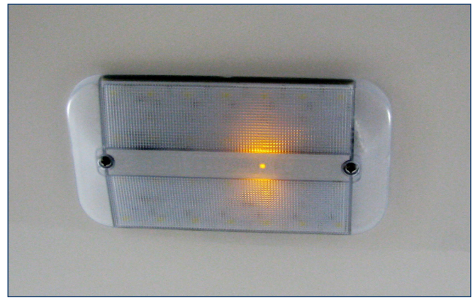
Aft System Compartment Light
