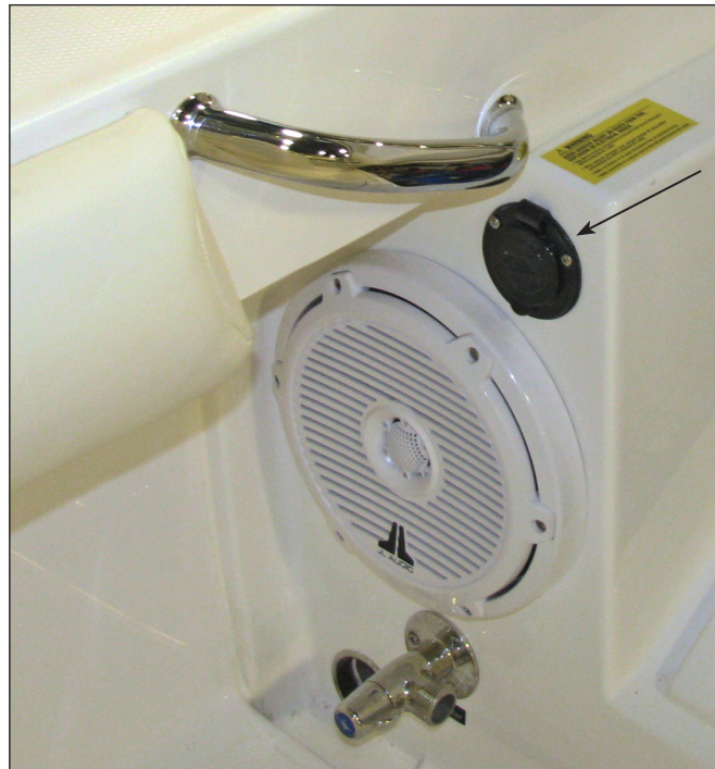
Typical 120 Volt Shore Power Inlet Connection
