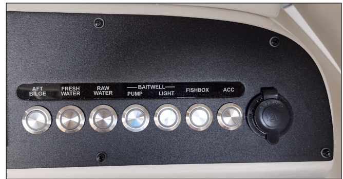
Starboard Helm Switch Panel
