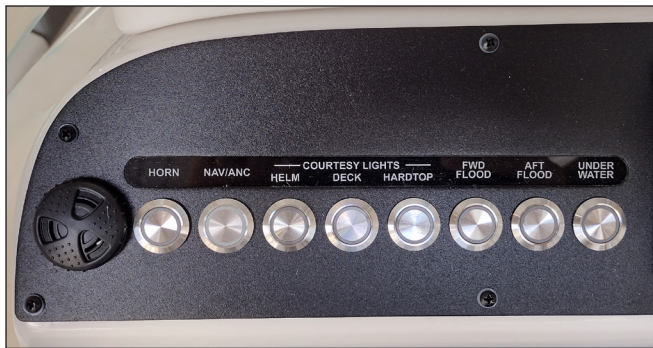
Port Helm Switch Panel
