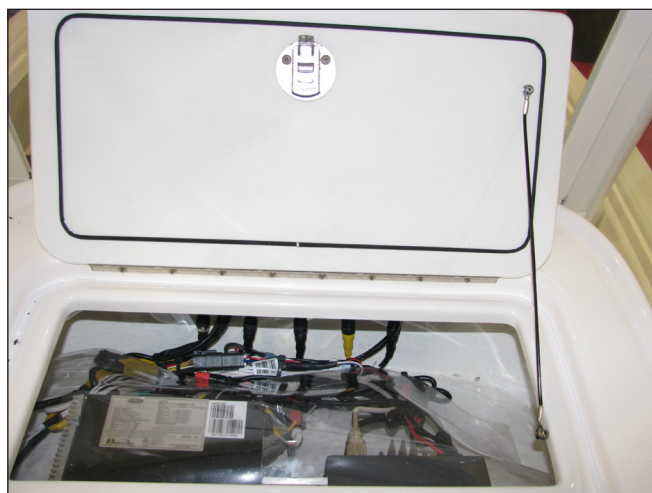
Top Step/Stand Platform Open to Service Electronics
