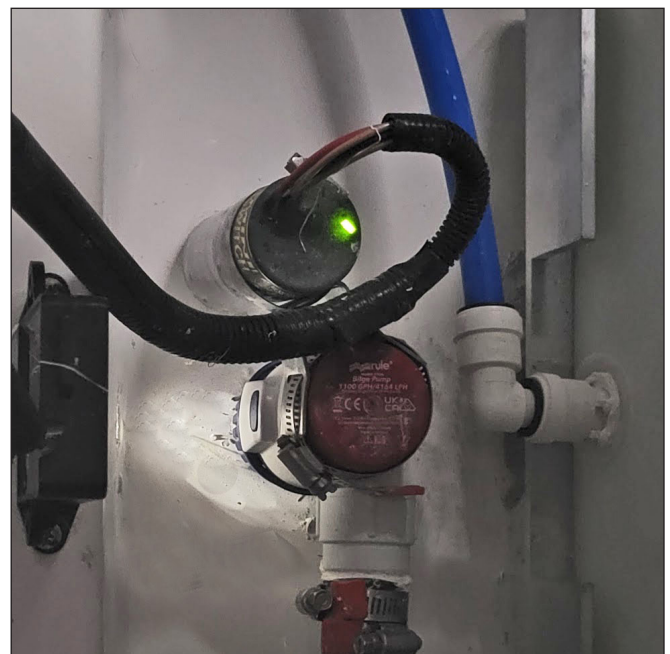
Aft Bilge Pump and Automatic Float Switch
