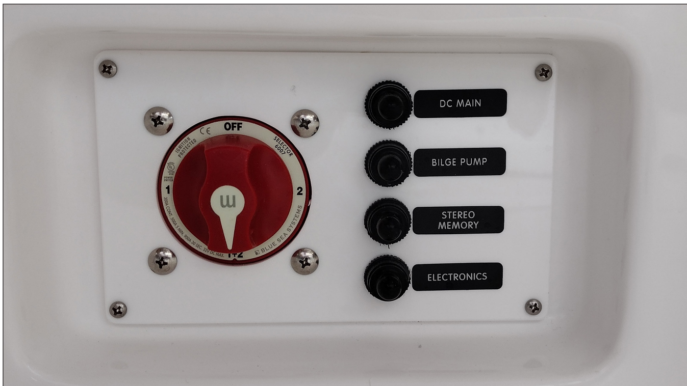
Battery Selector Switch and Circuit Breakers
