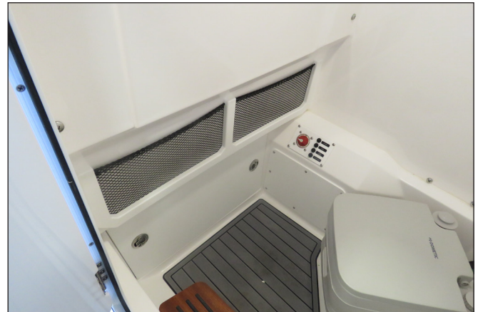
Forward Storage, Battery Compartment Access Hatch & Battery Switch Panel
