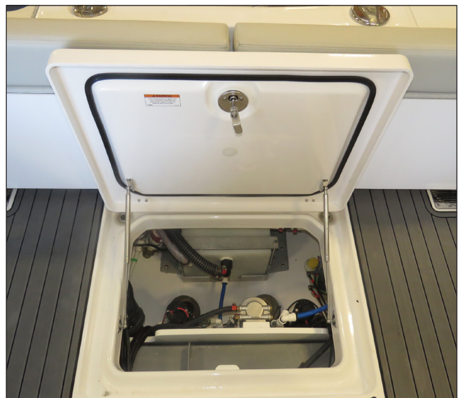
Aft Systems Access Hatch
