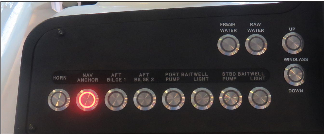
Helm Accessory Switch with Circuit Breaker Tripped
