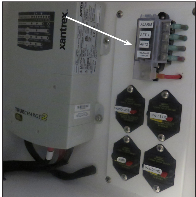
Continuous Power & Accessory Fuses Near Battery Charger
