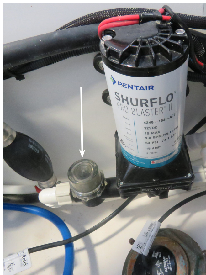
Raw Water Pressure Pump & Sea Strainer
