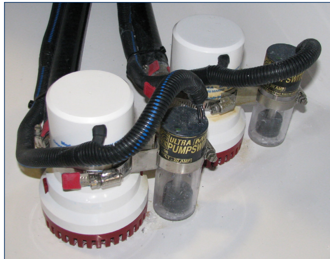
Aft Bilge Pumps & Automatic Switches
