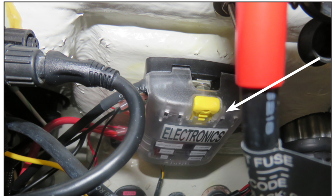
Electronics Fuse Panel Below the Helm
