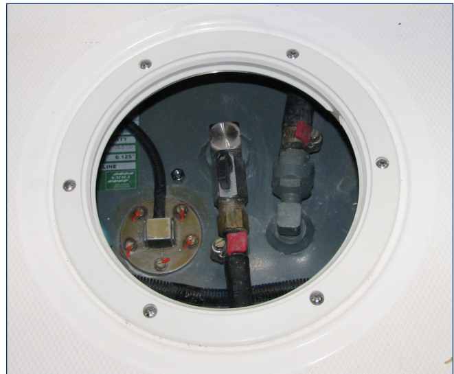
Typical Fuel Withdrawal Valves & Tank Sending Unit
