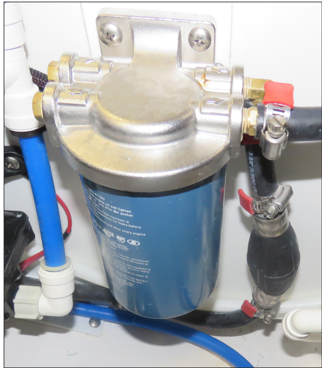
Typical Yamaha Fuel Filter In Aft Systems Compartment
