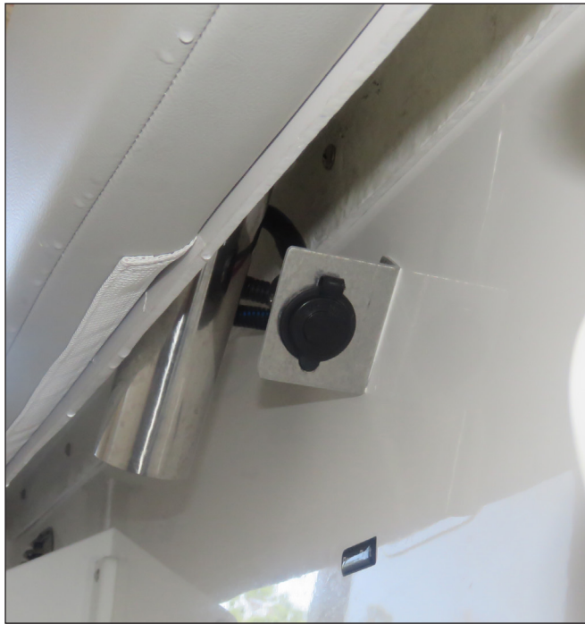
Typical Power Port
