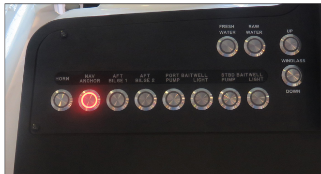
Helm Accessory Switch with Circuit Breaker Tripped
