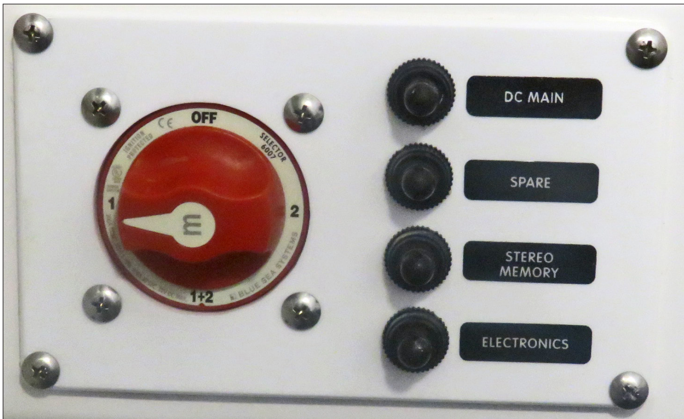
Battery Switches, Fuse Panels & Main Circuit Breakers
