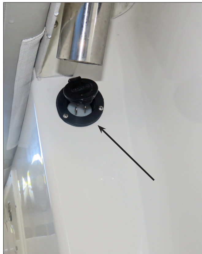
Typical 120 Volt Shore Power Inlet Connection
