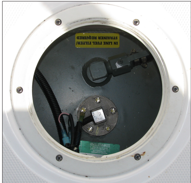
Fuel Gauge Sender and Fuel Shutoff Valve
