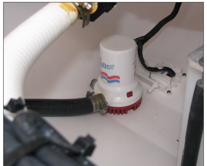
Typical Aft Bilge Pump and Automatic Float Switch
