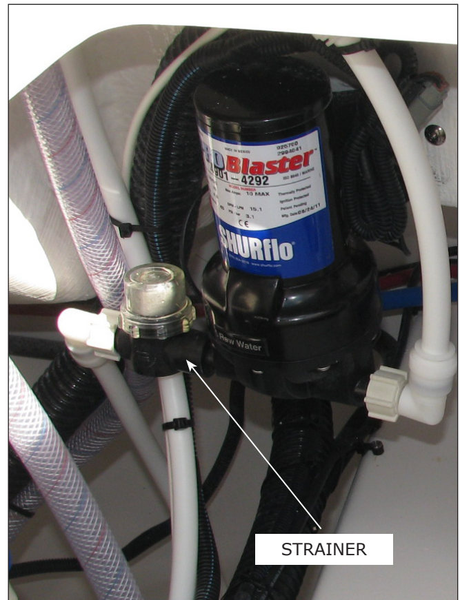
Typical Raw Water Pump and Strainer
