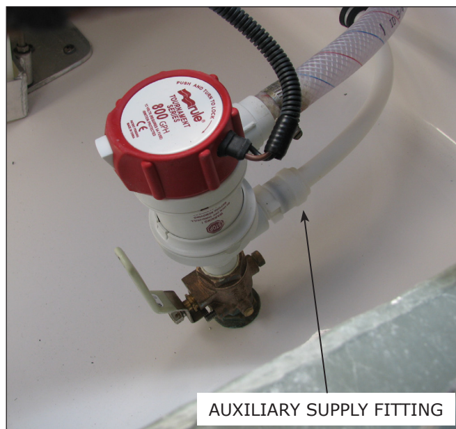
Baitwell Pump, Seacock Valve and Auxiliary Supply Connection
