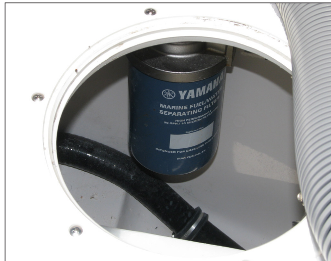
Fuel Filter Below Splashwell
