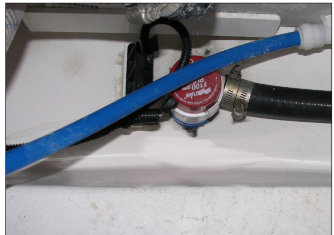
Aft Bilge Pump and Automatic Float Switch
