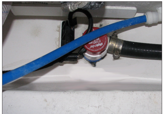
Typical Aft Bilge Pump and Automatic Float Switch
