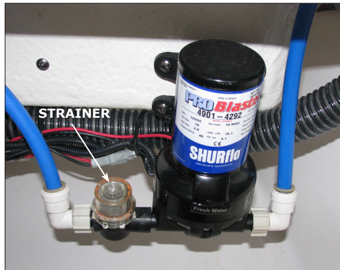
Typical Fresh Water Pump and Strainer
