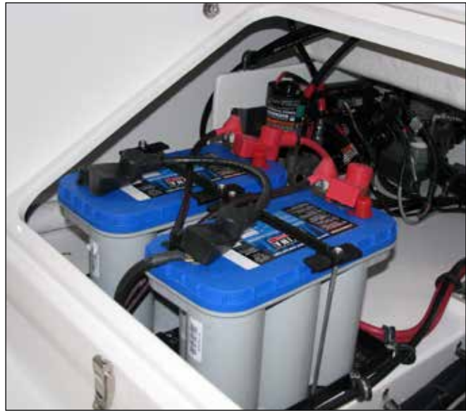
Typical AGM Batteries
