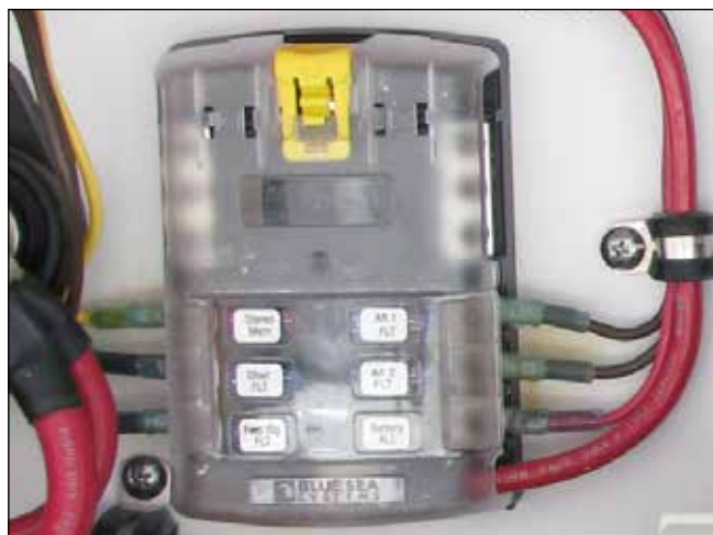
Typical Helm Accessory/Electronics Fuse Panel
