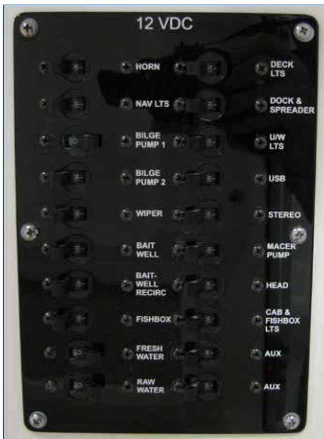
Accessory Circuit Breaker Panel In Head Compartment
