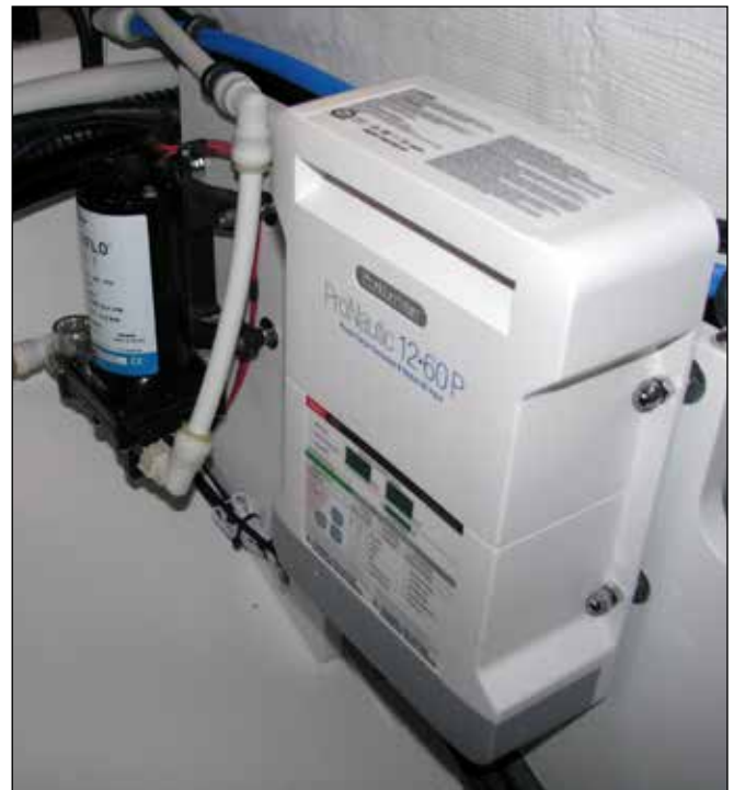
Typical Battery Charger
