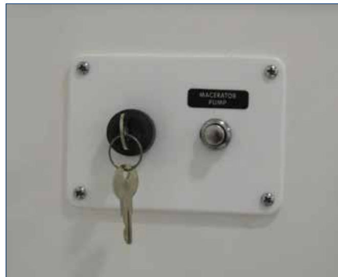
Head Compartment Macerator Pump Key Switch
