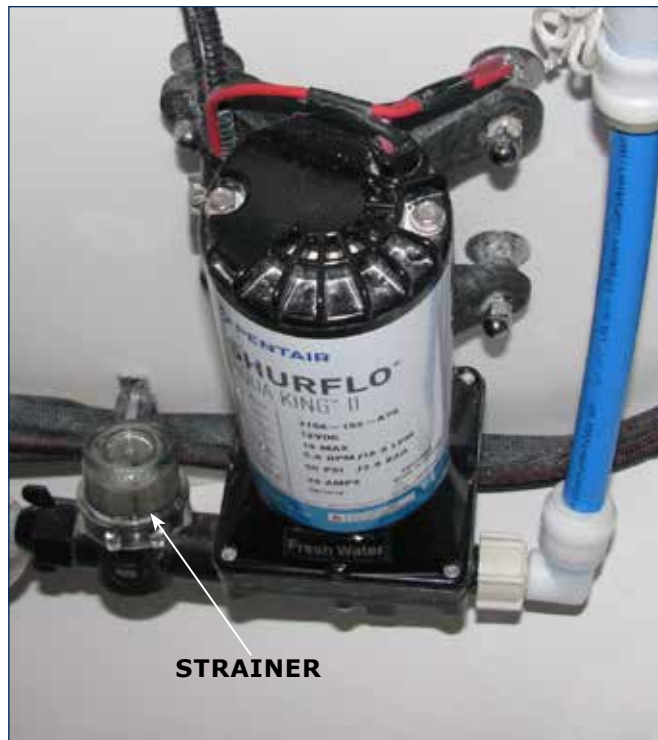
Fresh Water Pump & Strainer
