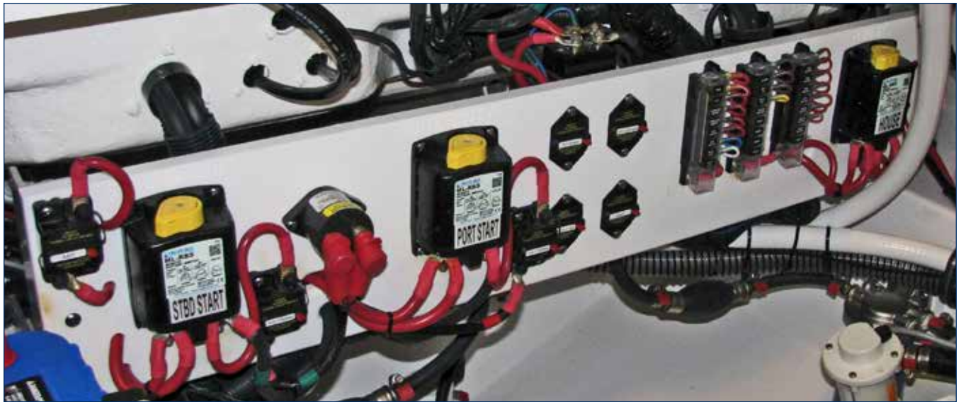
Battery Switch Panel In Aft Systems Compartment
