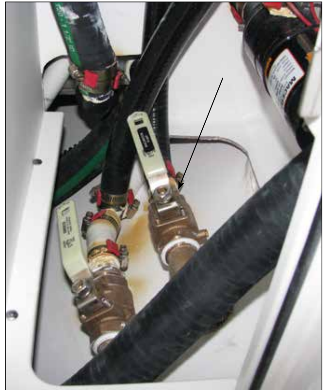
Overboard Discharge Thru-Hull Valve
