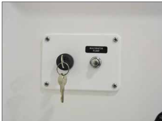
Waste System Pump Out Switch Panel
