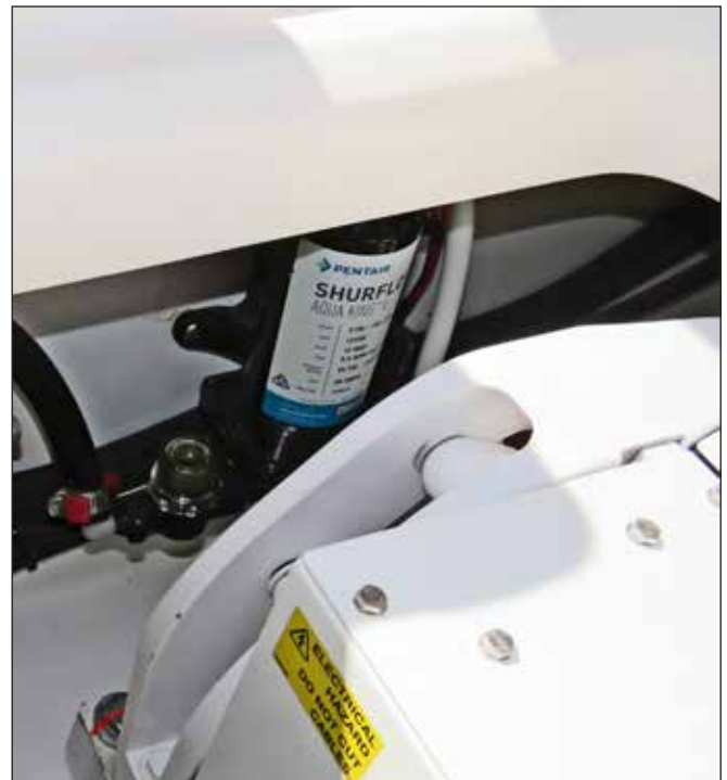
Raw Water Pressure Pump & Sea Strainer
