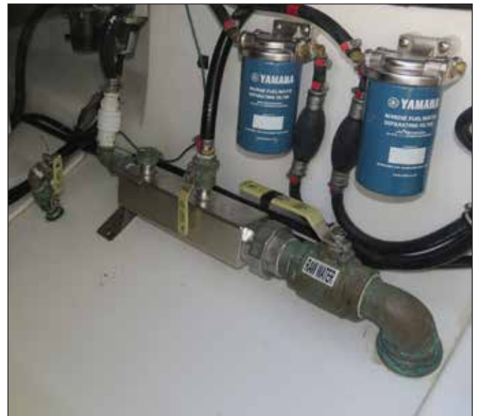
Raw Water System Manifold & Valves
