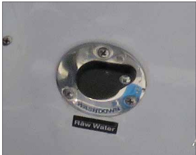
Raw Water Washdown Connection
