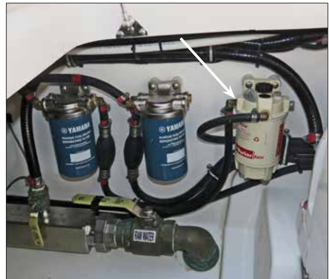
Generator Fuel Filter
