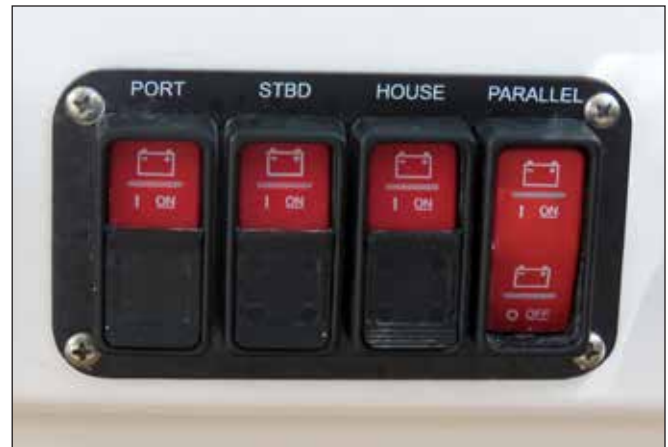
Remote Battery Switches At Helm
