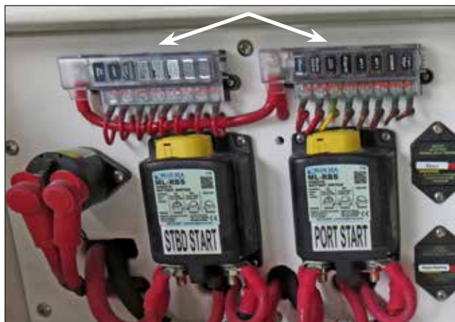
Continuous Power Fuse Panels
