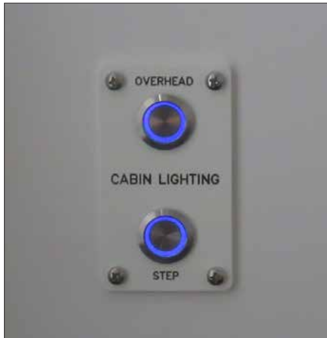
Cabin Light Switches
