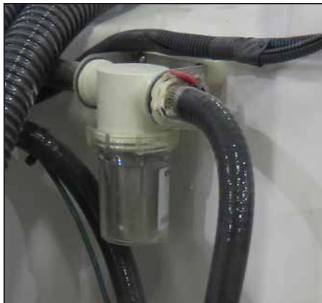
Typical Air Conditioner & SeaKeeper Pump Strainer
