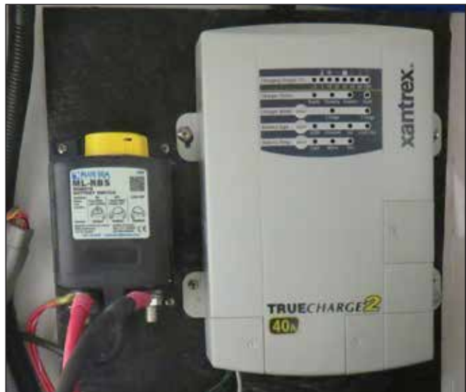
Seakeeper Battery Switch & Battery Charger
