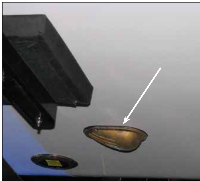
Typical Seawater Speed Scope & Strainer
