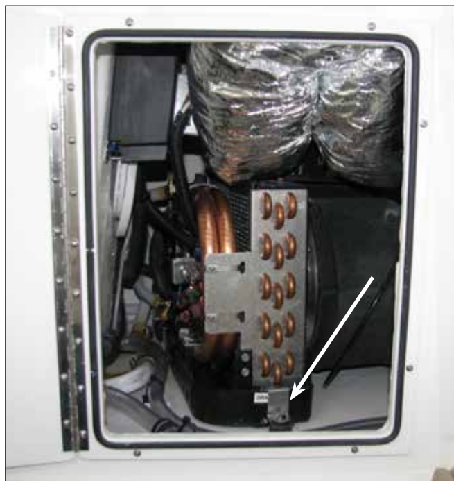
Typical Air Conditioner & Drain
