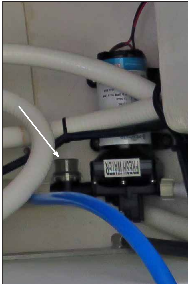
Fresh Water Pump & Strainer
