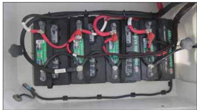
Engine & House Batteries
