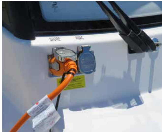
Shore Power Inlet Plugs
