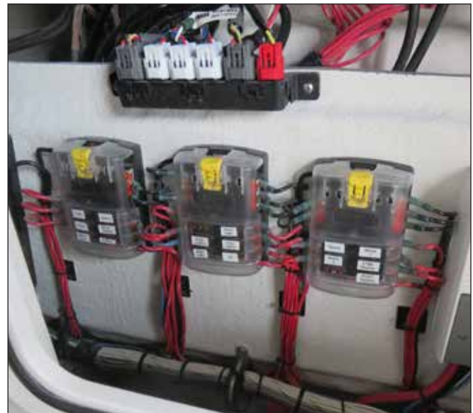
Electronics Fuse Panels Below Helm
