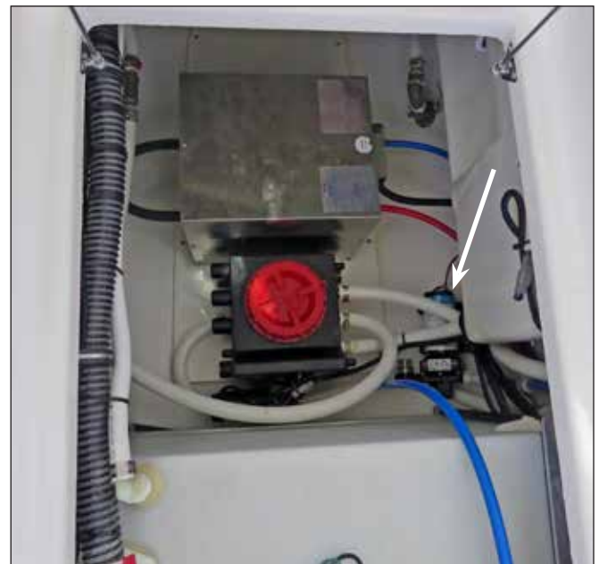
Fresh Water Pump, Drain Sump & Water Heater
