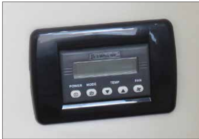
Forward Air Conditioner Control Panel
