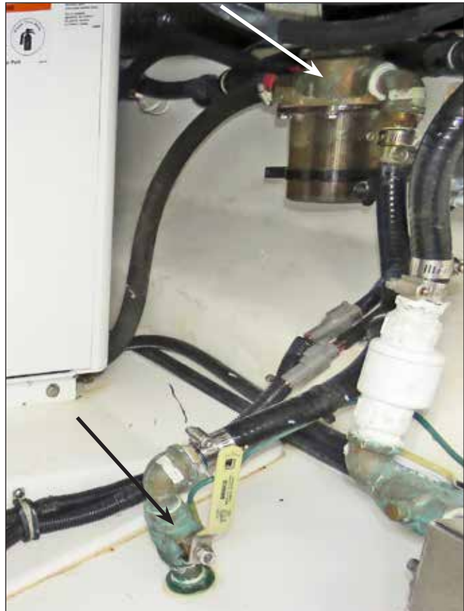
Generator Seacock Valve & Strainer
