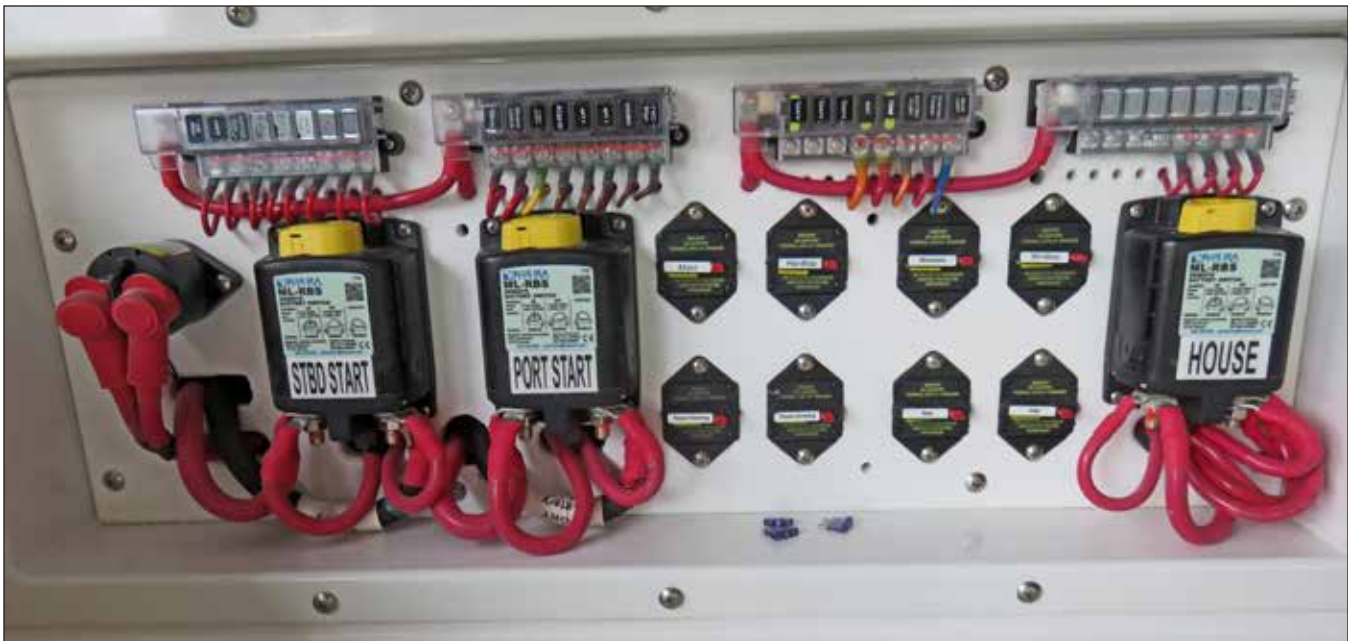
Battery Switches, Emergency Parallel Switch, Main Circuit Breakers & Fuse Panels
