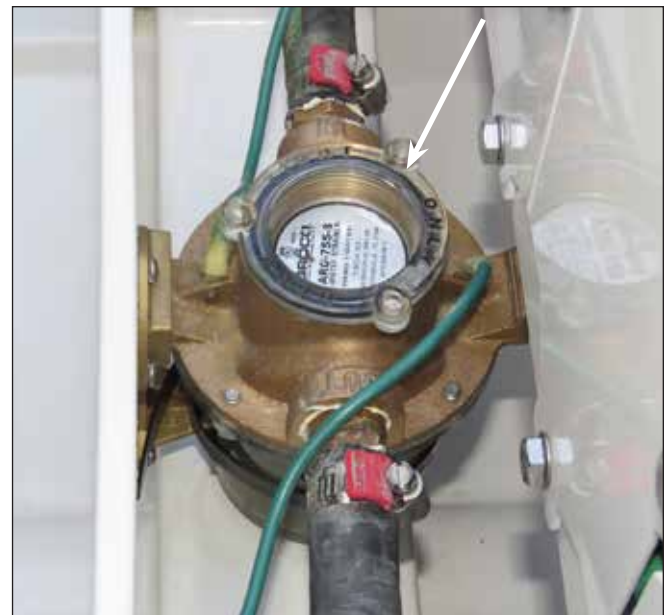
Typical Generator Sea Strainer Cap
