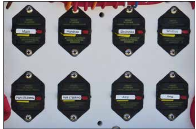
Main Circuit Breakers
