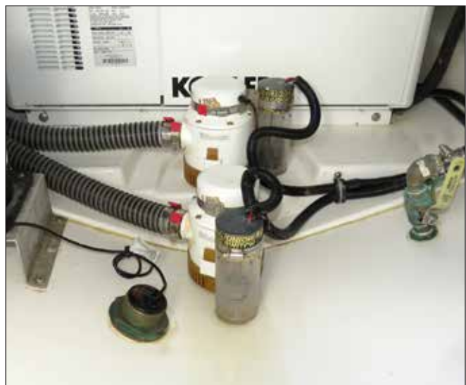
Aft Bilge Pumps & Automatic Switches
