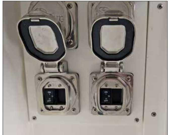
Shore Power Inlet Circuit Breakers
