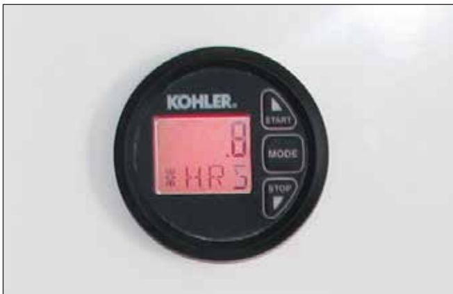
Cabin Generator Control Switch & Monitor
