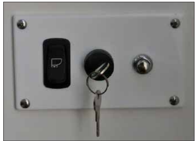
Waste Discharge Switch Panel & Marine Toilet Control Switch
