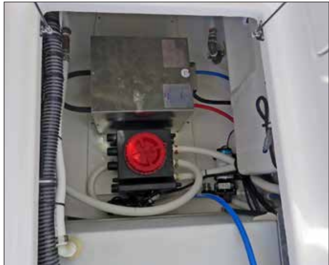
Drain Sump System
