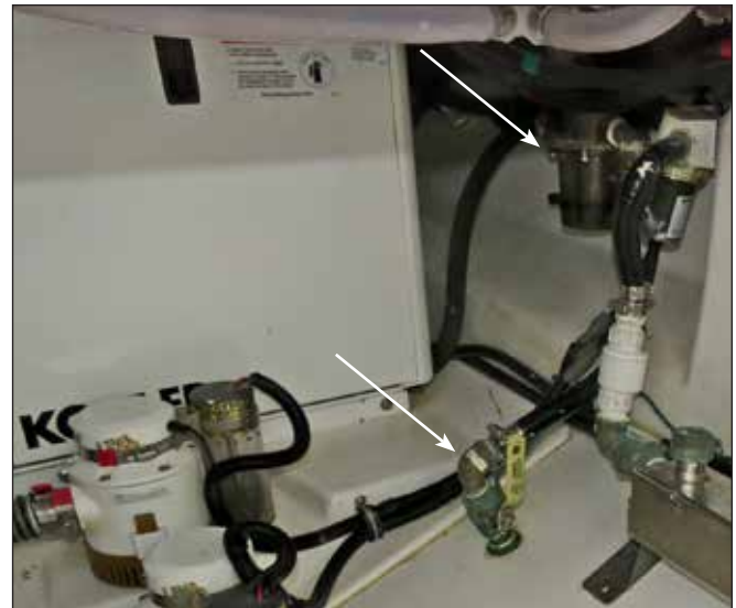
Generator Strainer & Seacock
