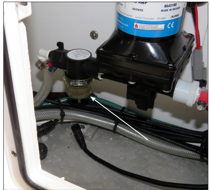
Seakeeper System Sea Strainer
