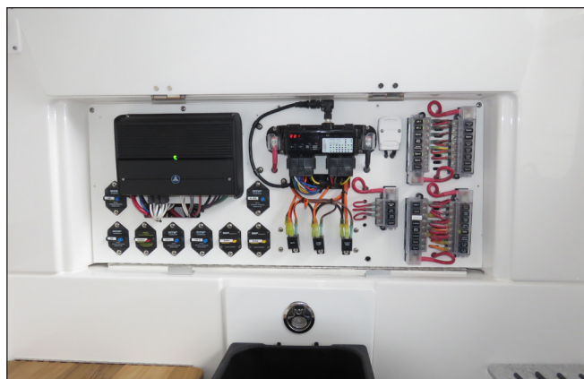
Electrical Systems Compartment Behind Lower Access Door
