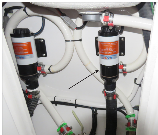
Waste Overboard Discharge Pump
