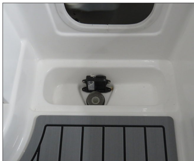
Head Compartment Sump System
