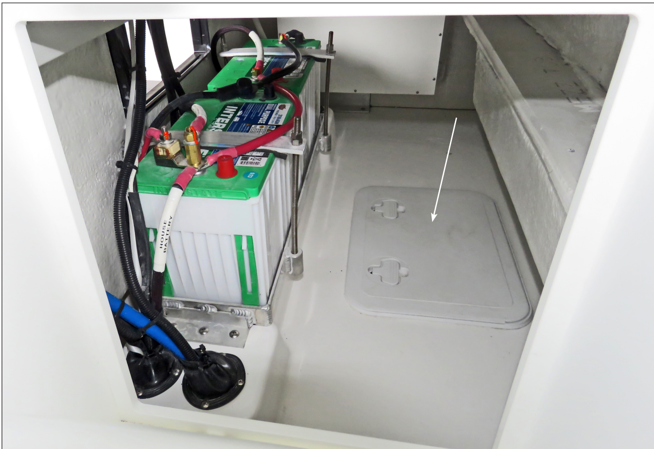
Fuel Valves & Fuel Gauge Sender Access Hatch In The Cockpit Sole Below The Mezzanine Seats Or Workstation
