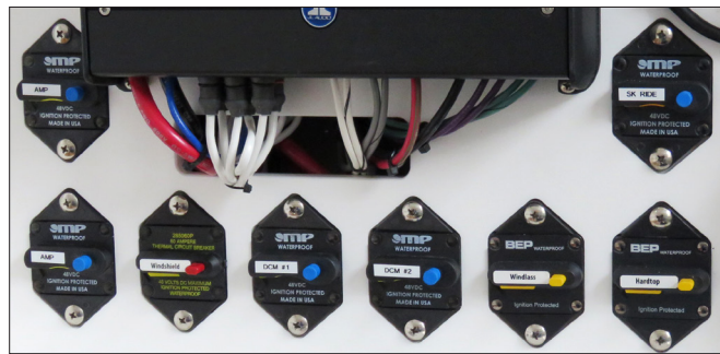
Main Circuit Breakers Behind Access Door In Head Compartment
