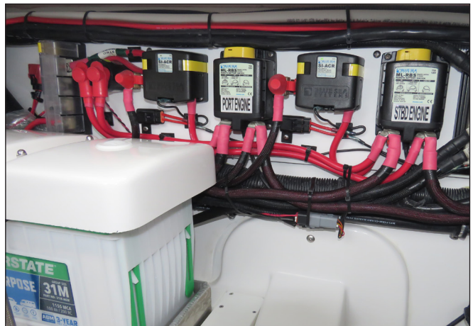
Engine Battery Switches & Automatic Charging Relays In Aft Systems Compartment
