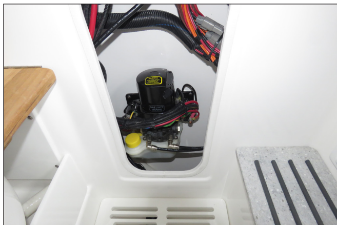
Windshield Hydraulic Pump Behind Basket Hatch
