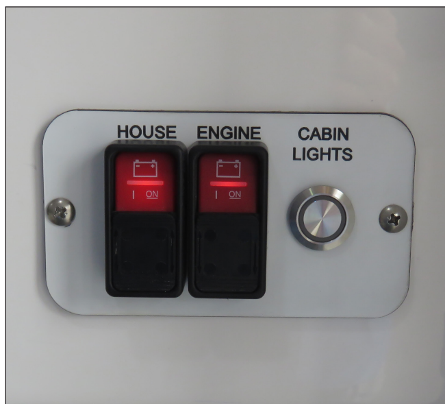
Battery Switches On Panel In Head Compartment
