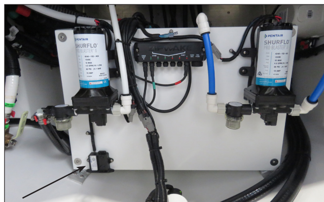
High Water Alarm Automatic Switch
