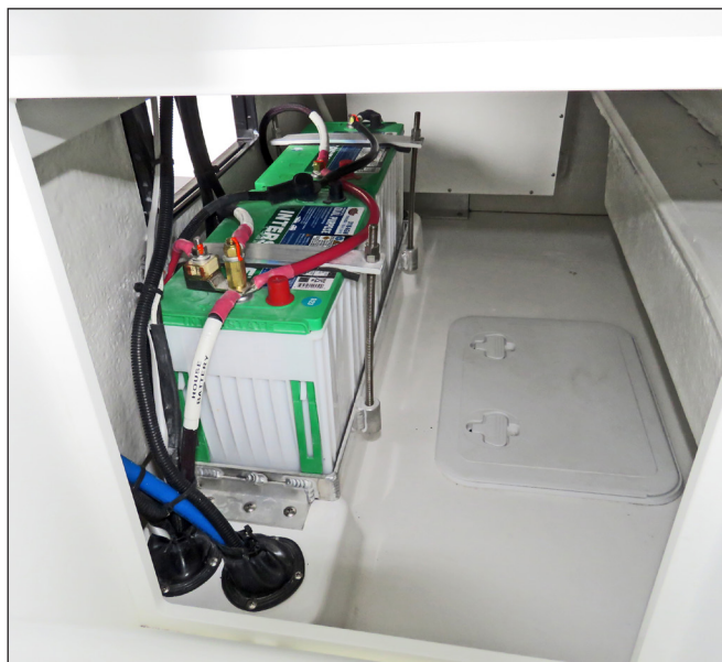
House Batteries & Fuel Tank Components Access Panel
