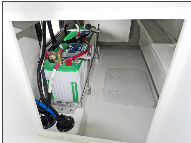
House Batteries In Compartment Below Helm Seats
