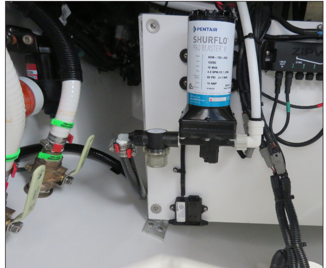
Raw Water Pressure Pump & Sea Strainer
