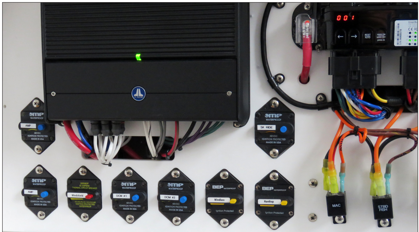
Main Circuit Breakers Located Behind Access Door in Head Compartment
