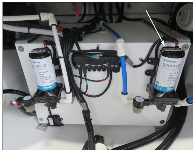
Fresh Water Pump
