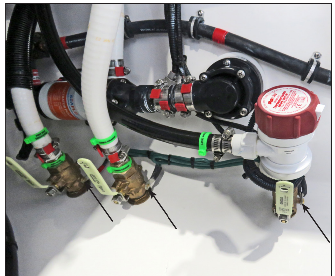
Typical Bonding Wires & Connections
