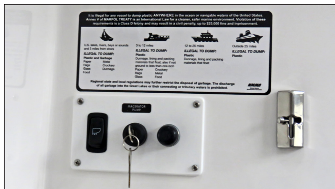
Toilet Fill/Flush Switch, Key Activated Lockout Switch & Macerator Discharge Pump Switch
