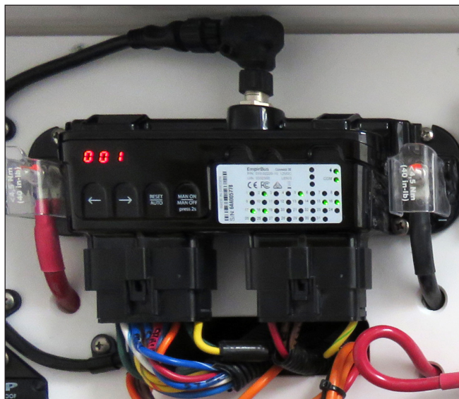
Digital Switching Control Module Circuit Breaker Reset & Manual Override Switches
