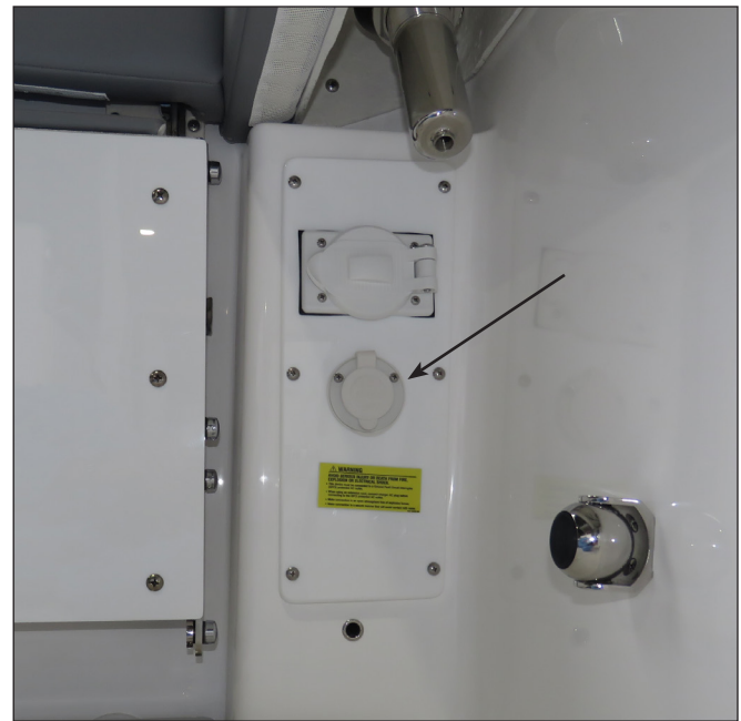
Shore Power Cable Inlet Connection
