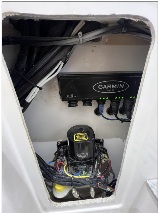
Typical Windshield Hydraulic Pump Behind Removable Access Panel In Aft Head Compartment Bulkhead
