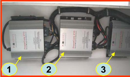
Power Management Enclosures
