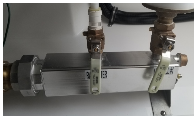
Raw Water System Manifold & Valves
