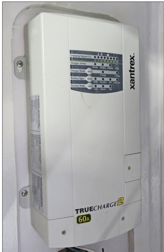
Typical Battery Charger
