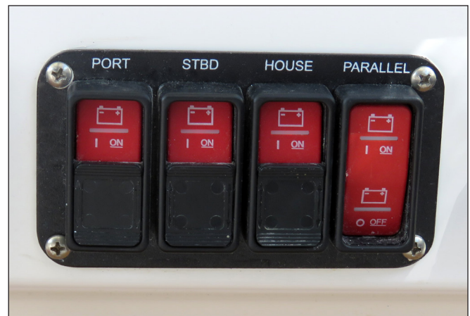
Remote Battery Switches At Helm
