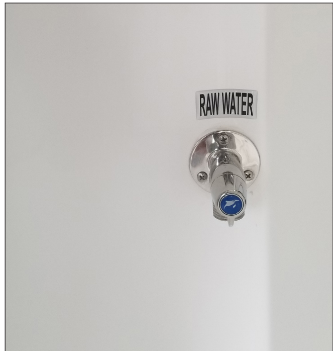
Raw Water Washdown Connection
