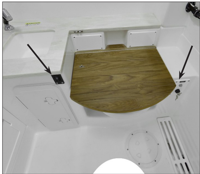
Waste Discharge Switch Panel & Marine Toilet Control Switch
