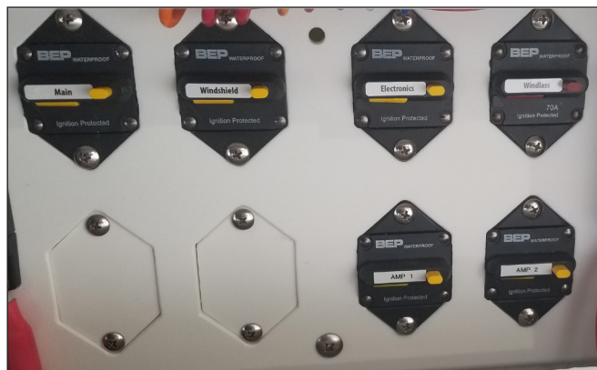
Main Circuit Breakers
