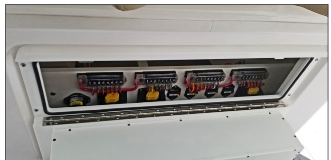
Battery Switch Access Door/Storage Compartment Open
