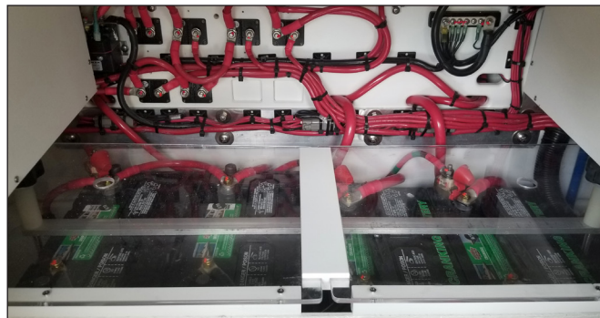
Engine & House Batteries
