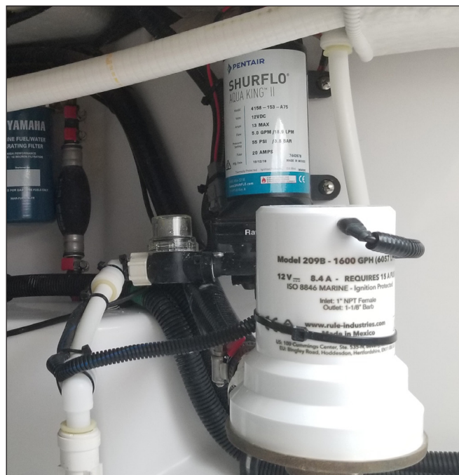
Raw Water Pressure Pump & Baitwell Pump
