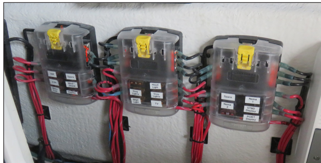
Typical Electronics Fuse Panels Below Helm
