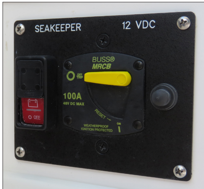
SeaKeeper Battery Switch & Circuit Breaker Panel
