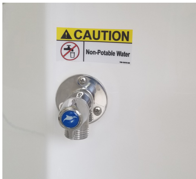
Fresh Water Washdown
