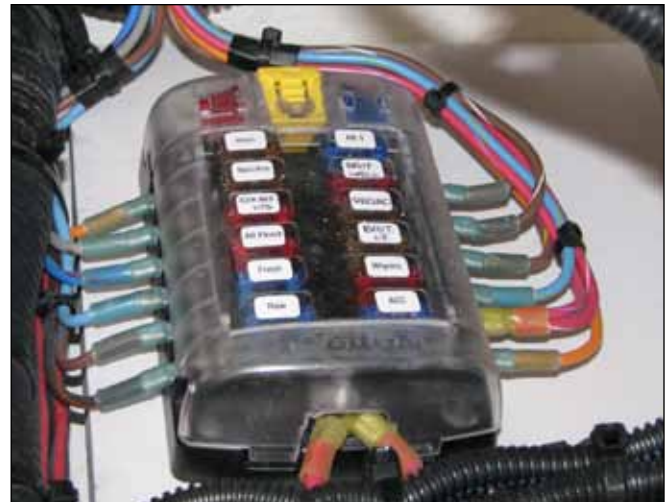
Accessory Fuse Panel Behind Helm
