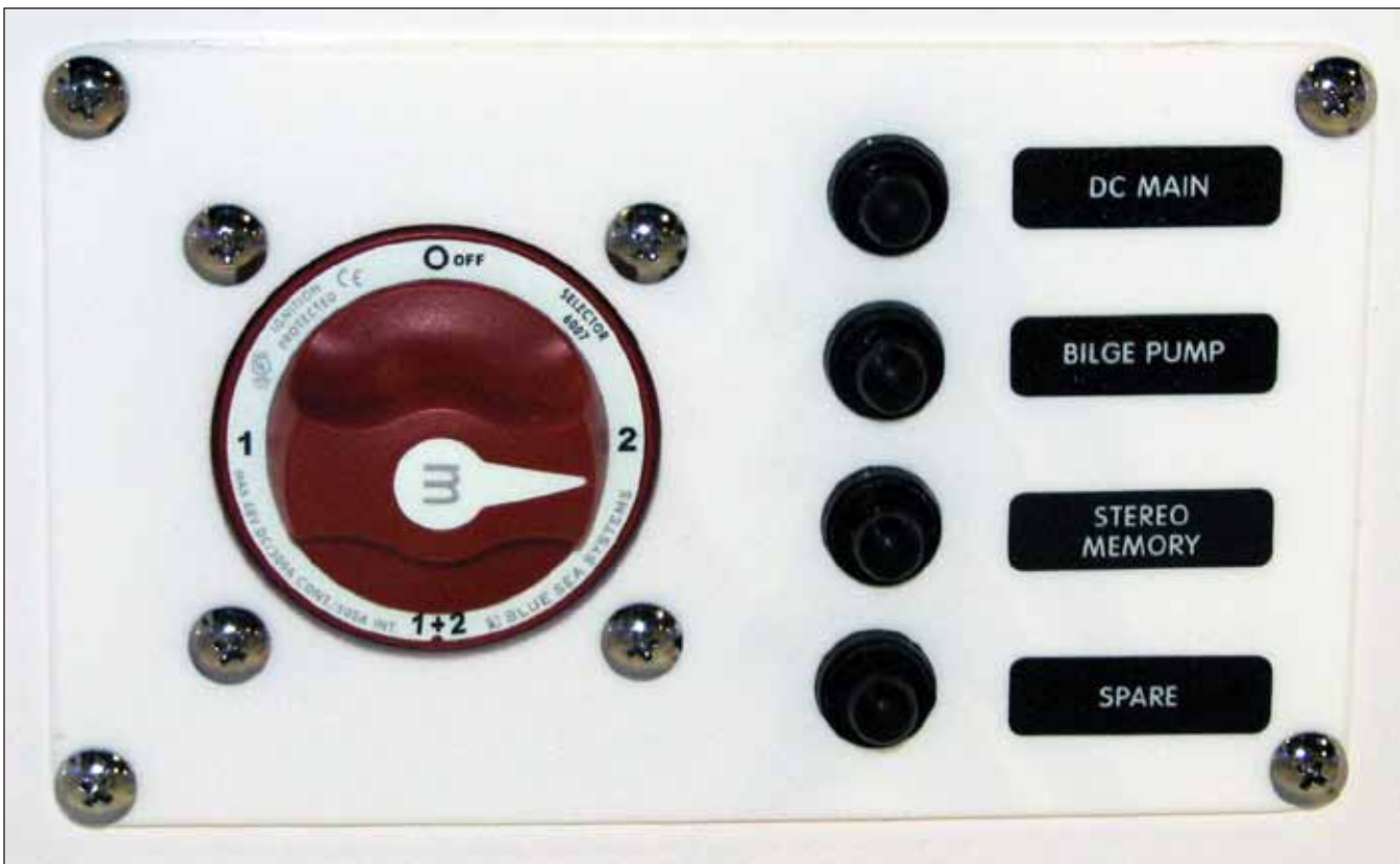
Battery Selector Switch and Circuit Breakers
