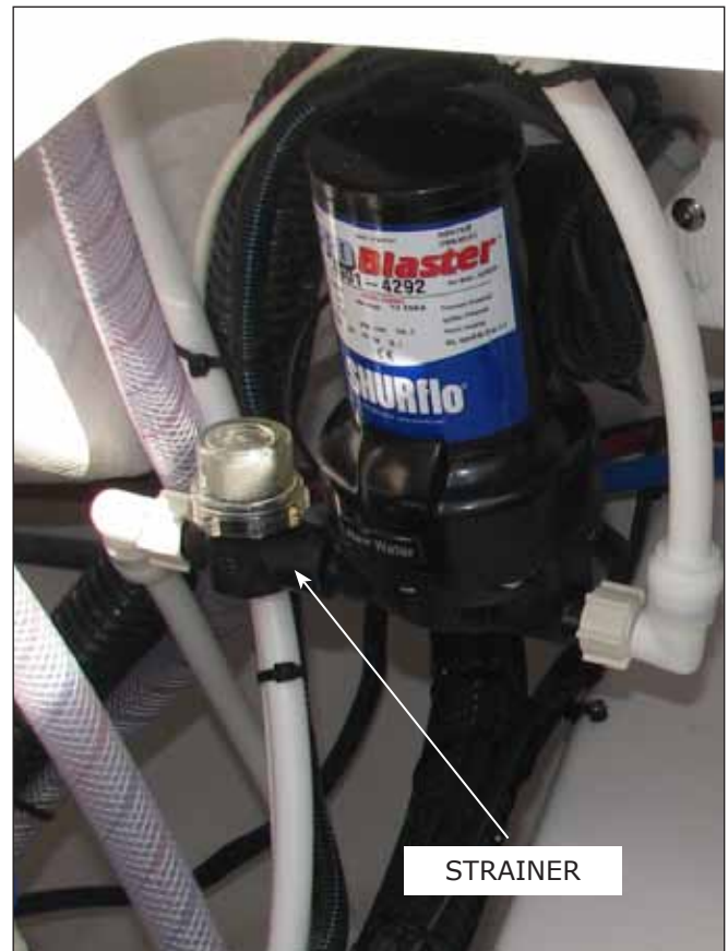
Typical Raw Water Pump and Strainer
