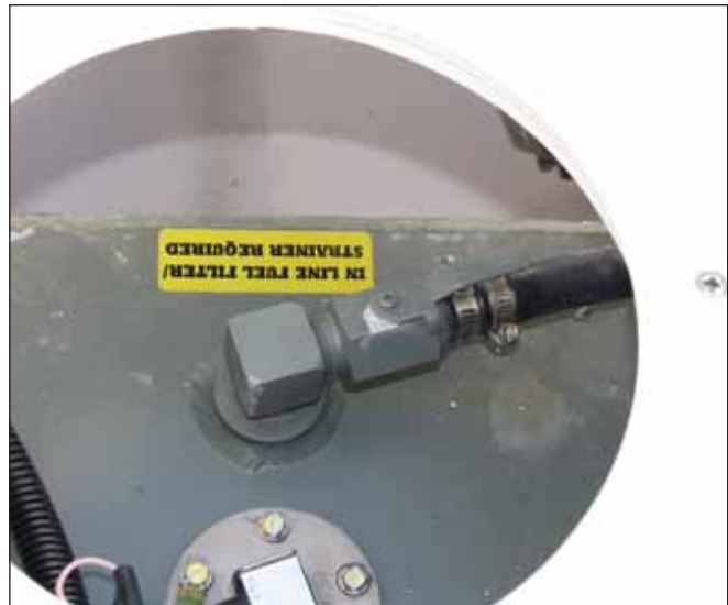
Typical Fuel Shutoff Valve
