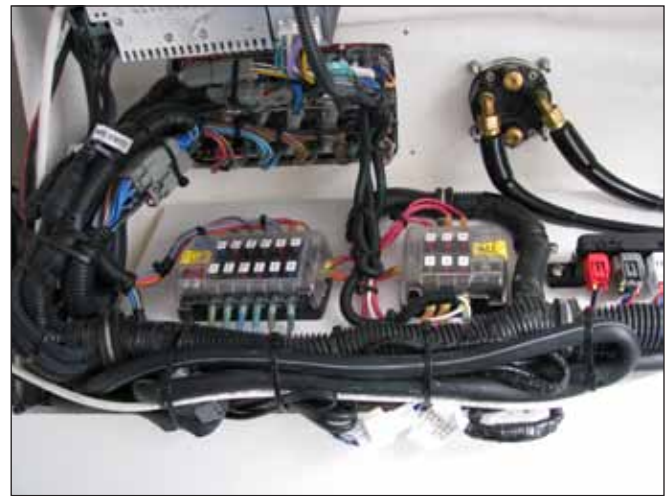
Fuse Panels Located Behind Helm
