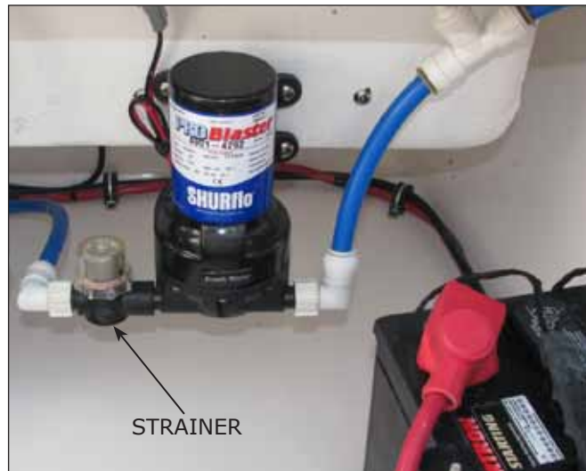
Typical Fresh Water Pump and Strainer
