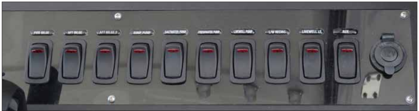
Starboard Helm Accessory Switch Panel
