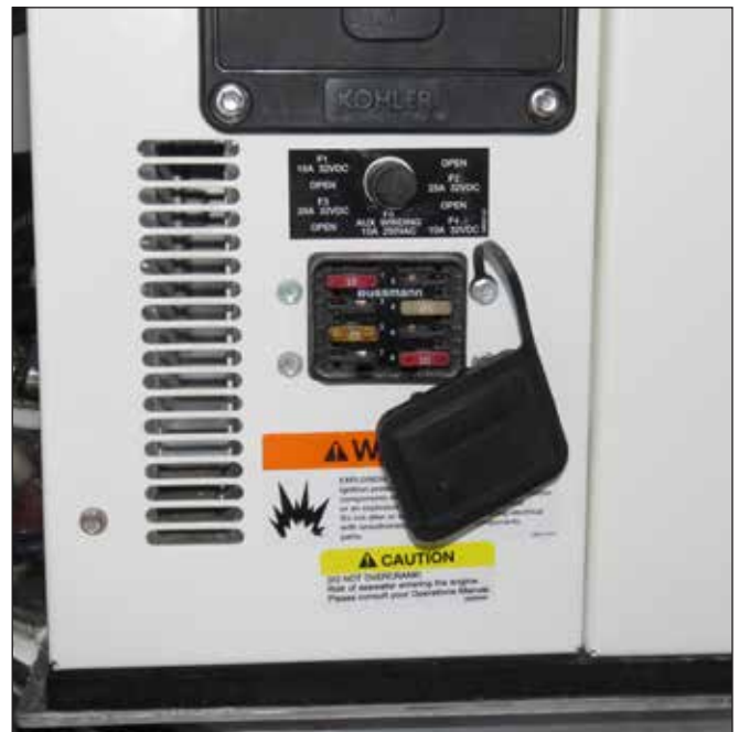
Typical Generator Fuse Panel
