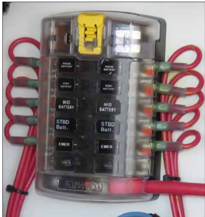
Remote Battery Switch Fuse Panel
