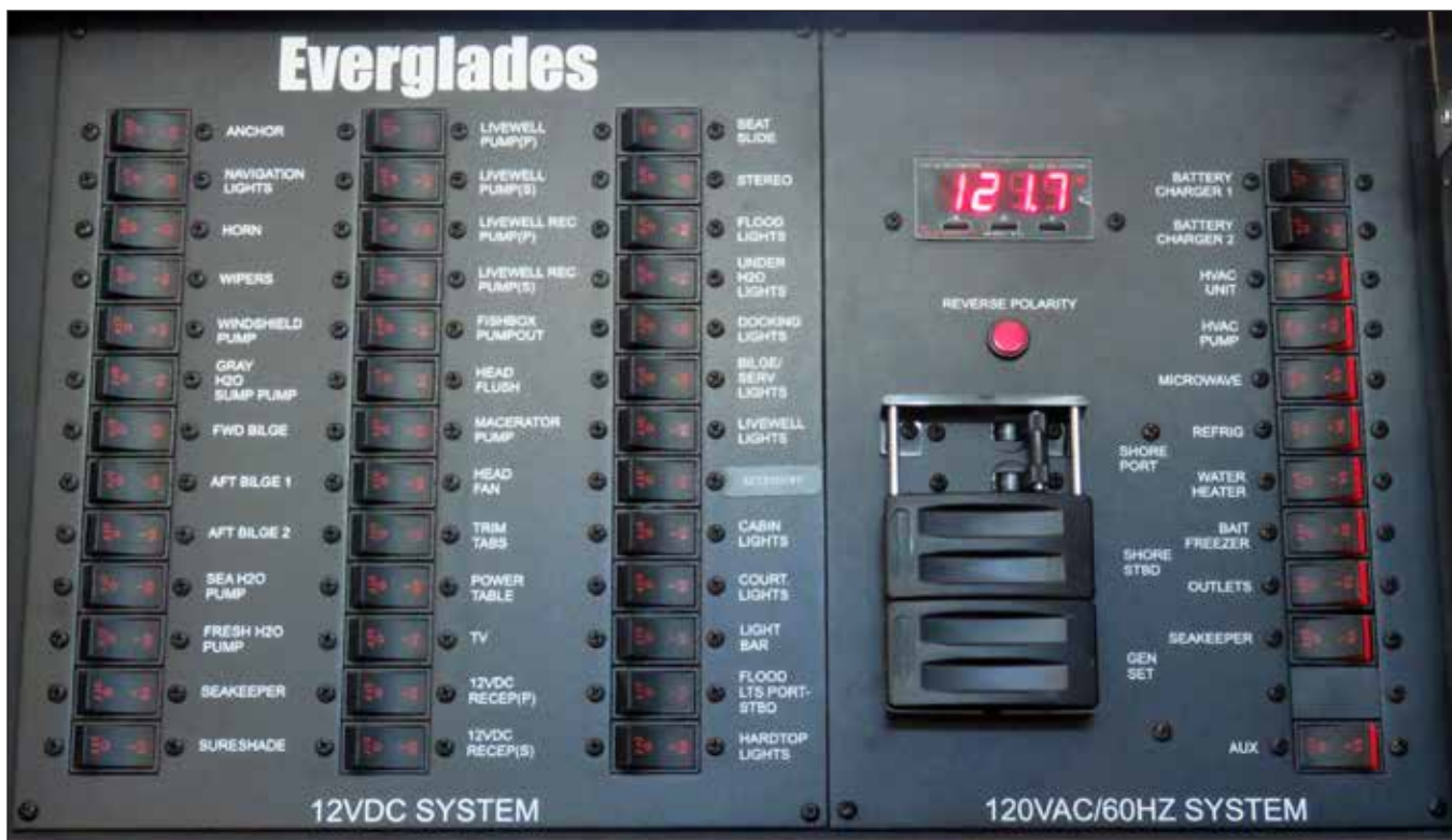
Cabin DC/AC Panel
