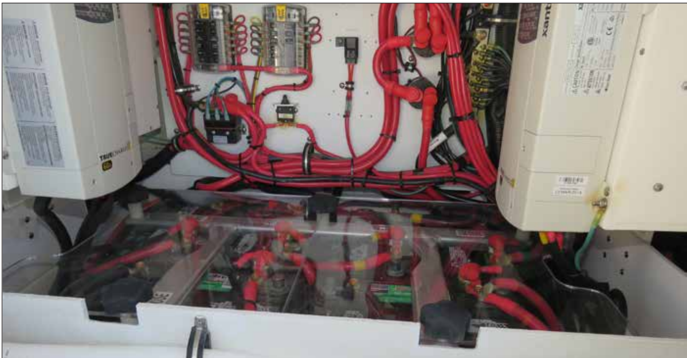
Batteries In Electrical Systems Compartment
