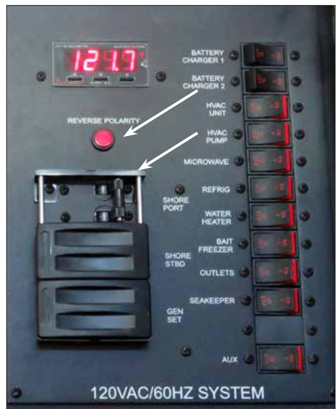
Reversed Polarity Light & Shore PWR/Generator Main Breakers
