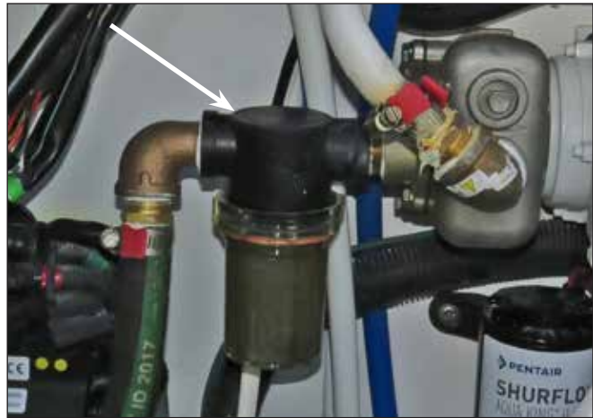
HVAC Pump Sea Strainer
