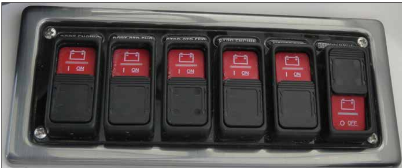
Battery Switch Panel at Helm
