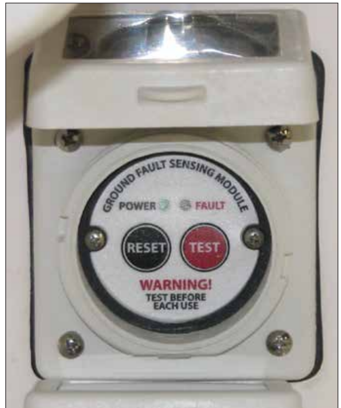
Typical ELCI Panel
