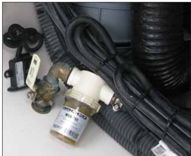
Typical Generator Raw Water Seacock & Strainer
