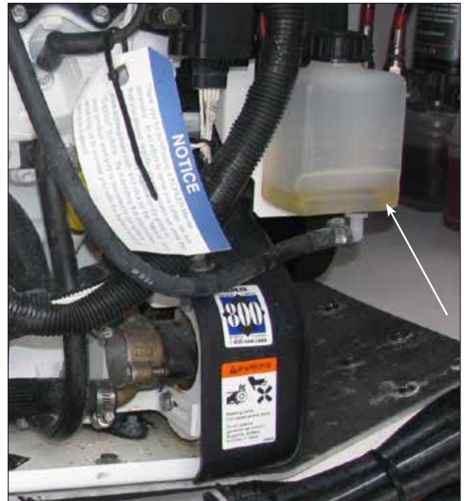
Typical Generator Coolant Recovery Tank
