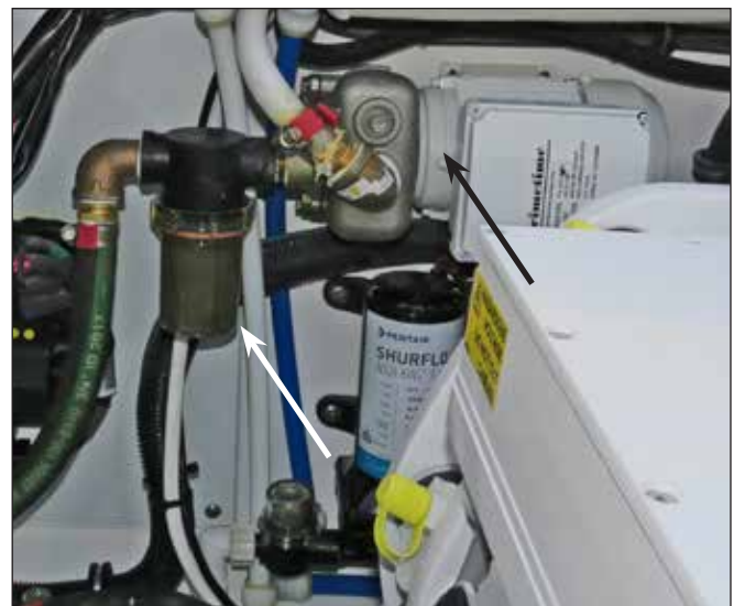
Air Conditioner Seawater Pump & Strainer
