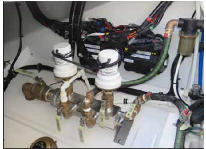
Raw Water Manifold, Port & Starboard Livewell Pumps, Raw Water Pump Connection, HVAC Pump Connection & Ball Valves
