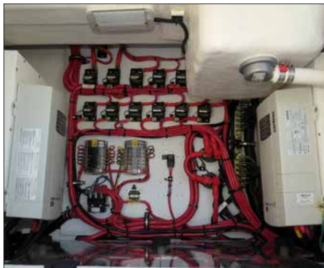
Main Circuit Breakers, Fuse Panels & Battery Chargers
