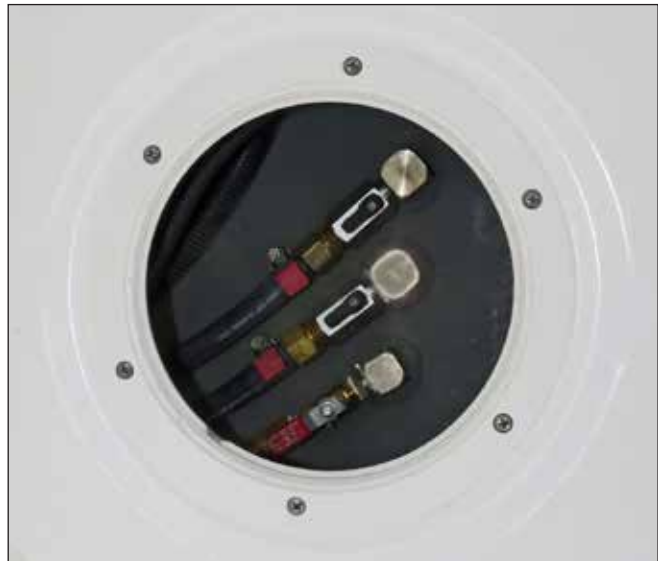
Typical Fuel Withdrawal Valves
