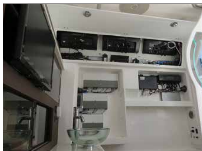
Electronics Access in Rear Cabin Bulkhead
