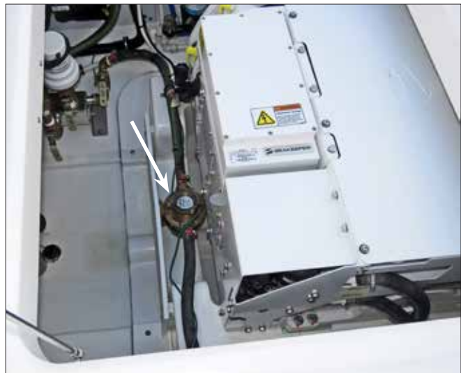
SeaKeeper System Sea Strainer
