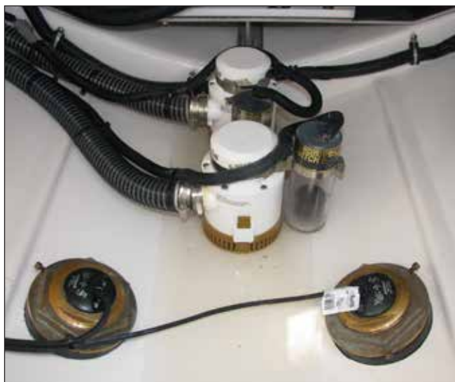
typical Stern Bilge Pumps & Automatic Switches
