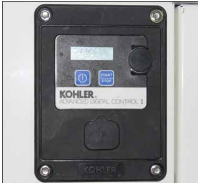
Generator Onboard Control Switch & Engine Monitor,
