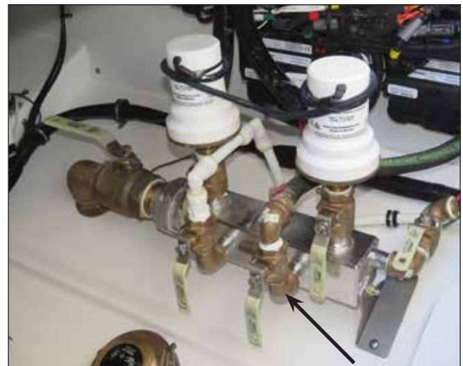
Air Conditioner Pump Supply Valve
