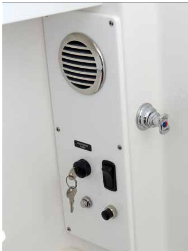
Head Switch Panel & Shower Control Valve
